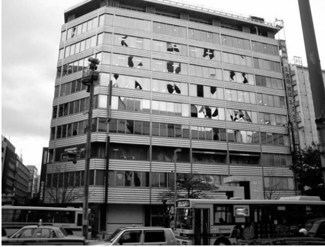
Fig. 8-3. Glass breakage in strip window system during Fukuoka (Japan) (magnitude 7.0) earthquake of March 20, 2005 Source: http://en.wikipedia.org/wiki/File:Fukuoka_Earthquake_20050320_Maruzen.jpg
