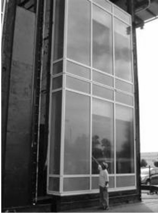
Fig. 4-3. Example of an installed two-story mockup for testing Source: Courtesy of Construction Consulting International; reproduced with permission
