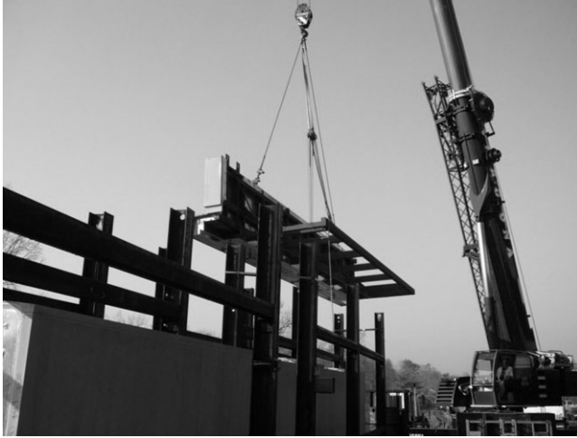
Fig. 3-9. Stone truss panel being hoisted from transportation vehicle; note the steel frame back-up behind the stone panels
