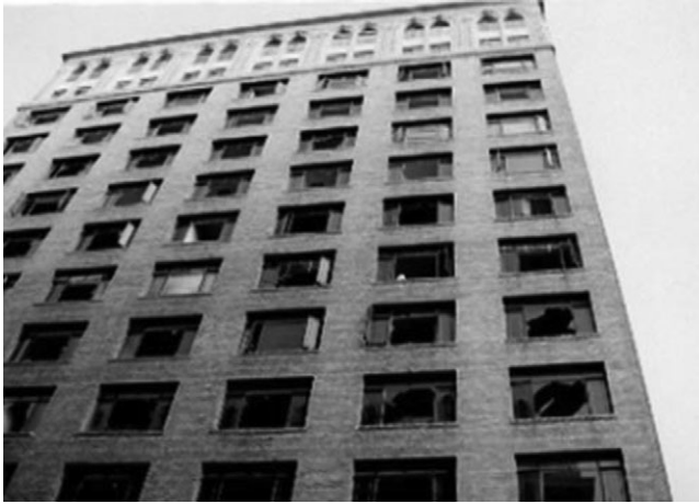
Fig. 8-1. Glass breakage in punched window system during Loma Prieta (magnitude 6.9) earthquake of October 17, 1989
