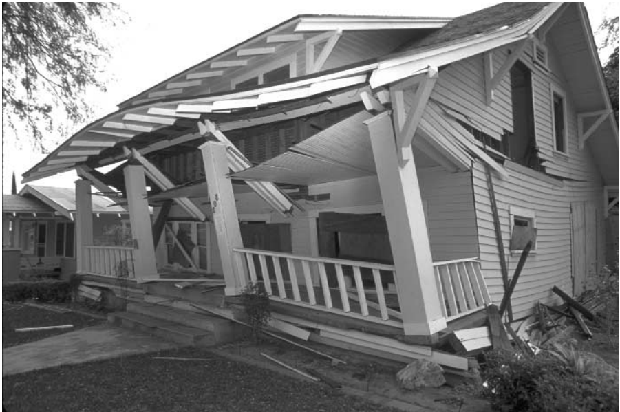
Figure 2-2 Northridge Earthquake, California, January 17, 1994. Buildings, cars, and personal property all were destroyed when the earthquake struck. Approximately 114,000 residential and commercial structures were damaged and 72 deaths were attributed to the earthquake. Damage costs were estimated at $25 billion. FEMA News Photo.
