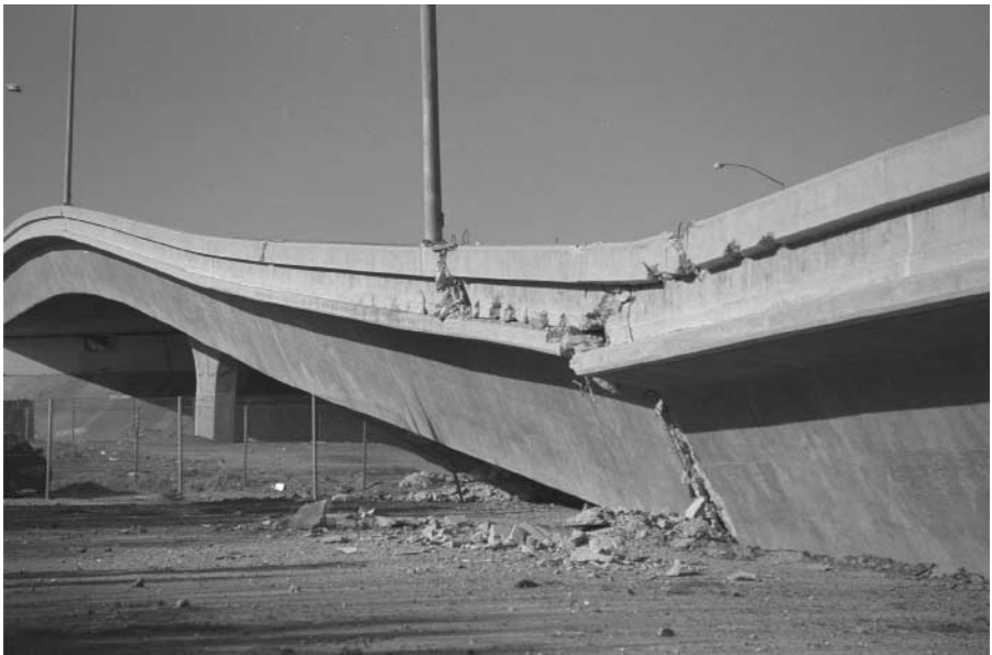
Figure 1-2 Northridge Earthquake, CA, January 17, 1994. Many roads, including bridges and elevated highways, were damaged by the 6.7 magnitude earthquake. Approximately 114,000 residential and commercial structures were damaged and 72 deaths were attributed to the earthquake. Damage costs were estimated at $25 billion. FEMA News Photo.
