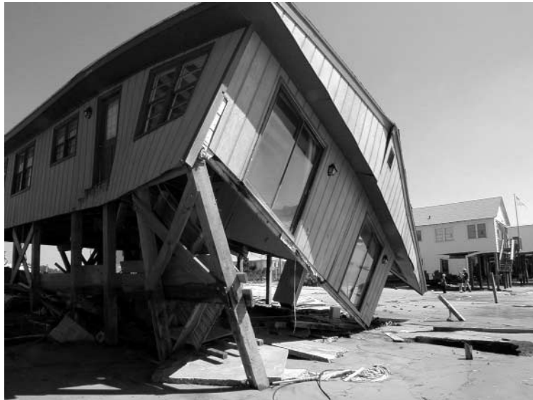
Figure 5-2 South-facing Long Beach on Oak Island, North Carolina, September 17, 1999. Hurricane Floyd brought a devastating 15 feet of storm surge that damaged or destroyed hundreds of houses along this community's oceanfront and flattened its frontal sand dunes. Here, even elevation failed to save this home. Additional strapping, upgraded mitigation work, might have helped. Photo by Dave Gattley/FEMA News Photo.
