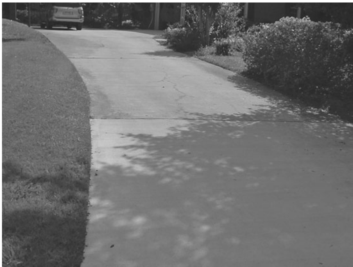
FIGURE 2.7.2 Example of weathered and new concrete pavement surfaces in Columbia, S.C. The weathered surface is approximately 15 years old, and the new surface is less than a month old.
