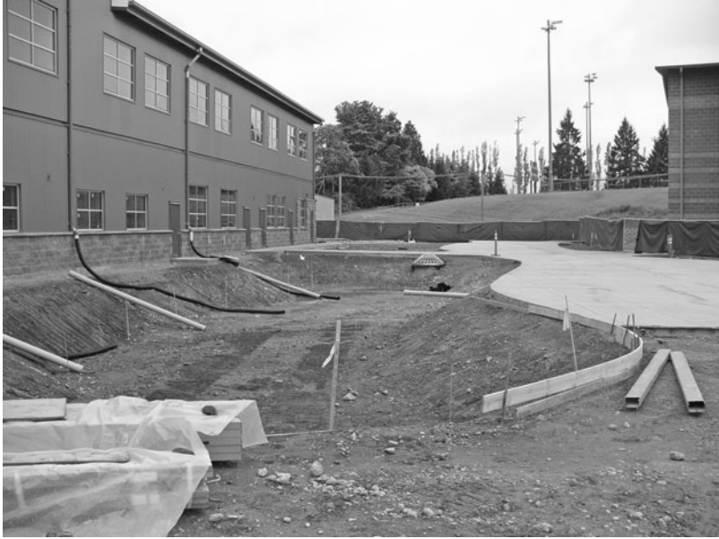
FIGURE 10.2.4 Roof stormwater leaders directed into a rain garden under construction at Bothell High School in Washington. (Photograph courtesy Coughlin Porter Lundeen taken September 2008.)
