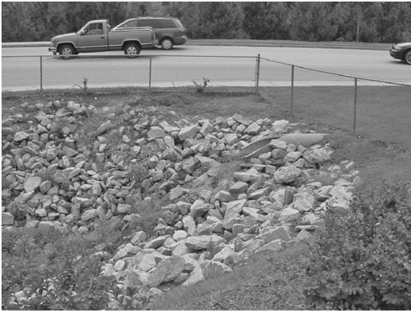
FIGURE 10.1.4 Detention pond with riprap erosion control around the inlets and banks in Irmo, S.C. (Photograph taken July 2007.)
