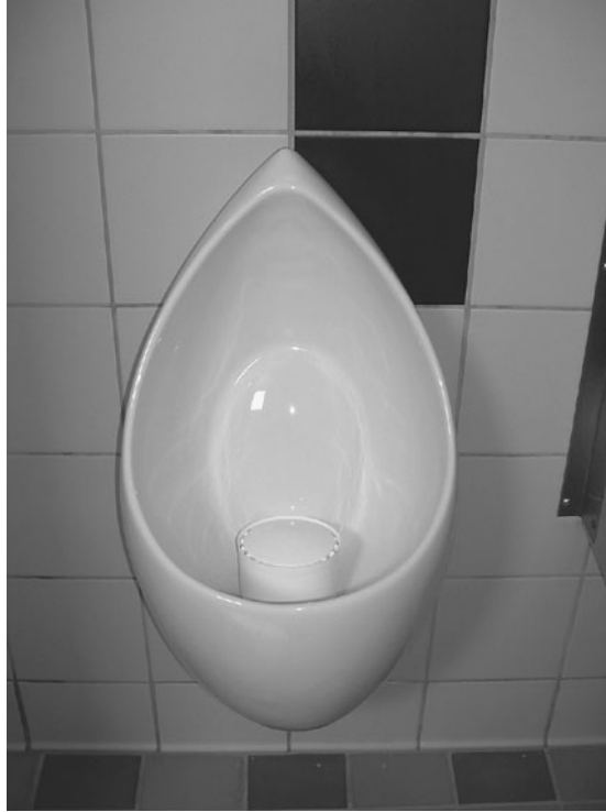
FIGURE 3.2.1 Waterless urinal installed in the LEED certified public health building at the University of South Carolina, Columbia, S.C. (Photograph taken July 25, 2007.)
