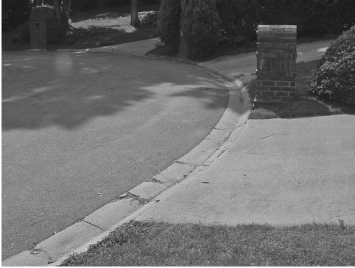
FIGURE 2.7.1 Example of weathered concrete and asphalt pavement surfaces in Columbia, S.C. The pavements are approximately 15 years old.
