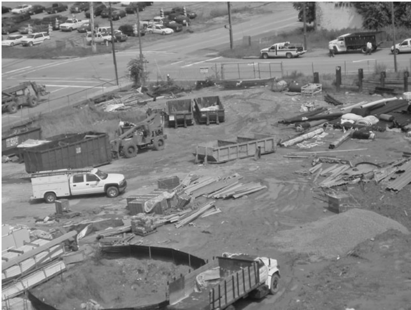
FIGURE 1.1.1 Construction debris container yard at a LEED-registered project in 2005 at the University of South Carolina in Columbia, S.C. (Photograph taken by Steve Bruner.)
