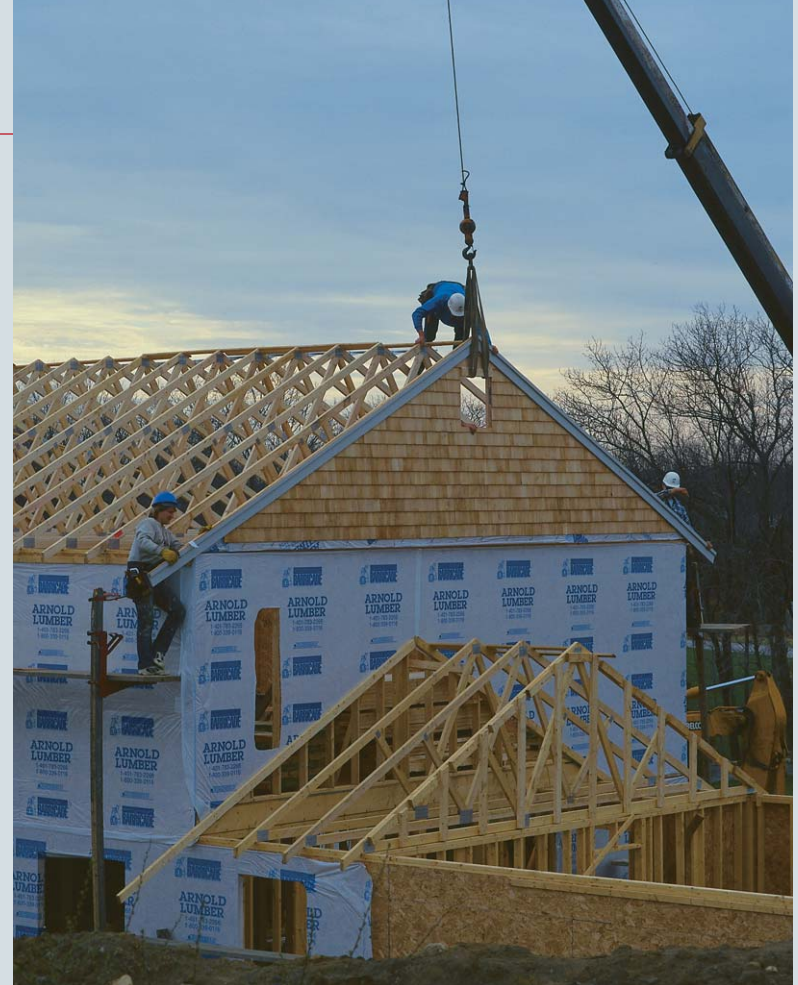
Factory-fabricated roof trusses have made framing a roof much easier and faster, but they have also eliminated attic space in the majority of new homes.
