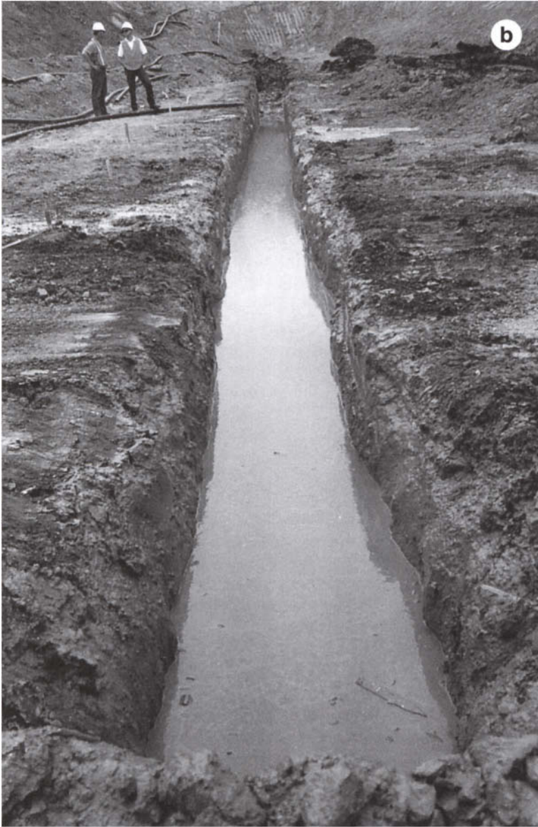
Figure 7 Permeable reactive barrier and slurry wall construction near Monticello, Utah, (June 1999), (a) Open trench before reactive materials were emplaced, (b) Bentonite slurry in the trench for the south slurry wall.
