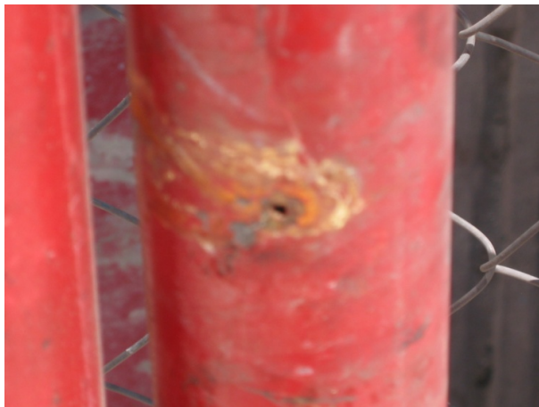
Figure 2. External pitting caused by biocorrosion on the internal surface of a carbon steel pipe in a fire extinguisher system.
