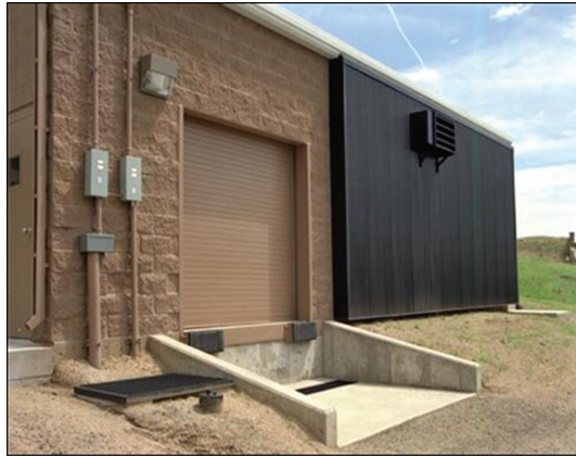
Figure 7.11. Photograph of transpired solar collector and bypass damper of solar ventilation air preheat system on NREL chemical storage building (photo by the author).
