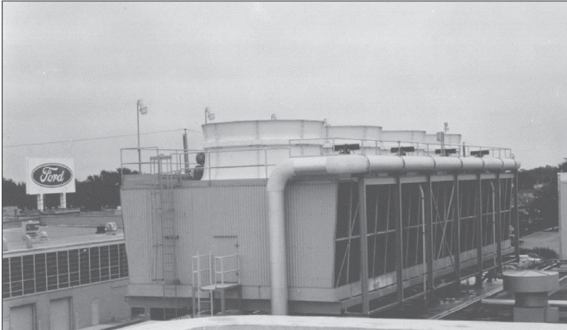
Figure 3.7. Photograph of induced draft cooling tower installation. (Courtesy of SPX Cooling Technologies, Inc., Overland Park, KS. With permission CRC Press [4].)
