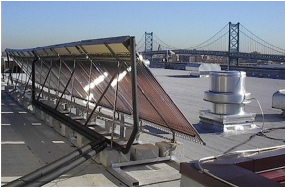
Figure 7.15. Evacuated tube solar water heating system on Social Security Building, Philadelphia, PA (photo by the author).
