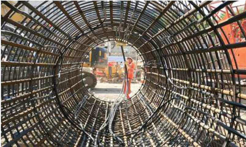
Figure 1.7. Installation of ground source heat pipe piping inside the foundation piles of buildings for a project in Abu Dhabi (Courtesy of M. Krarti [11]).
