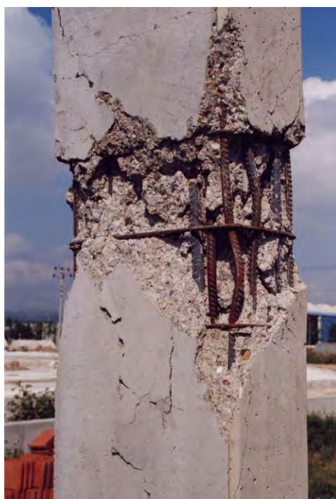
Fig. 2-8: Close-up of poor column details (1999 Kocaeli earthquake)
