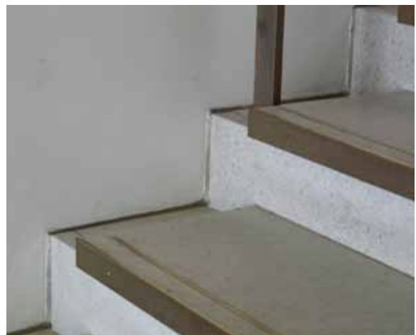
Although these nosings on stairs in a concert hall do not fully comply with the recommendations, they do satisfactorily identify the edge of the step by the brass inlaid strips on the treads and the visually contrasting band on the riser
