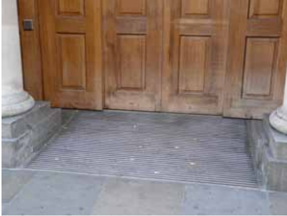
The single step at this recessed entrance has been replaced by a slope within the recess
