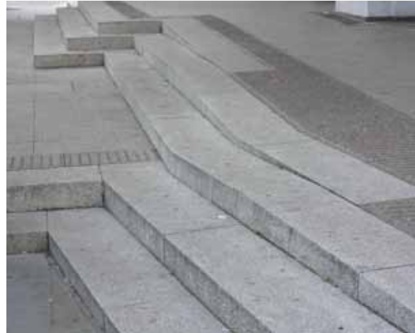
External steps with tapered risers to take account of a slope across the steps present a trip hazard and confusing tactile hazard warning. Note that the ribs of the corduroy tactile warning surface are at right angles to the steps: they should be parallel to the steps
