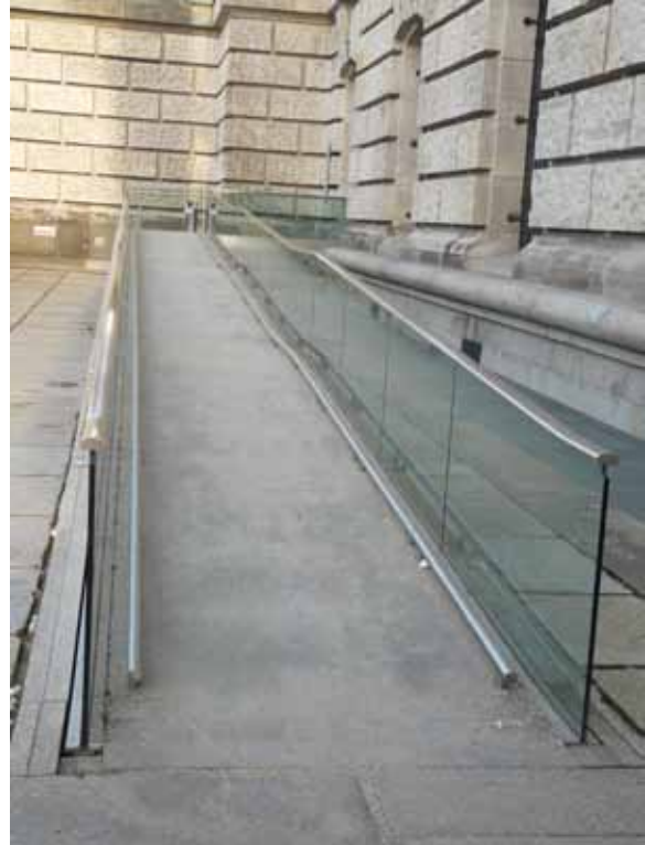
A continuous metal low rail protects the glass barrier on either side of the freestanding ramp and provides a tapping rail
