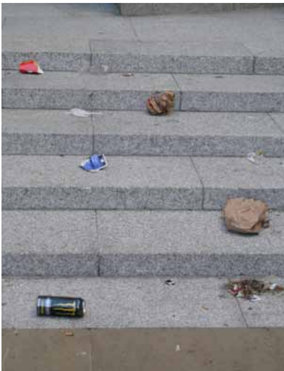
Litter on steps is a trip and slip hazard. Note the lack of nosings and tactile warning surface at the foot of the steps
