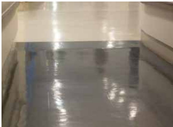
Bright ceiling lights reflected on the shiny surface of a ramp can cause glare and may be confusing
