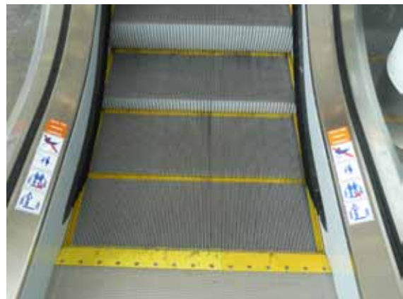
In healthcare buildings it is recommended that there is a yellow line at the back and sides of the treads to indicate that the steps are moving; it also helps people to stand in the right place, not too close to the edge of the step. Note the wide yellow band marking the comb plate
