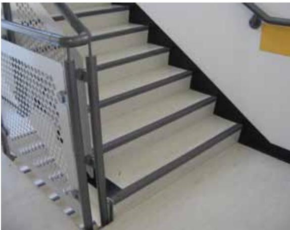
These simple square-edged stairs in a hospital have well-contrasted nosings that meet the recommendations
