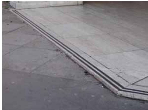
A single tapered step with a small rise is a trip hazard and should be replaced with a regraded sloping surface
