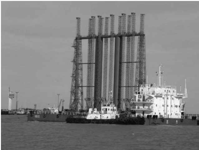
Figure 4.16 A PVD installation barge. (From Yan, S.W., Chu, J., Fan, Q.J., and Yan, Y. (2009). Building a breakwater with prefabricated caissons on soft clay. Proceedings of ICE, Geotechnical Engineering , Vol. 162, No. 1, pp. 3–12.)
