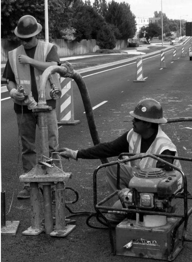
Figure 8.14 Hydraulic ram to extract LMG injection pipe. (Courtesy of Hayward Baker Inc.)
