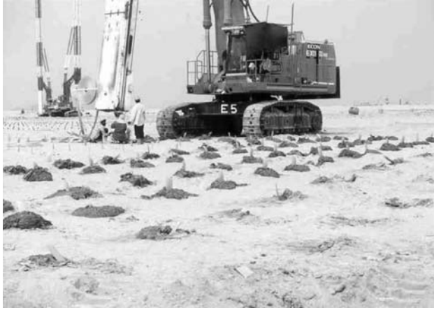
Figure 4.48 Extrusion of viscous pore water and mud during PVD installation. (From Chu, J., Bo, M.W. and Choa, V. (2006). Geotextiles and Geomembranes , Vol. 24, No. 6, pp. 339–348.)
