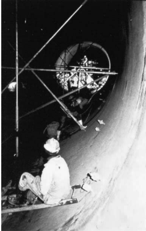
Figure 5.7 Drakensberg Pumped Storage Scheme, RSA, Tailrace Tunnel, Precompression grouting, ESCOM, Rodio SA, 1970s.
