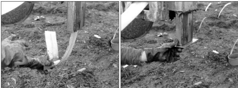
Figure 4.20 Use of an anchor plate for PVD installation. (Courtesy of J. Han.)
