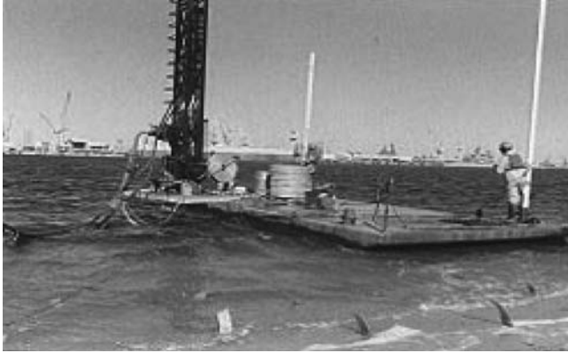
Figure 4.15 A floating raft for PVD installation in shallow water (From Chu, J., Bo, M.W. and Arulrajah, A. (2009). Soil improvement works for an offshore land reclamation. Proceedings of the Institution of Civil Engineers—Geotechnical Engineering , Vol. 162, No. 1, pp. 21–32.)
