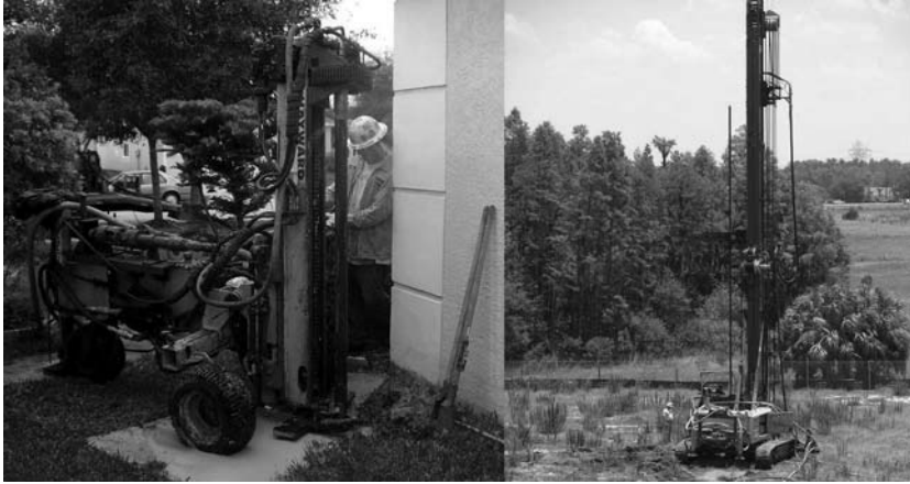
Figure 8.13 Small-wheeled and large-tracked drills to install LMG injection pipe. (Courtesy of Hayward Baker Inc.)
