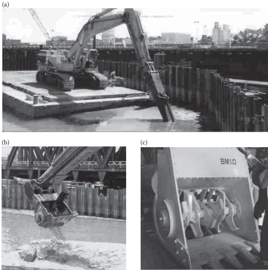
Figure 9.23 Shallow mixing equipment used at Fort Point Channel Site in Boston. (Courtesy of R. Jakiel.)
