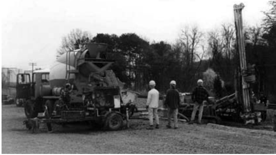
Figure 8.10 Concrete truck delivers LMG to grout site. (Courtesy of Hayward Baker Inc.)
