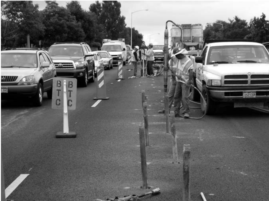
Figure 8.12 Hand equipment to install LMG injection pipe. (Courtesy of Hayward Baker Inc.)
