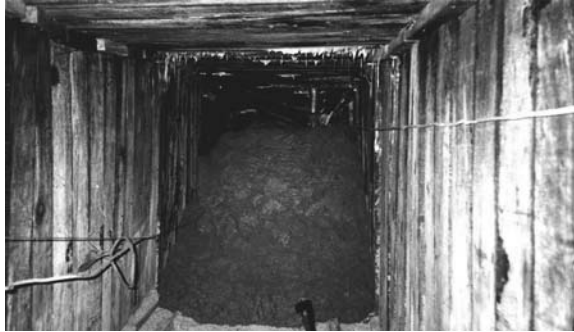
Figure 8.7 LMG used to fill a mine tunnel. (Courtesy of Hayward Baker Inc.)
