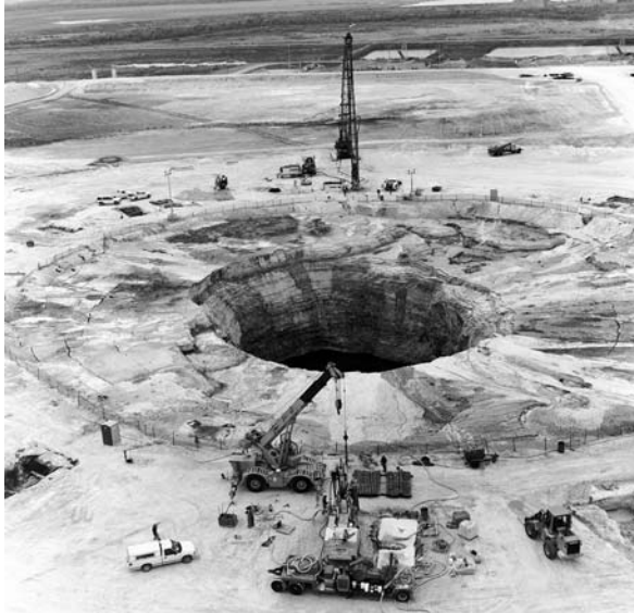
Figure 8.4 LMG to stabilise large sinkhole at a central Florida mining facility. (Courtesy of Hayward Baker Inc.)
