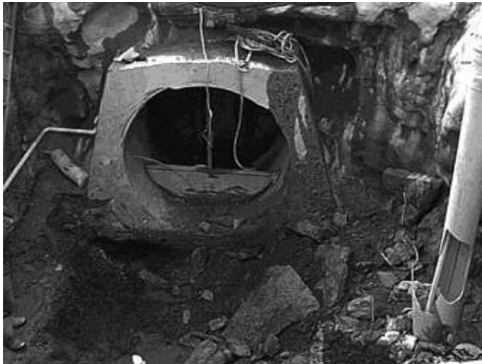
Figure 6.44 Soilcrete seal around and below the conduit with the bulkhead visible within the conduit.
