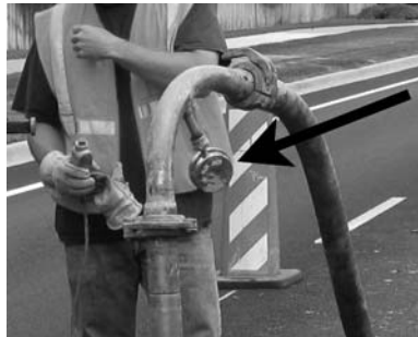
Figure 8.15 Pressure gauge and gauge saver near top of grout injection pipe. (Courtesy of Hayward Baker Inc.)
