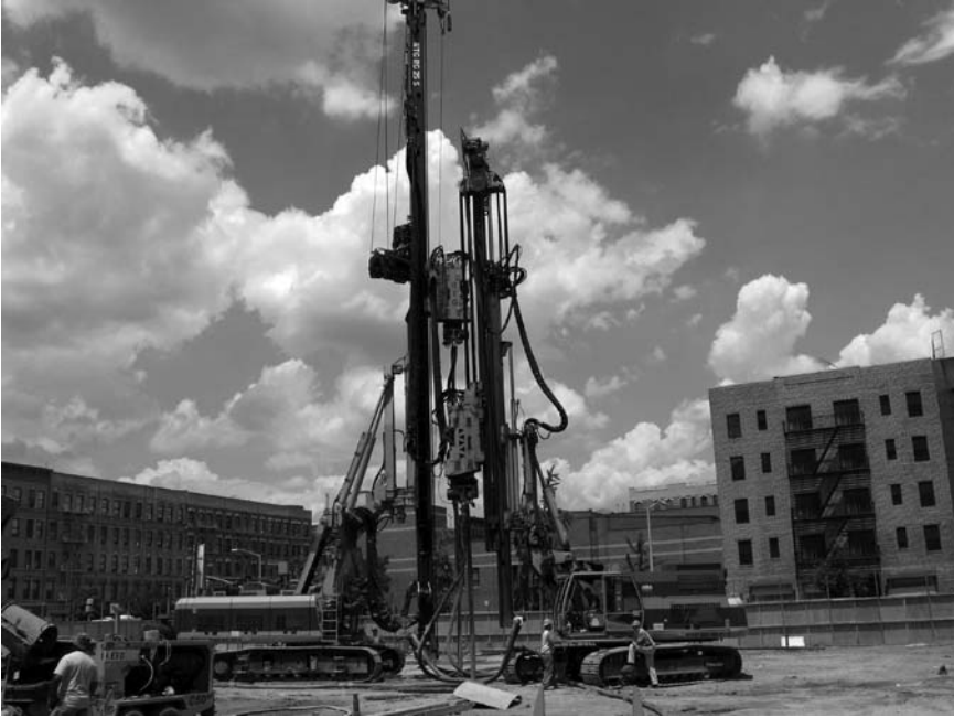
Figure 8.18 Large track-mounted drill rigs with telescopic masts installed the injection pipes in a single stroke to the maximum required treatment depth of 50 feet (15.2 meters). (Courtesy of Hayward Baker Inc.)
