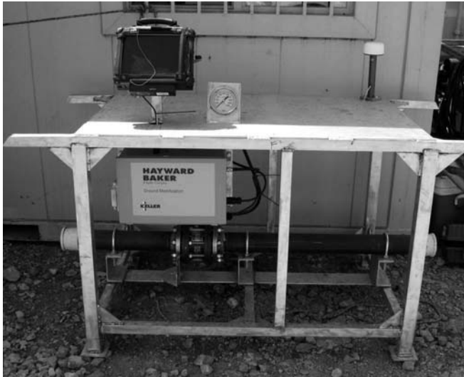
Figure 8.17 Compaction grout DAQ system with grout line under table where grout pressure and volume is measured. (Courtesy of Hayward Baker Inc.)
