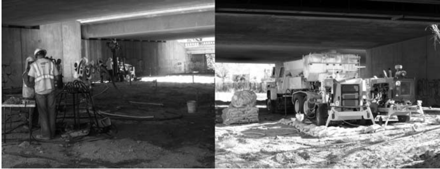
Figure 8.21 Small-tracked drill installing the injection pipes (left) and truck mounted batch plant producing LMG (right). (Courtesy of Hayward Baker Inc.)
