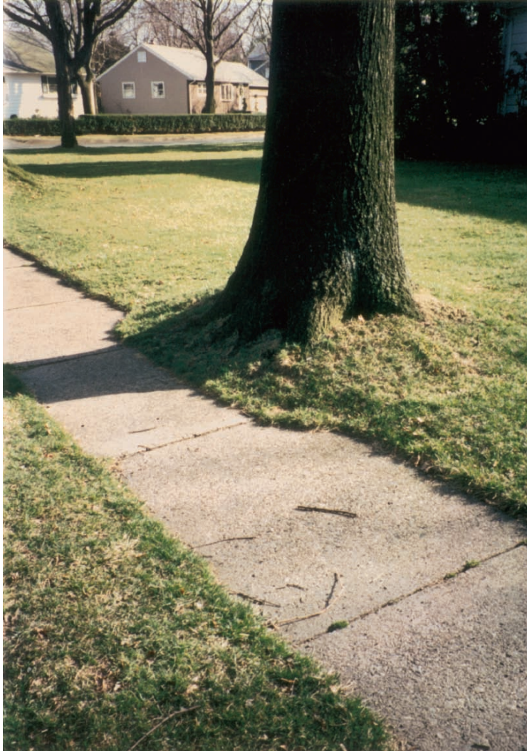
FIGURE 6. Contoured sidewalk creates “breathing room” for the tree. Photo, William R. Comery. Note: For most trees 10 to 12 feet of DeepRoot Barrier will be adequate to protect the sidewalk from future damage.
