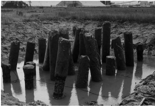
Fig. 6.11. Damaged pile shafts of a driven cast in place concrete pile group for a pier foundation
