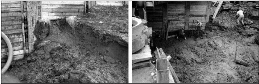
Fig. 4.8. Problems with soldier piles in excavation in soft lacustrine soil
