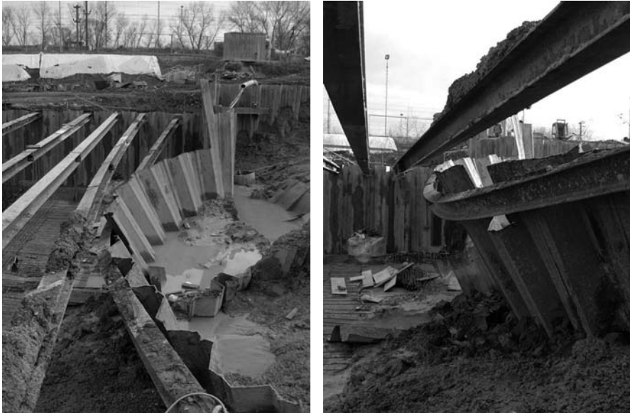
Fig. 4.133. Excessive deformation and collapse of an intermediate sheet pile wall
