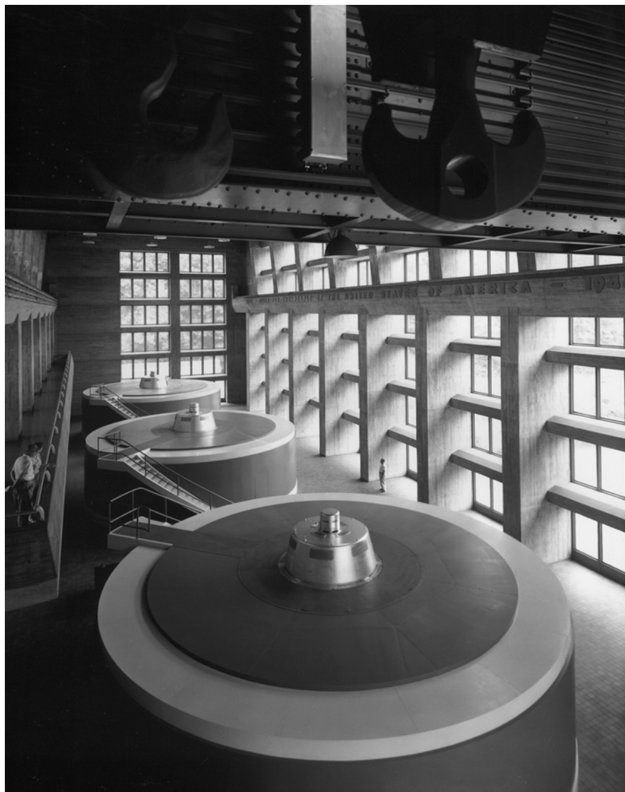
3.51 Inside powerhouse at Fontana Dam.
