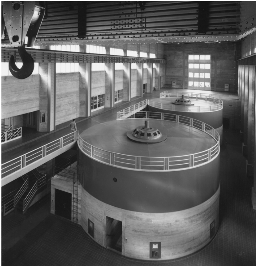
3.15 Interior view of powerhouse, Norris Dam.
