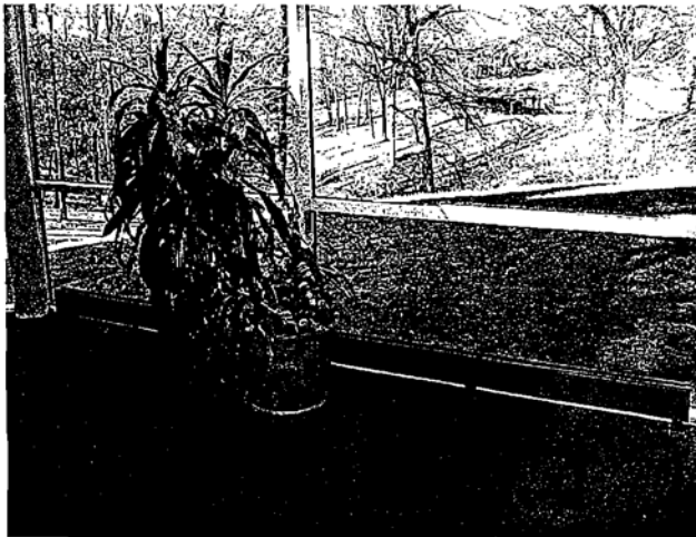
FIGURE 6.33. Baseboard finned tube radiation (FTR). (Photo by Vaughn Bradshaw.)
