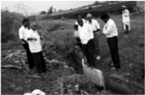
Reinforced fiber plastic cut throat flume on OT of Budhni minor canal: GLBC
