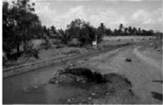
Damaged canal network
