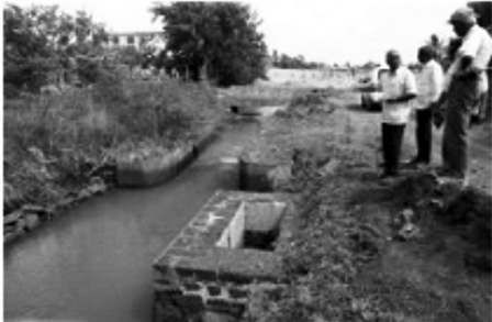
GLBC - stone masonry standing wave flume and gauge well on minor canal
