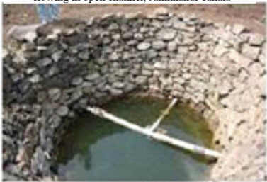
Collection well for subsurface drainage system reuse of drainage water, Jamkhandi Tahala
