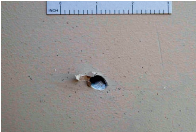
FIGURE 6.1 Powder pattern in painted wallboard.
