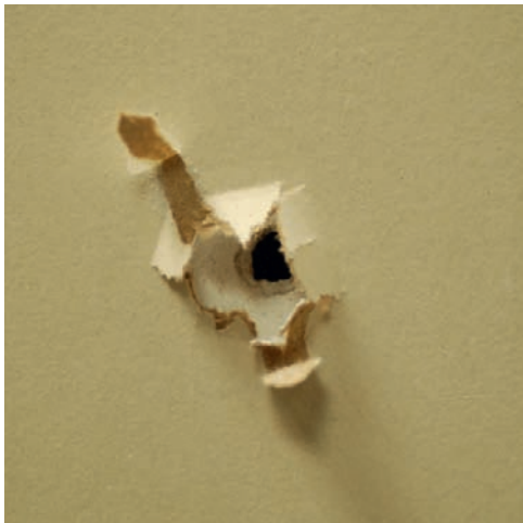
FIGURE 4.6 Typical exit from drywall with ragged edges and a noticeable lack of bullet wipe.
