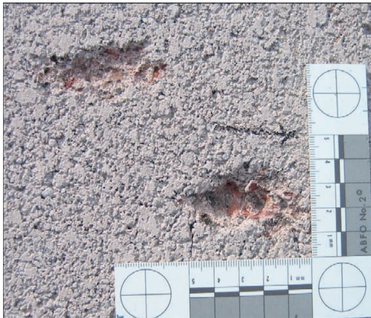
FIGURE 9.12 Two suspected impacts in a concrete block.
