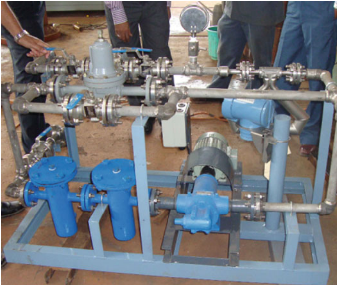
Fig. 5 Existing fuel flow measurement system
