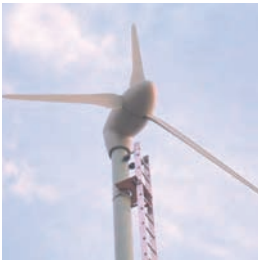
Figure 2.6 WES5 Tulipo turbine with access ladder (WES – Wind Energy Solutions)
