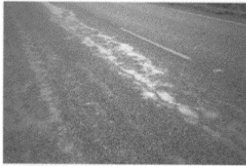
Figure 6 isolated fatigue cracking in foamed bitumen stabilised pavement, Allora.
