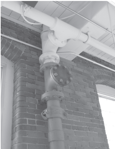
Figure 18.30 Sprinkler supply pipes
