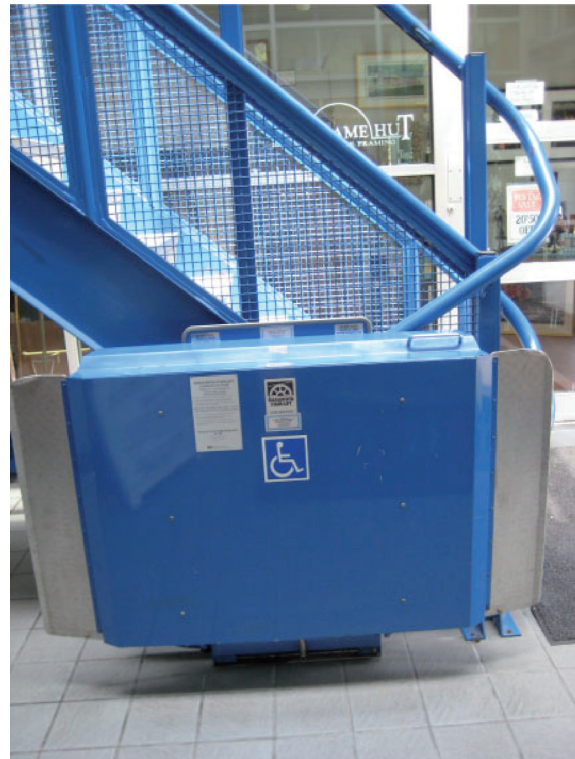
Figure 19.8 Inclined platform lift on stair
