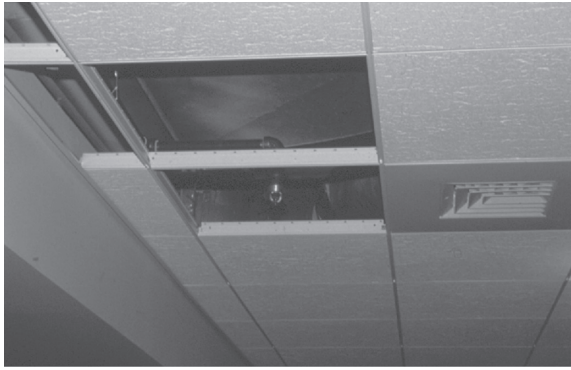
Figure 8.26 Acoustic ceiling tiles
