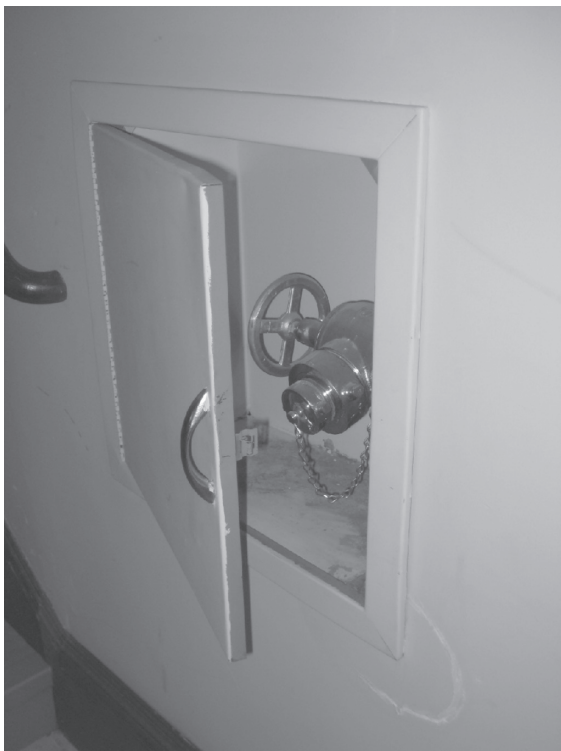
Figure 18.34 Standpipe access panel
