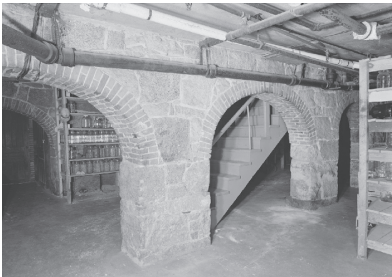
Figure 4.11 Masonry arch, Shaker Church Family Dwelling House, Enfield, New Hampshire Source: Library of Congress Prints and Photographs Division, Aubrey P. Janion, photographer, 1959
