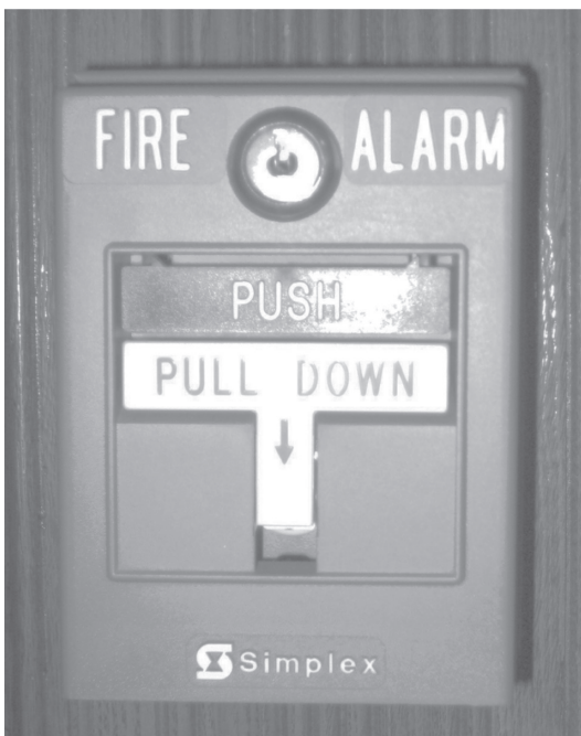
Figure 18.26 Fire alarm manual pull station
