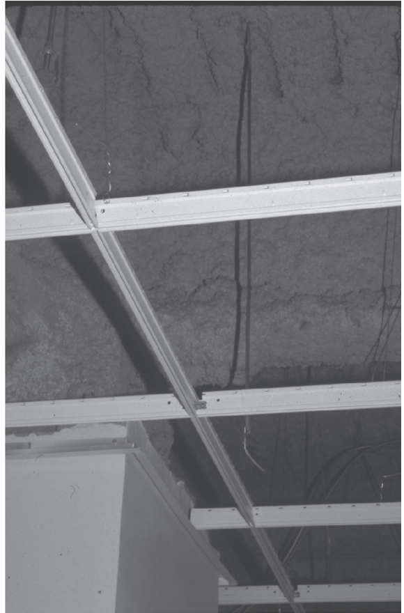
Figure 8.27 Suspended ceiling grid
