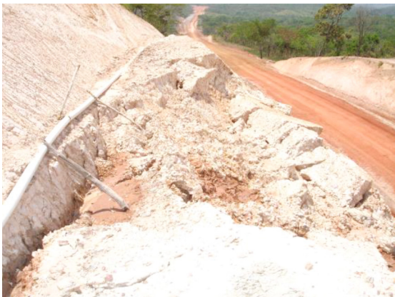
Fig. 12. Failure stretch in cut 25 slope.
