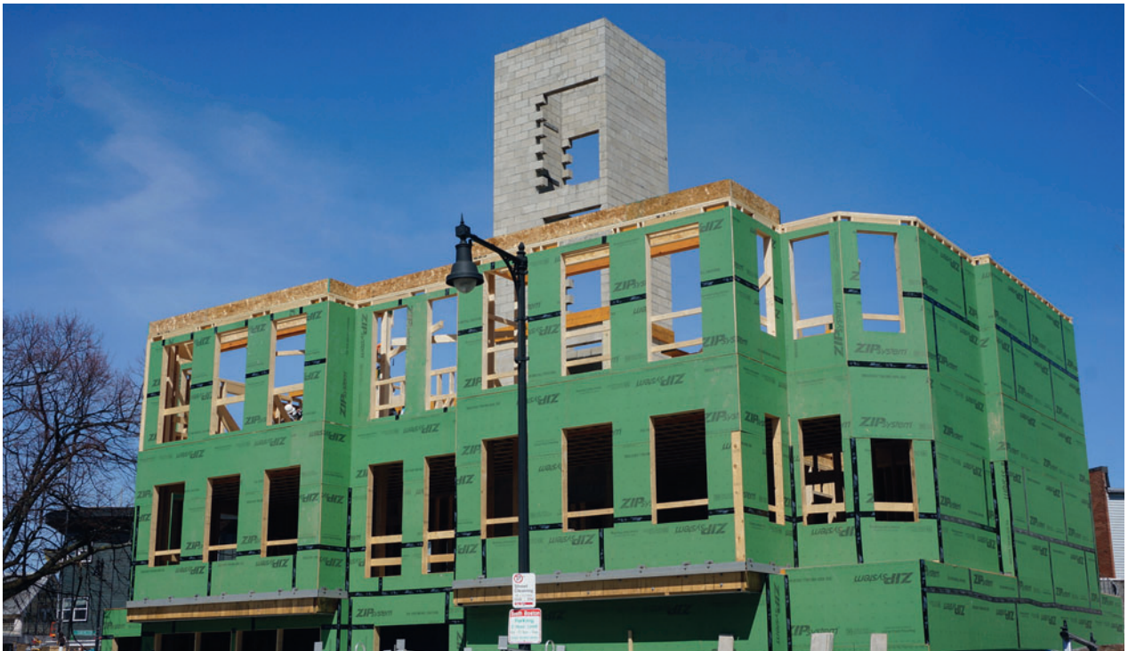
Figure 3.17 This Low-Rise Apartment Building In Boston, MA, Is Being Built With Light Wood Framing Methods Employed Across The Country
