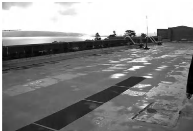
Figure 3.45 Plastic flat roof covering in a severe climatic exposure zone, by the coast.
