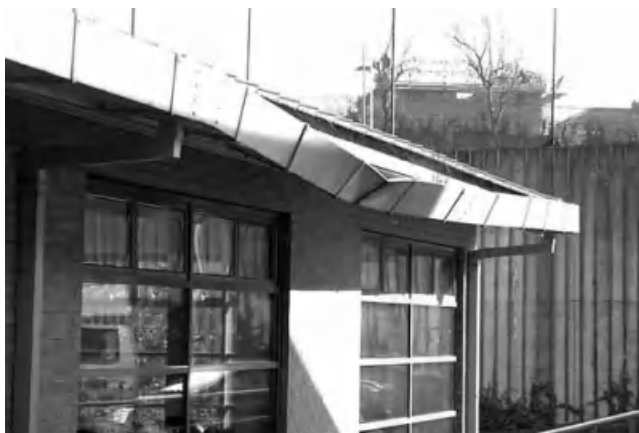
Figure 3.49 Gutter failure due to excessive snow loading in a traditionally procured school.
