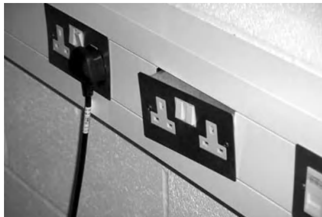
Figure 3.37 Poor electrical specification in a PFI school.
