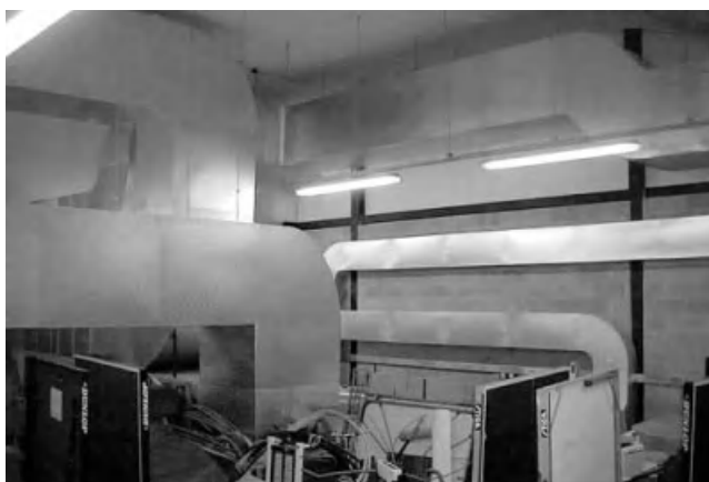
Figure 3.35 Oversized plant room in a traditionally procured school.
