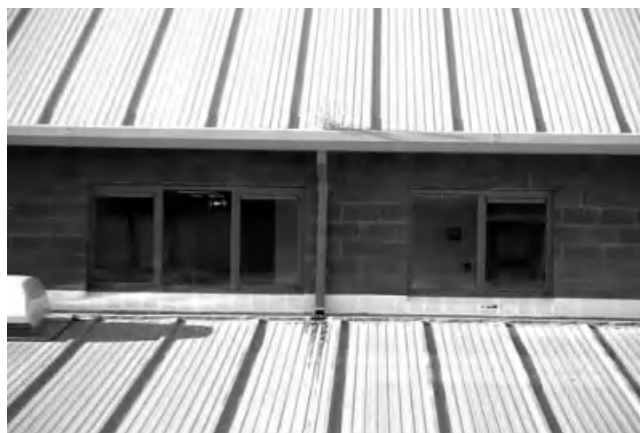
Figure 3.43 Vegetation growing at the top of a downpipe of a recently opened PFI school.
