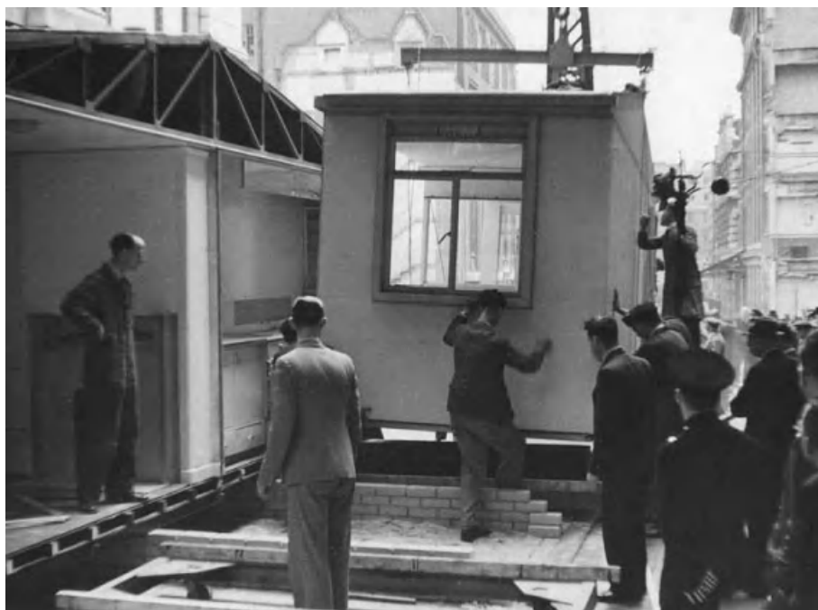
Figure 5.5 The aluminium temporary house: the last of the four sections being swung into place. Reproduced with permission from RIBA Library Photographs Collection.
