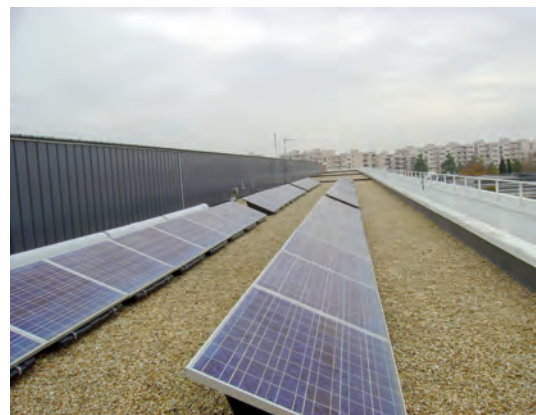
Figure 10.7 78m 2 of photovoltaic panels installed on the roof of the new block C
