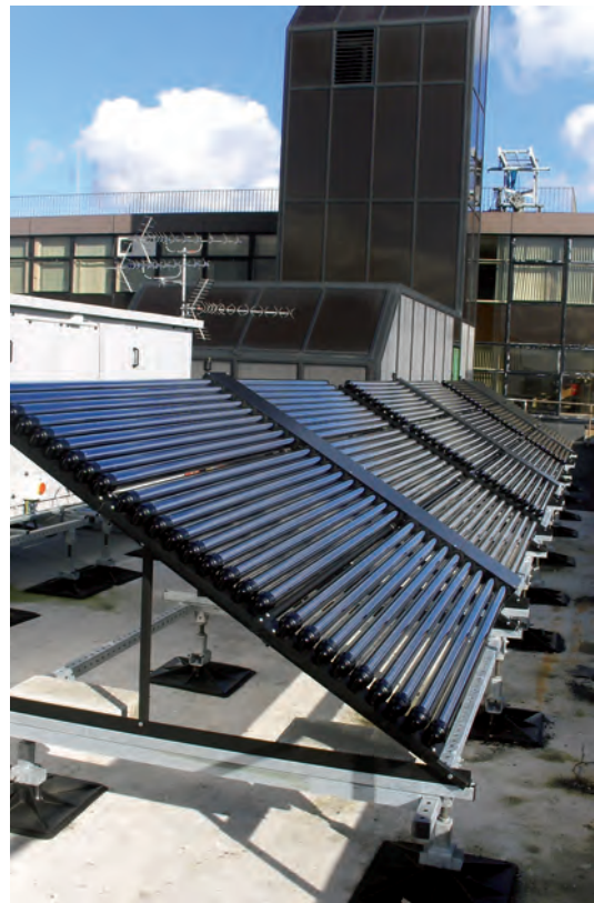
Figure 11.10 The evacuated tube array of solar thermal collectors contributing to domestic hot water
