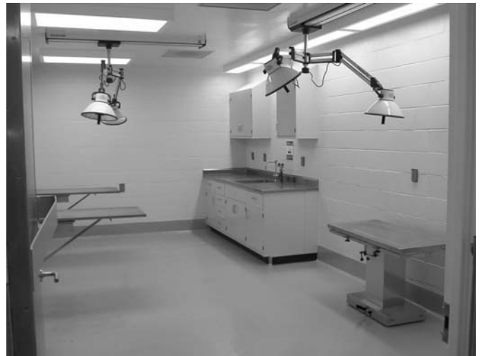
Fig. 21-4 Procedure room in indoor NHP facility.
