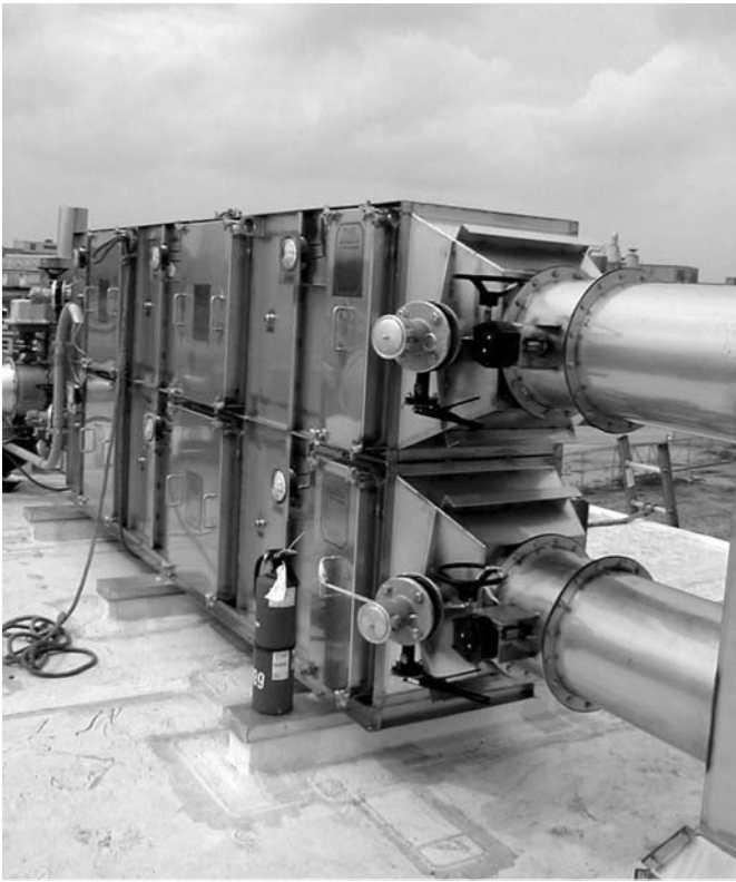
Fig. 34-5 Redundant bag-in/bag-out HEPA filters.
