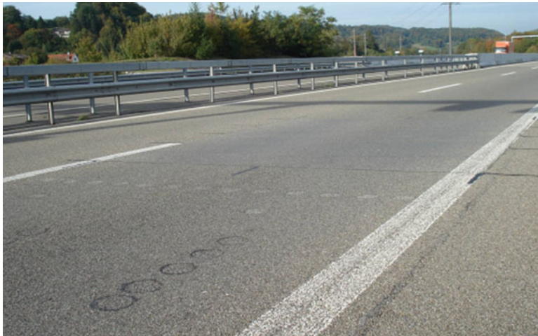
Fig. 4.47 Picture showing the surface course of the road after 10 years in service for bituminous layer system B
