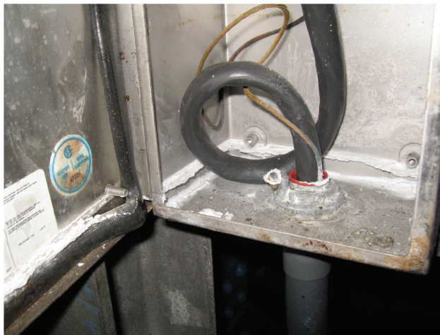
Figure 5. Electrical box with salt/debris build up and corrosion to conduit.
