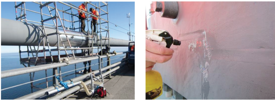
Figure 9. Storebælt Bridge, equipment setup for flow test and leakage at longitudinal joint.
