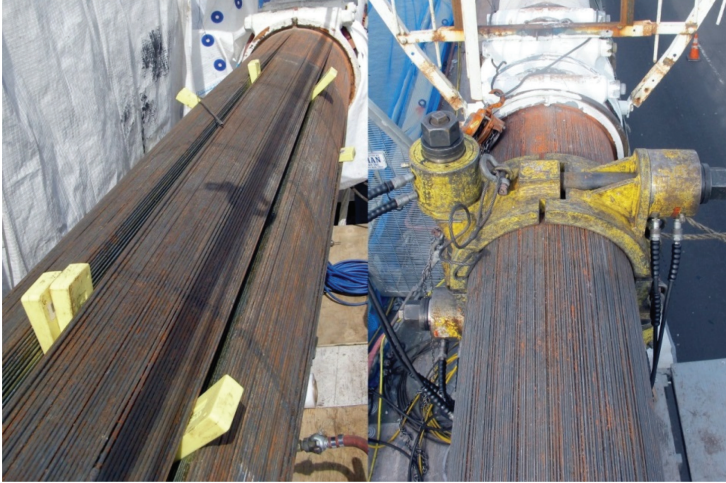
Figure 12. Inspection and re-compaction of a 100-year-old cable.
