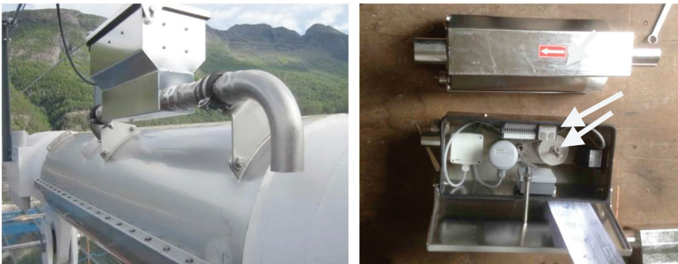
Figure 17. Exhaust sleeve with damper, bolt for adjustment of damper – see arrow, Hardanger Bridge.
