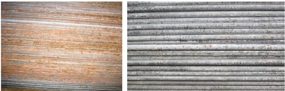
Figure 1. Corrosion on main cables, roughly 30 (left) and 15 (right) years old.
