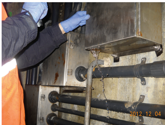
Figure 6. Electrical box in tail lock area with water still flowing out after 1 month.
