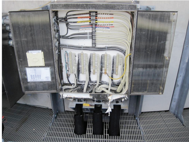
Figure 7. Submarine cable terminal box partially submerged—note clear line showing water elevation.
