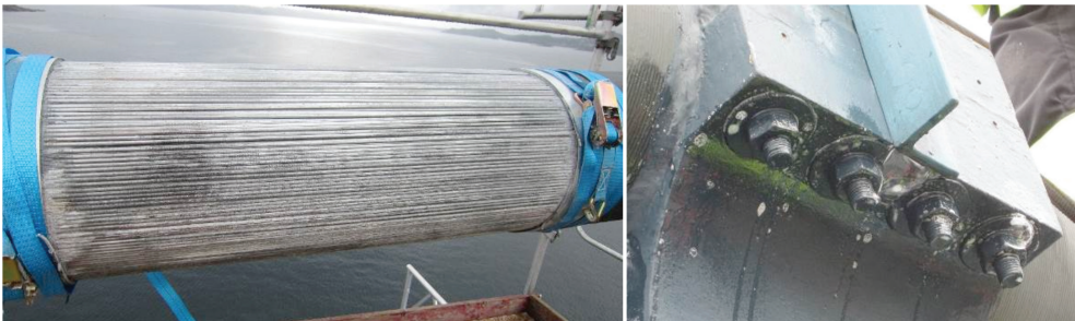
Figure 11. Storda Bridge, cleaned cable at injection point and leakage at washer on cable band.
