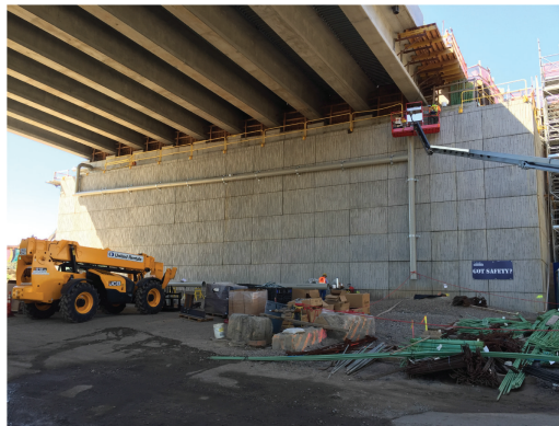
Figure 17. Front face of abutment with T-WALL® units.
