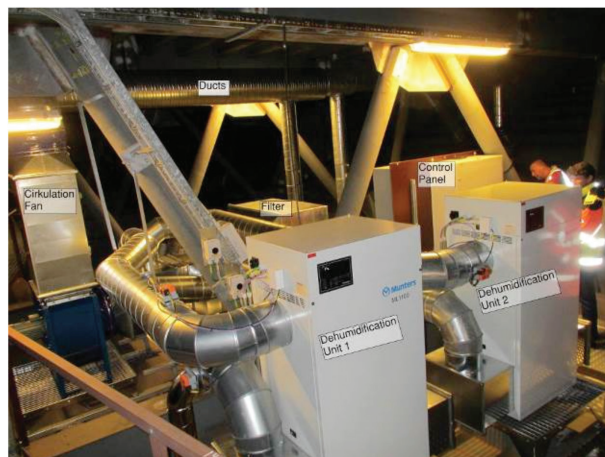
Figure 14. Dehumidification plant for main cables, Storebælt Bridge.
