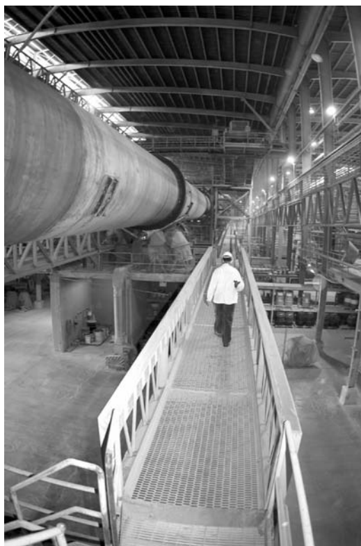
Figure 5.7 Long cement kiln without preheating and precalcination tower (St Lawrence Cement, Joliette Plant) (courtesy of Philippe Pinsonneault, Ciments St-Laurent).
