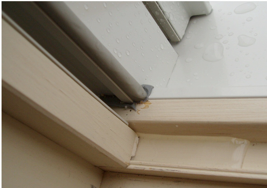
PHOTO 2. Water collecting in an undrained trough or gutter.
