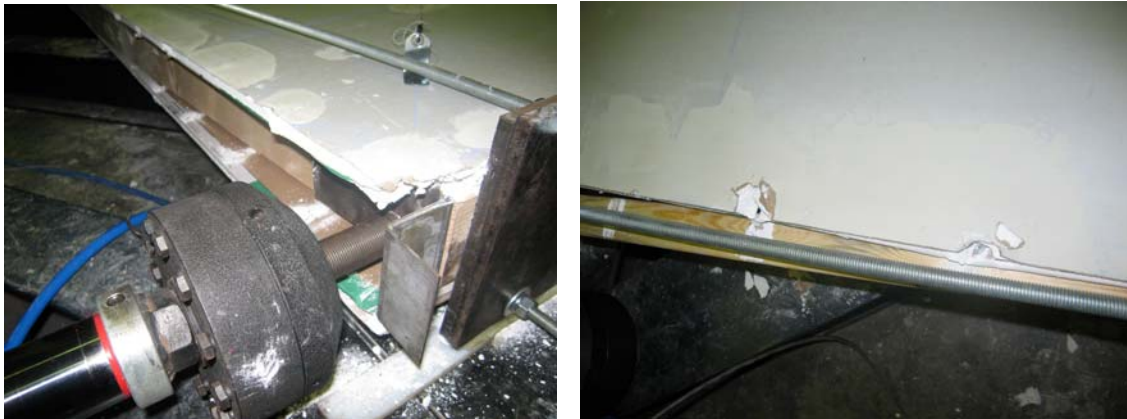
Figure 10. Screws on end studs tearing through drywall
