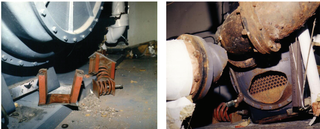
Figure 1. Pipe rupture resulted from failure of vibration-isolator supports of a chiller, 1994 Northridge Earthquake (Photo Credits: Lloyd 2003).
