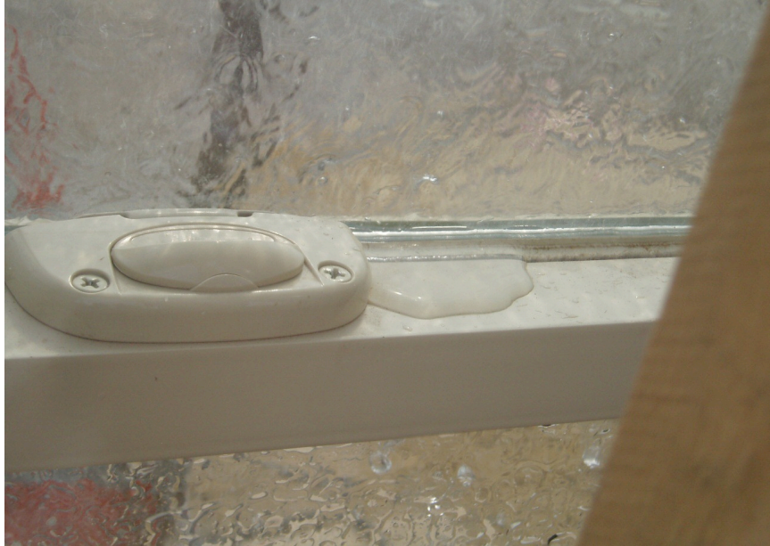
PHOTO 1. Water collecting on the window meeting rail.
