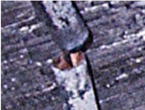
Figure 18 – AHJ Fire-Incident Image showing Joint Separation, Visible Wires and No Couplings Visible.
