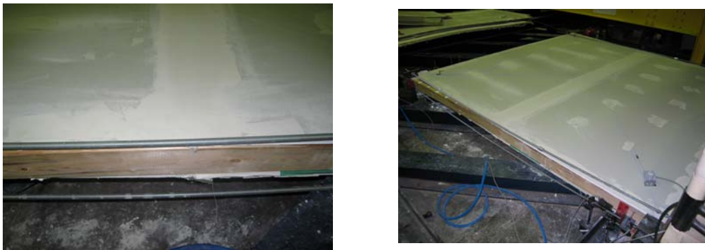
Figure 9. No crack through any part of the horizontal joint finished with OnePass compound
