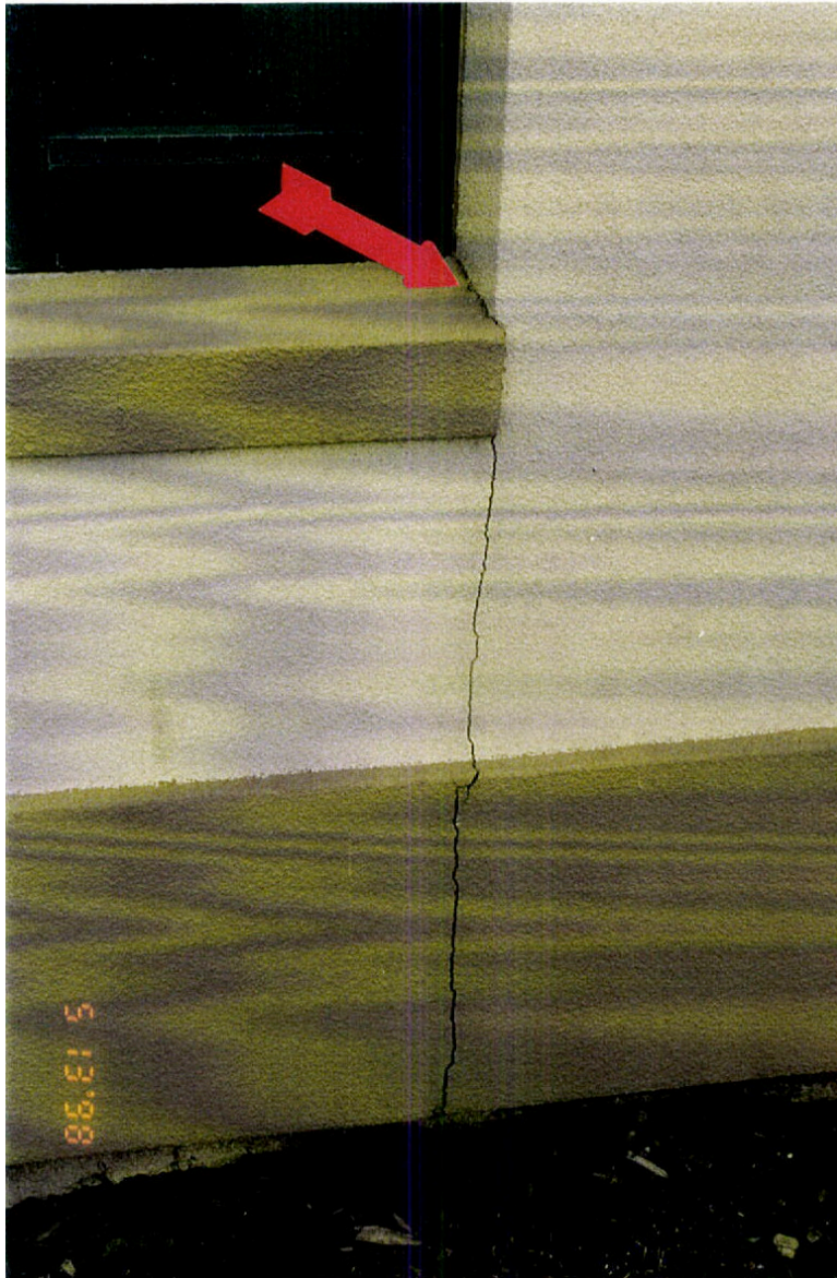
Figure 3: Typical cracking visible at the corners of openings in the wall system; cracking at the base at an EPS joint
