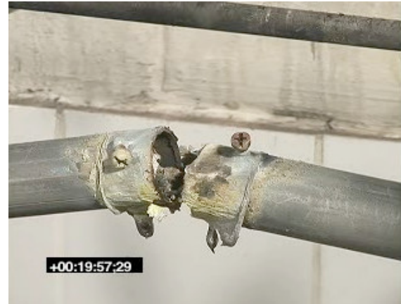
Figure 16 - Complete failure of Die-Cast Coupling
