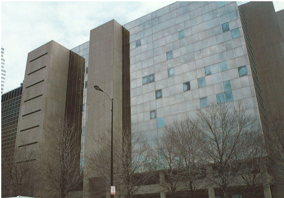
Figure 2: Fogging of IG units observed from the building exterior.
