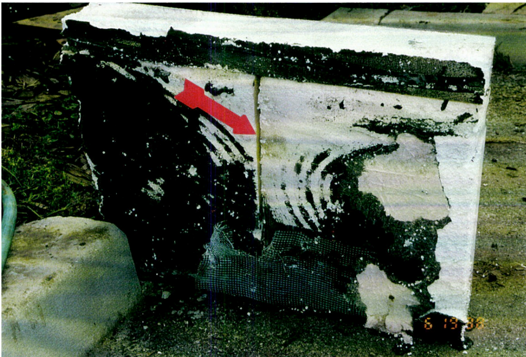
Figure 6: Exterior destructive examination revealed an underlying cause of cracking near the base of the EIFS was a gap in the EPS boards, which should have been installed plumb, with an EPS sliver wherever necessary
