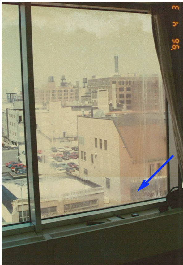
Figure 1: Fogging of IG unit observed from inside the building.
