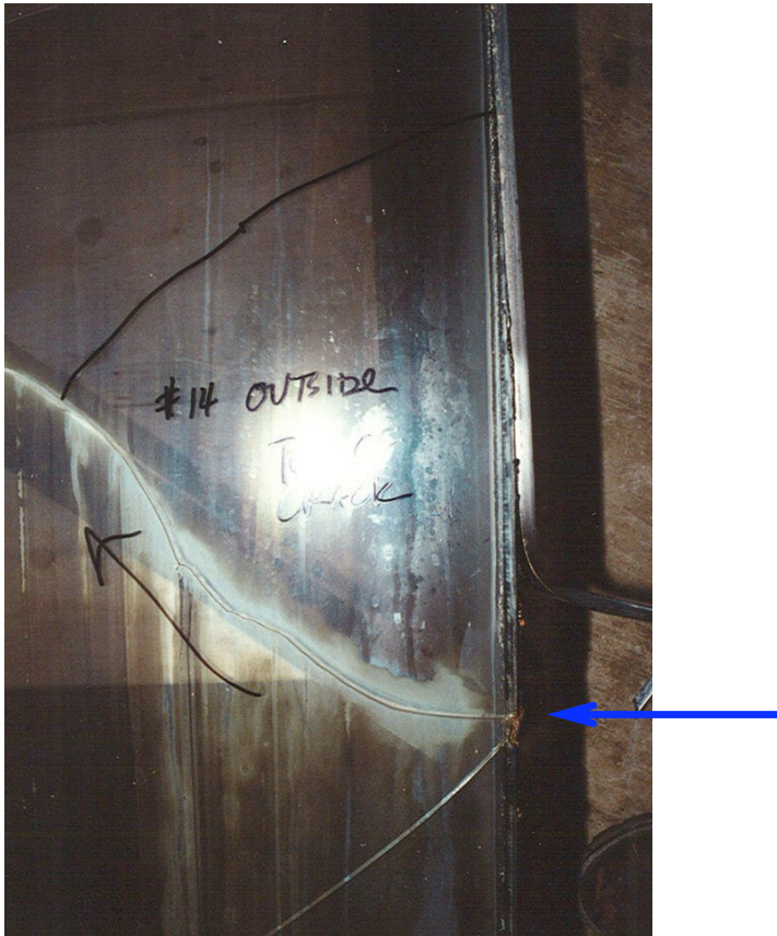
Figure 3: Corrosion by-products can induce compressive forces on the glass and crack the glass.
