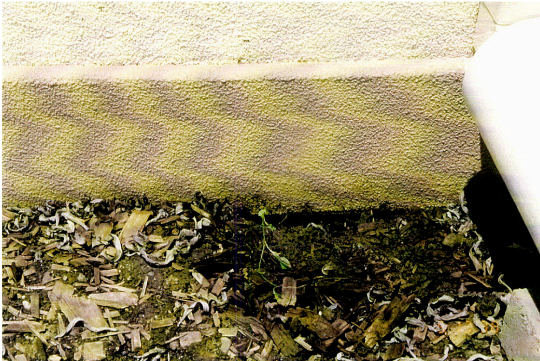
Figure 5: EIFS located too close to grade and more susceptible to water infiltration and premature degradation
