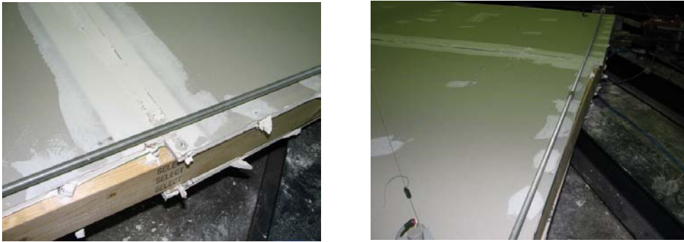
Figure 6. Sliding of drywall sheets at the joint and tearing of drywall by edge stud screws
