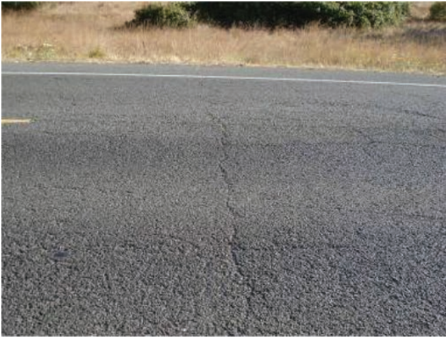
Figure 1. Existing pavement showing cracking and raveling.
