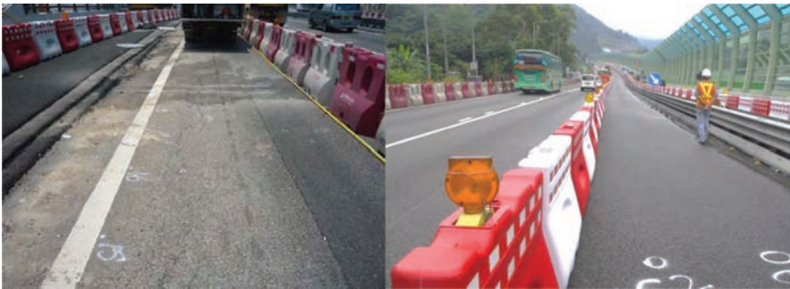
Figure 1. General conditions of Tuen Mun Rd (left: distressed section, right: non-distressed section).
