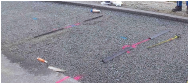
Figure 3. Triangle steel bars and T shaped steel bars fixed in the UGM.
