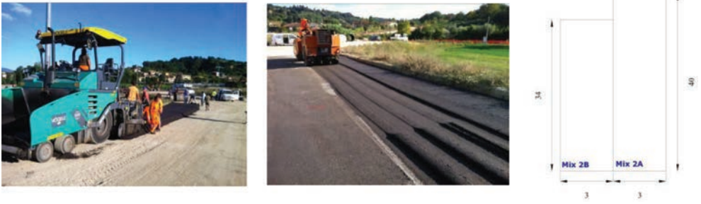
Figure 1. Pictures taken during laying and compaction on the left. Dimensions of trial section on the right.
