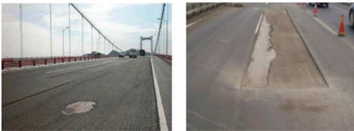
Figure 5. Debonding at the interface of asphalt surfacing and steel bridge decks.
