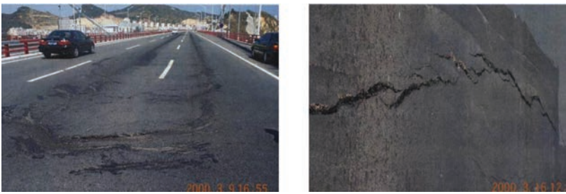
Figure 4. Slippage cracking of SMA asphalt layer.
