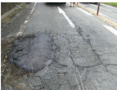
Photo 7. Urgent repair situation.
