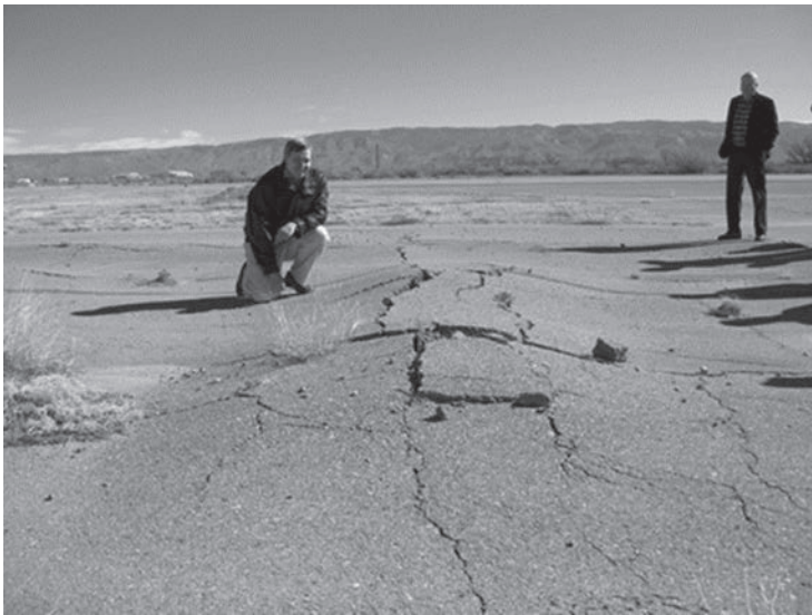
Figure 3. Swelling from sulfate attack on Type V cement-stabilized subgrade, Holloman AFB.
