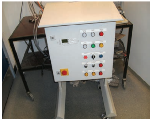
Figure 3. Thermal cycling device control unit.
