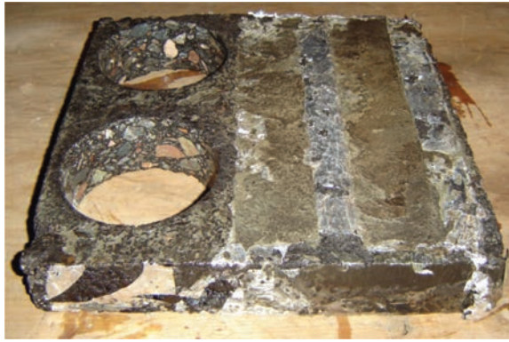
Figure 5. Specimens cored from the slab.
