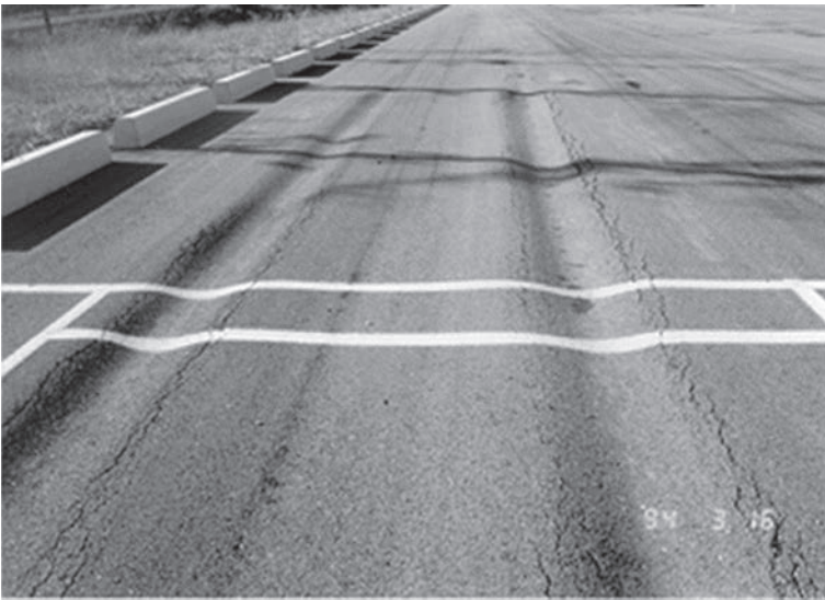
Figure 2. Subgrade shear failures, Ft. Leonard Wood.
