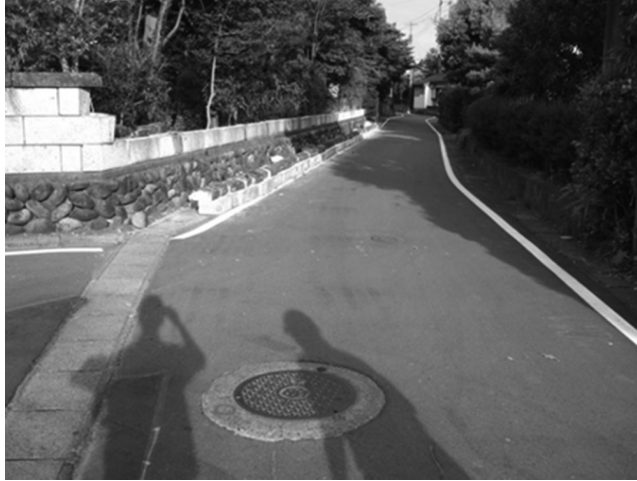
PHOTO 21.10 No damage to sewer manhole and its backfill treated with cement in Kashiwazaki city (reconstructed after the 2004 Niigataken-Chuetsu earthquake). (From Sasaki, T. et al., Found. Eng. Equipment (Kisoko) , 36(9), 25, 2008 [in Japanese].)
