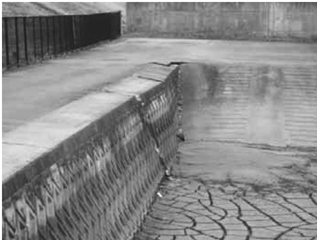
FIGURE 20.26 Cracks at the bottom of sludge basin.
