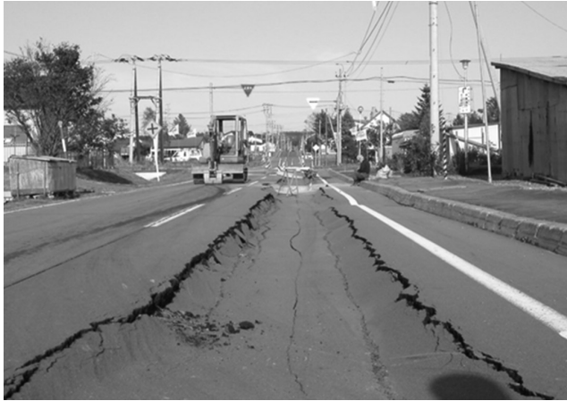
PHOTO 21.4 Settlement of sewer pipe backfill with excavation depth of about 3 m in Toyokoro town caused by the 2003 Tokachi-Oki earthquake.
