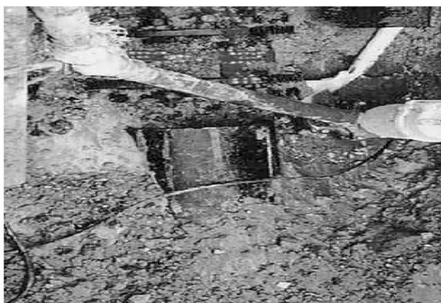
FIGURE 20.6 Pulling out of mechanical joint of a ductile cast iron pipe of 300 mm diameter.
