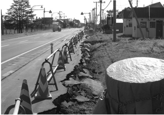
PHOTO 21.6 Uplift of sewer manhole and settlement of untreated backfill in Onbetsu town caused by the 2003 Tokachi-Oki earthquake.
