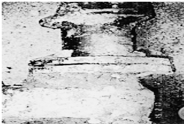
FIGURE 20.15 Loosening of flange bolt of gate valve.
