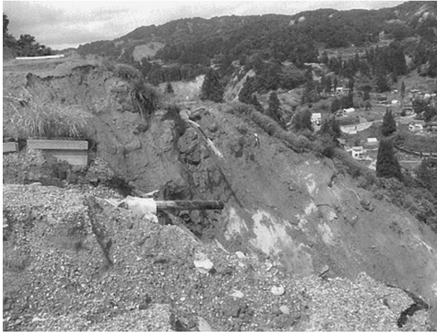
FIGURE 20.36 Pulling out of mechanical joint (K type) of ductile.
