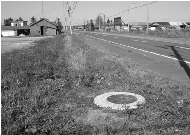
PHOTO 21.5 No damage to sewer manhole and its backfill treated with expanded polystyrene bead and cement in Onbetsu town.
