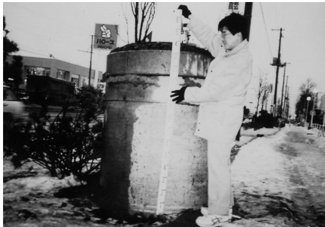
PHOTO 21.1 Uplifted sewer manhole in Kushiro town caused by the 1993 Kushiro-Oki earthquake. (From Koseki, J. et al., Soils Found. , 40(1), 99, 2000.)
