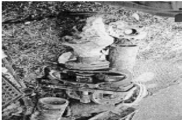
FIGURE 20.17 Broken body of air valve.
