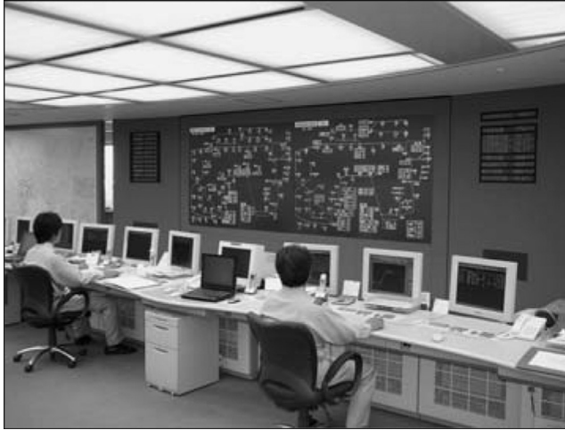
FIGURE 4.9 Supply control center.
