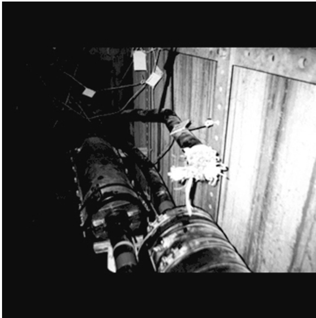
FIGURE 24.5 Damaged underground cables.
