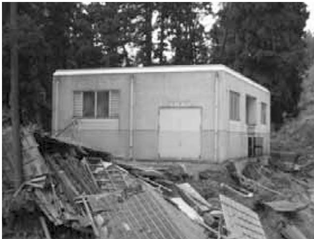
FIGURE 20.28 Ground displacement due to landslide in the purification plant.
