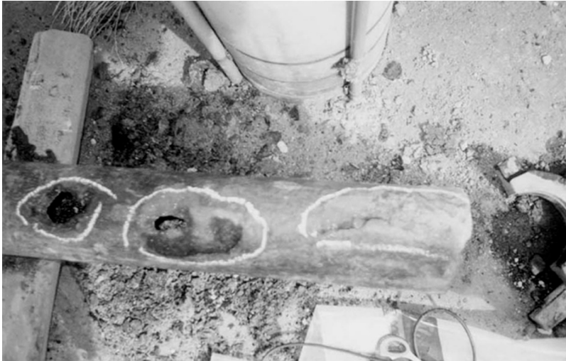
FIGURE 14.2 External corrosion of ductile cast iron pipes.
