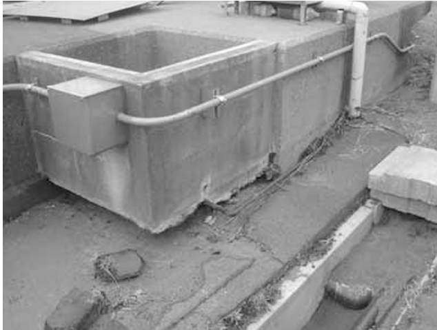
FIGURE 20.21 Settlement of related structures.
