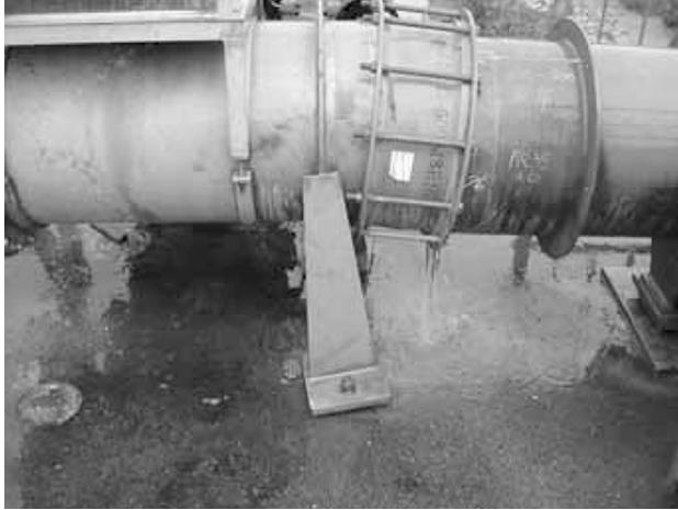
FIGURE 20.33 Deformations of expansion joint and ring support.
