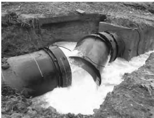
FIGURE 20.43 Flood from expansion joints of 2400 mm diameter.
