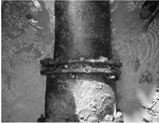
FIGURE 20.44 Leakage from expansion joint of 150 mm diameter.
