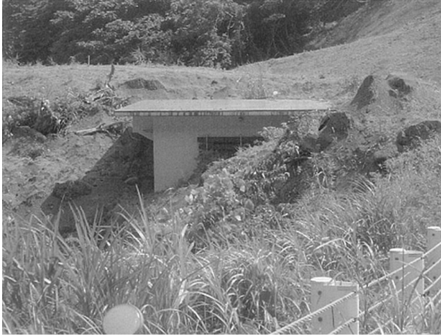
FIGURE 20.29 No. 1 pumping station buried due to ground collapse.
