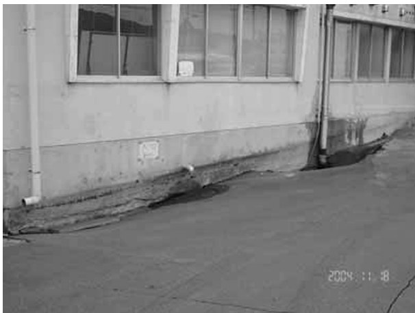
FIGURE 20.20 Settlement of an office.
