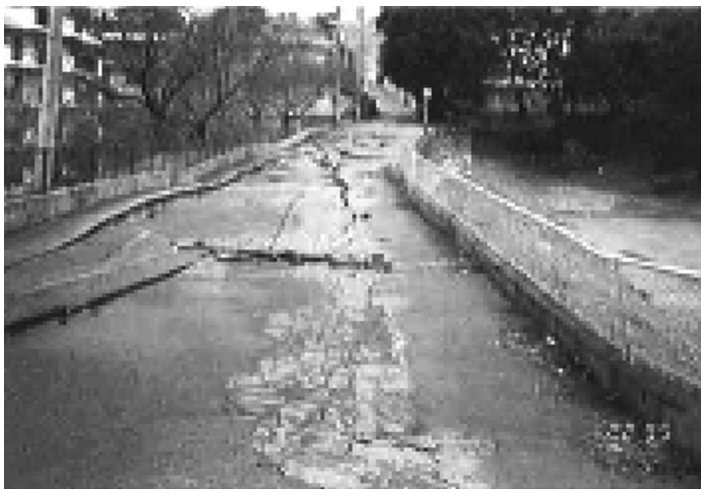
FIGURE 20.2 Damage of embankment of the lower reservoir in Niseko.
