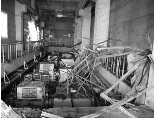
PHOTO 21.14 Damage to South Gamo sewage treatment plant in Sendai city, Miyagi, prefecture induced by tsunami inundation after the 2011 off the Pacific coast of Tohoku earthquake. (Courtesy of Japan Sewage Works Association, Tokyo, Japan.)
