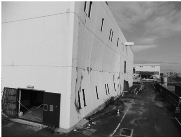
PHOTO 21.15 Damage to wall of South Gamo sewage treatment plant in Sendai city, Miyagi, prefecture induced by tsunami force after the 2011 off the Pacific coast of Tohoku earthquake. (Courtesy of Japan Sewage Works Association, Tokyo, Japan.)
