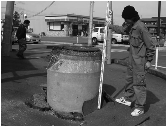
PHOTO 21.7 Uplift of sewer manhole in Ojiya city caused by the 2004 Niigataken-Chuetsu earthquake.
