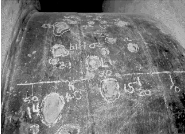
FIGURE 14.4 Macrocell corrosion between concrete and steel pipe. (Corrosion occurred during 11 years following installation in 1980.)
