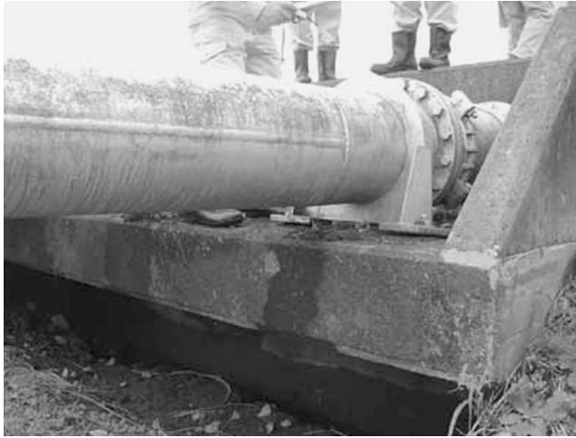
FIGURE 20.23 Uplifting of foundation of pipe bridge.
