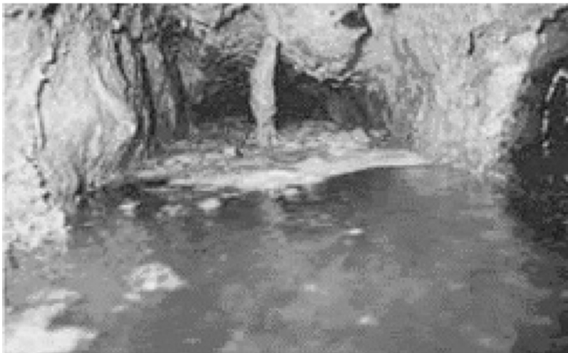
FIGURE 15.8 FOG in sewer.
