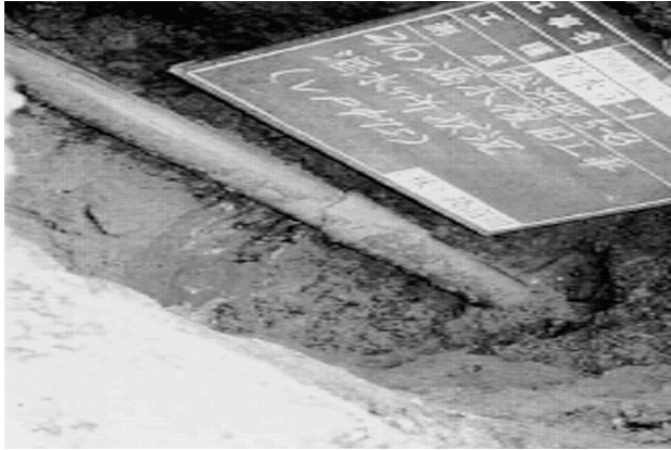
FIGURE 20.11 Leakage from a rigid polyvinyl chloride pipe of 75 mm diameter at the slope area.
