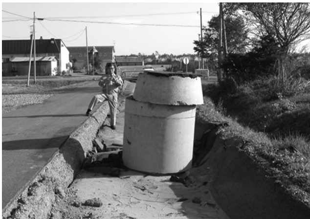
PHOTO 21.3 Uplift of sewer manhole and settlement of its backfill with excavation depth of about 5 m in Toyokoro town caused by the 2003 Tokachi-Oki earthquake.
