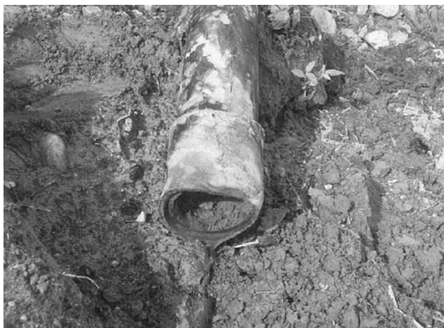
FIGURE 20.40 Joint failure of polyethylene pipe covered by coated steel plate.
