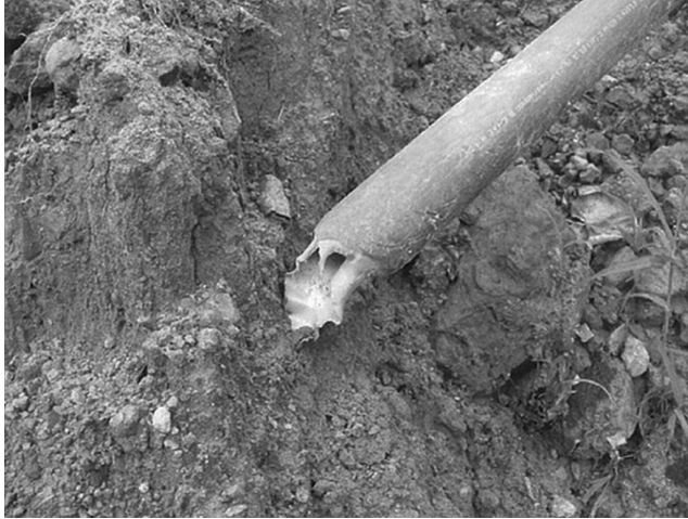
FIGURE 20.38 Broken pipe body of polyethylene pipe.
