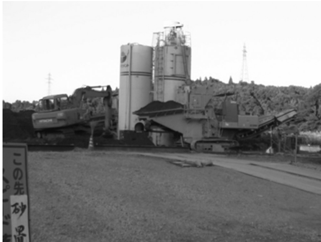
PHOTO 21.9 Cement-treatment plant facility in Nagaoka city constructed after the 2004 Niigataken-Chuetsu earthquake.
