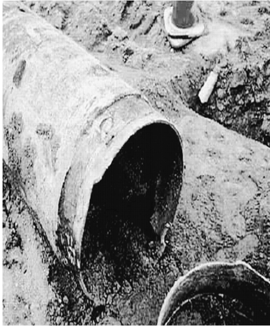
FIGURE 20.7 Damage of welded joint in a steel pipe of 600 mm diameter.
