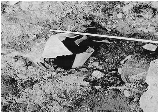
FIGURE 20.8 Pulling out of mechanical joint in a ductile cast iron pipe of 350 mm diameter.
