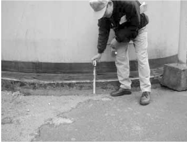
FIGURE 20.25 Ground settlement around the filter basin.
