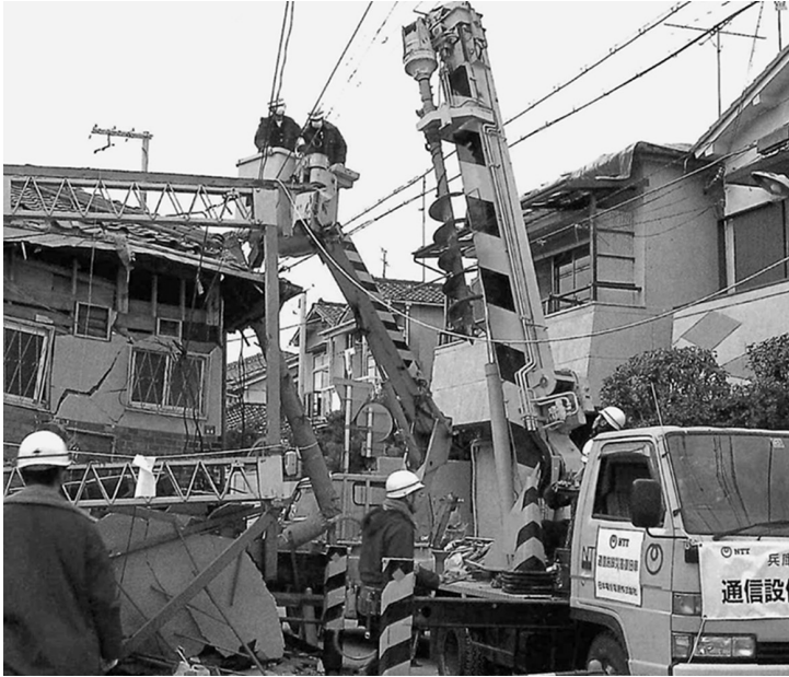
FIGURE 24.4 Damage and restoration of aerial cables.
