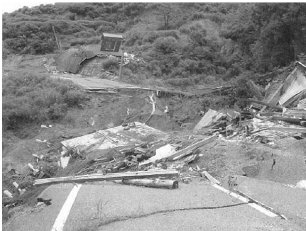
FIGURE 20.35 Situation of road collapse.
