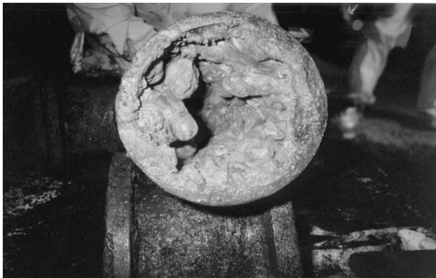
FIGURE 14.5 Corrosion at the internal surface of cast iron pipe.
