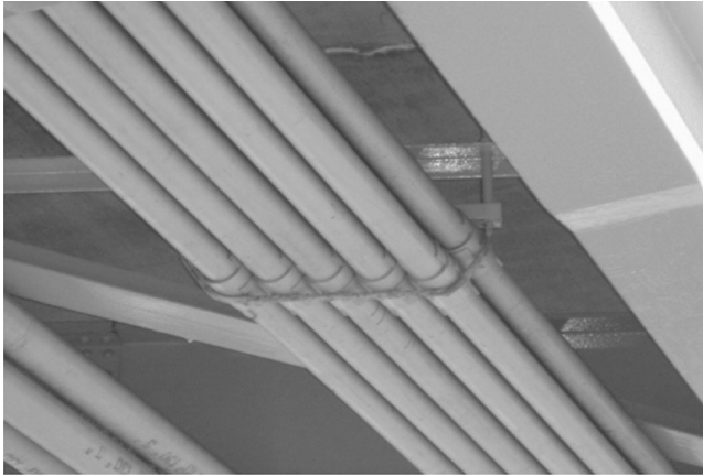
FIGURE 12.27 Conduits attached to a bridge.
