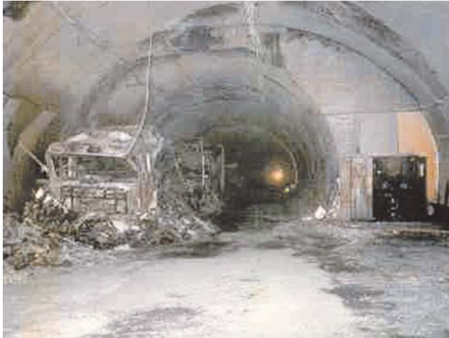
FIGURE 3 Mont Blanc Tunnel after fire.
