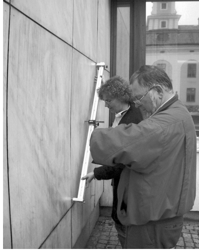
FIG. 12—Measurements of bowing amplitudes on a marble façade with the use of a “Bow-meter.” Photo by Björn Schouenborg.
