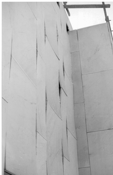
FIG. 1—Bowling of marble panels (1998) on the Finlandia Hall, Helsinki, Finland. Photo by Bent Grelk.
