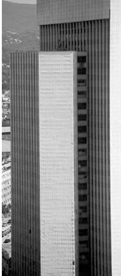
FIG. 14—Zagrepcanka building in Zagreb with concave bowing on the lower part and convex bowing of the upper part of the façade. Photo by Jan Anders Brundin.
