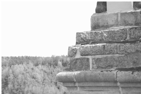
FIG. 5—Displaced granite at tower corner. Note sealant was installed around granite at mortar joints.
