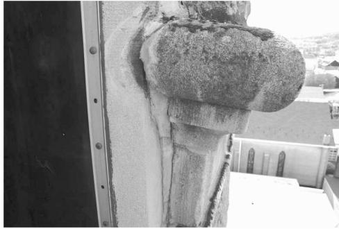
FIG. 4—Outwardly displaced limestone, nearly 3 in. Note joint opened by displaced masonry was filled with mortar during repair efforts, which will both conceal and cause further outward displacement.
