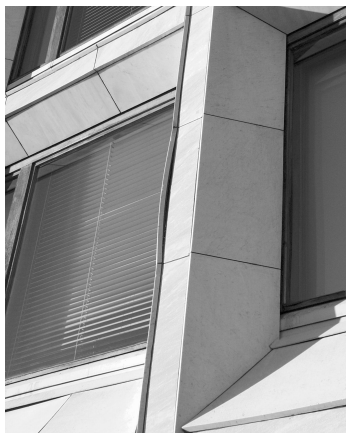
FIG. 5— The same marble can display different bowing patterns on the same building. Horizontal panels are concave and the vertical ones are convex.
