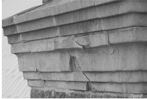
FIG. 8—Cracked and spalled limestone at upper portion of tower.
