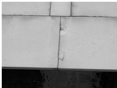
FIG. 3—Expansion of the marble panels creating cracking and spalling around the anchoring points, on a building façade in Malmo, Sweden. Photo by Bent Grelk.
