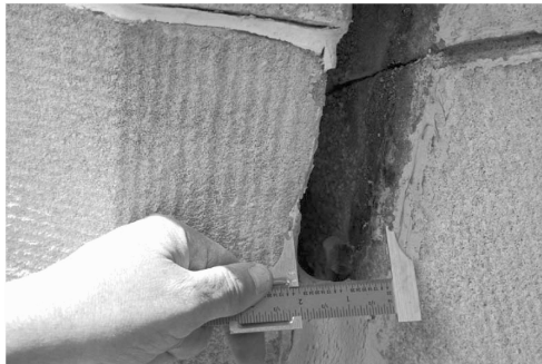
FIG. 3—Displaced limestone opening at joint, nearly 2 in. wide. Note sealant was installed covering widened joint.
