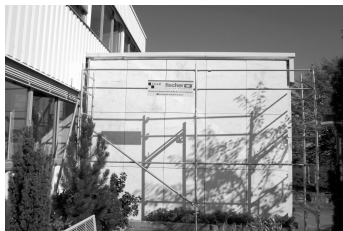
FIG. 3—Test wall at fischerwerke in Waldactahl, SW Germany. One marble type in combination with five different anchoring systems were installed.
