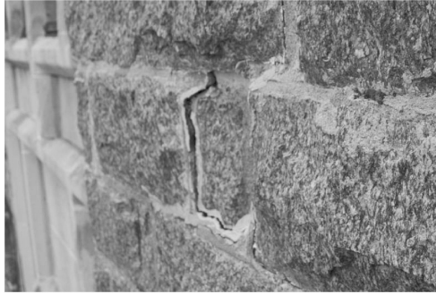
FIG. 6—Outwardly displaced (nearly 3/4 in.) granite at top of tower.
