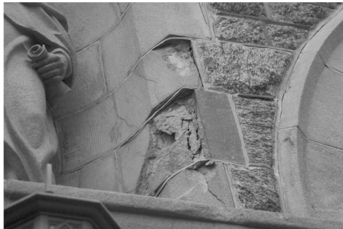
FIG. 7—Spalled limestone at alcove adjacent to granite.
