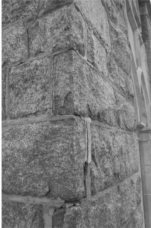
FIG. 2—Areas of previous mortar joint repointing that were applied too thin and have deteriorated.
