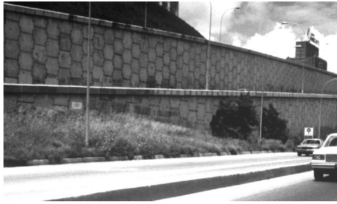
Figure 6.32 Reinforced earth walls (Caracas, Venezuela).
