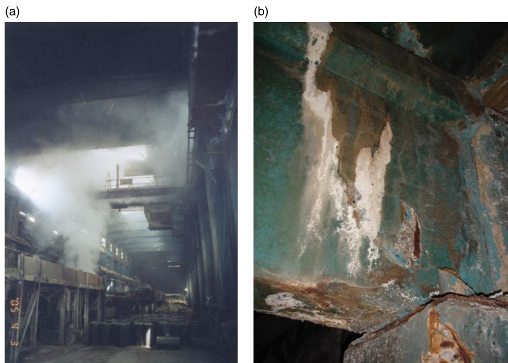
Figure 1.2 Advanced deterioration of concrete elements in a steel process workshop constructed in 1980, aged 24 years at inspection. The RC elements in the steel workshop were exposed to high concentration of corrosive gas rich in chloride and sulfate, high temperature, and humidity (a). The local degradation was manifested through advanced corrosion of steel bars, concrete spalling, and leachates from concrete cracks (b). Source: courtesy of Tingyu Hao.
