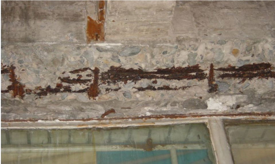
Figure 1.1 Rebar corrosion of RC slabs in a fine-art gallery of age 38 years by concrete carbonation. The building was constructed in 1962 with C25 concrete for the RC beams. The concrete binder is ordinary Portland cement (OPC), and the building was exposed to a rather dry environment with average temperature of 11 °C and average humidity of 57%. Source: courtesy of Tianshen Zhang.
