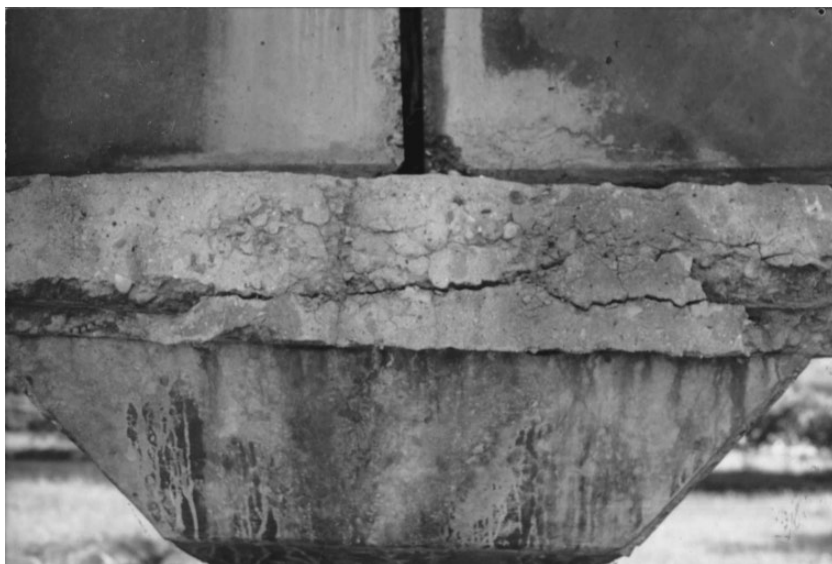
Figure 2.2 Urban viaduct affected by deicing salts. The solution of deicing salts infiltrated to the pier cap and induced advanced corrosion of the embedded reinforcement steel. The structure was 12 years old at inspection. The concrete grade was C30 for the pier cap, and the deterioration is typical for waterproof failure followed by deicing salts attack. Source: courtesy of Peixing Fu.
