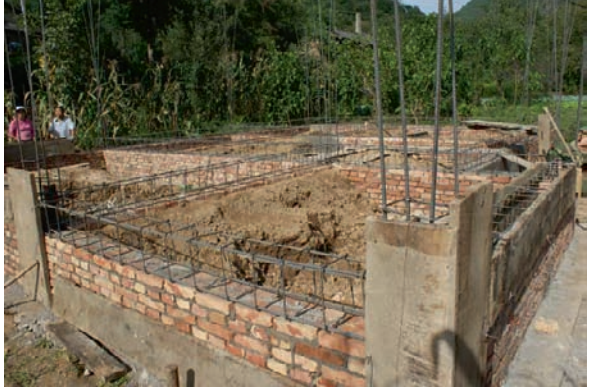
Fig. 53 A newly built house for post-disaster construction in the Kangxian county of Gansu province
