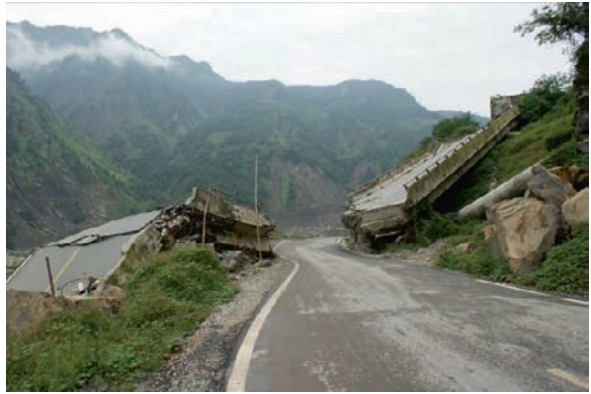
Fig. 23 The Duwen highway, which connects the Dujiangyan city and the Wenchuan county, was completely destroyed
