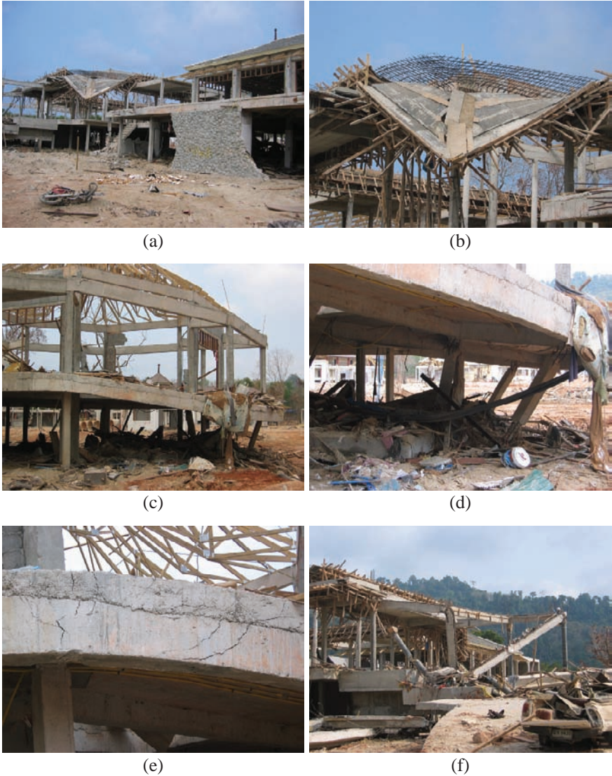
Fig. 3 Damage to reinforced concrete frame building under construction in Nai Thon Beach, Thailand
