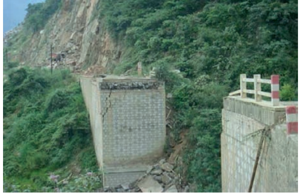
Fig. 27 The Luoxuangou bridge, which connects the Wenxian county of Gansu province and the Guanyuan city of Sichuan province, in Wenxian county
