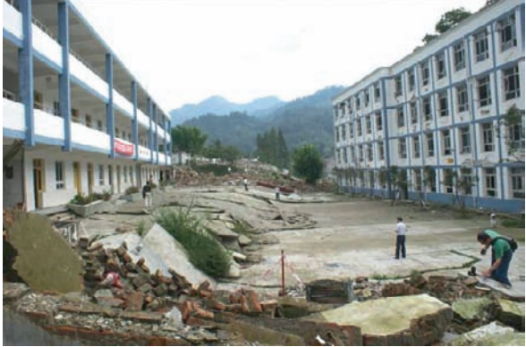
Fig. 36 A rupture crossed between two buildings of the Bailu high school
