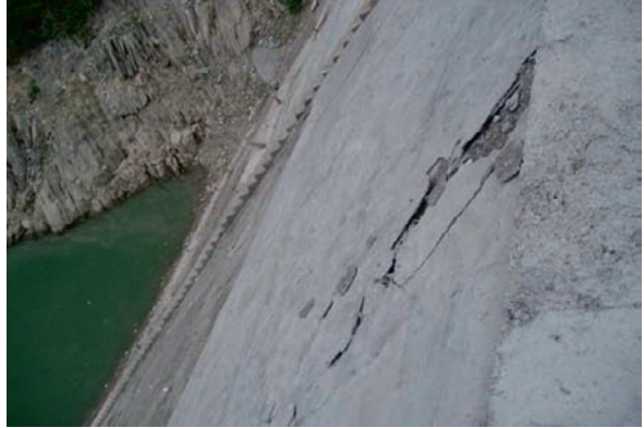
Fig. 29 Damage to the Bikou reservoir in Wenxian county
