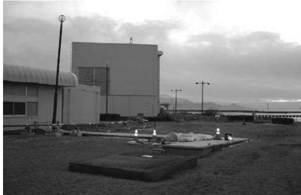
Fig. 8 Settlements of the ground at the site of nuclear power station
