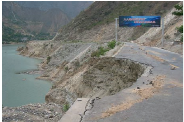
Fig. 24 A subsidence with 10 m long and 3 m wide in the G212 highway
