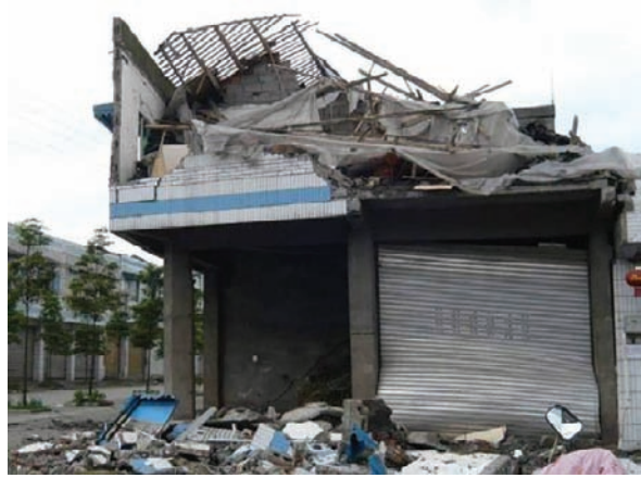
Fig. 17 The building with the top floor destroyed in Guangji town, Mianyang city
