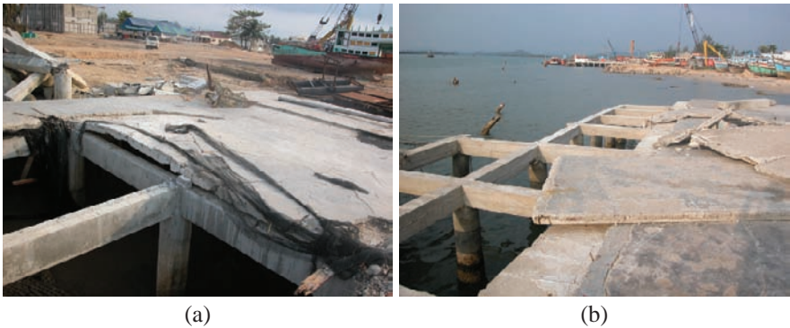
Fig. 5 Damage to precast slab strips of the concrete dock in Khao Lak, Thailand
