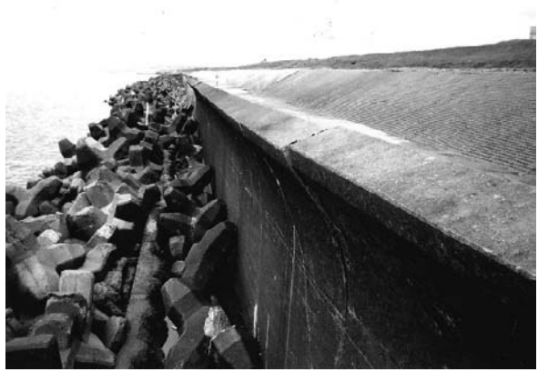
Fig. 15 Stacks of wave-braking blocks and parapet wall displaced about 1.0–1.5 m seaward at Kitazono area
