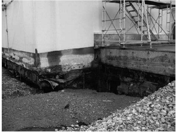
Fig. 10 Depression of the ground in the vicinity of the building
