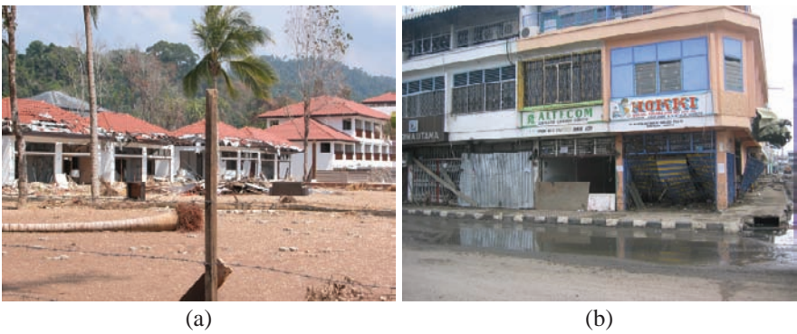
Fig. 7 Non-engineered concrete frames that survived the tsunami; (a) Khao Lak Beach, Thailand and (b) Banda Aceh, Indonesia
