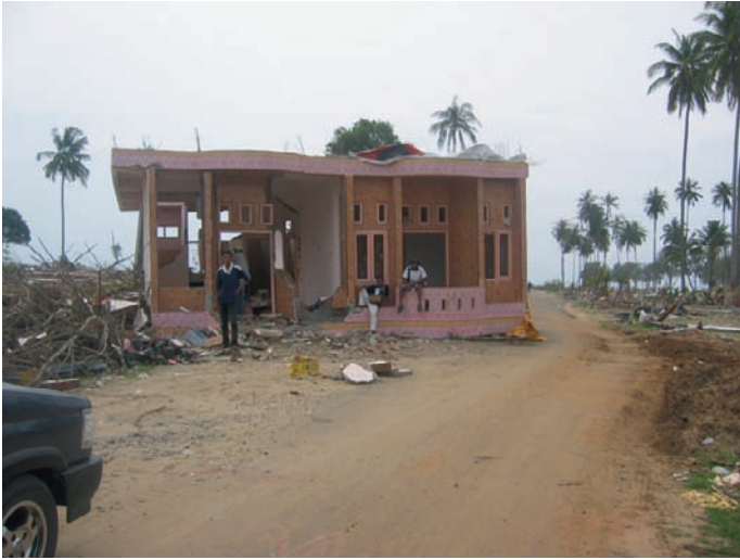
Plate 16 A single-story house, displaced by water pressure due to lack of proper anchorage, Banda Aceh, Indonesia (See also Fig. 13 on page 164)
