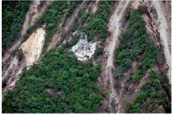
Fig. 30 A power transmission tower was damaged. (From Xinhuanet, 2008)
