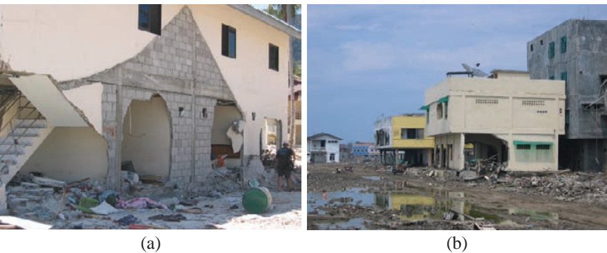
Fig. 9 Typical punching failure of masonry walls; (a) Phi Phi Island, Thailand; (b) Banda Aceh, Indonesia
