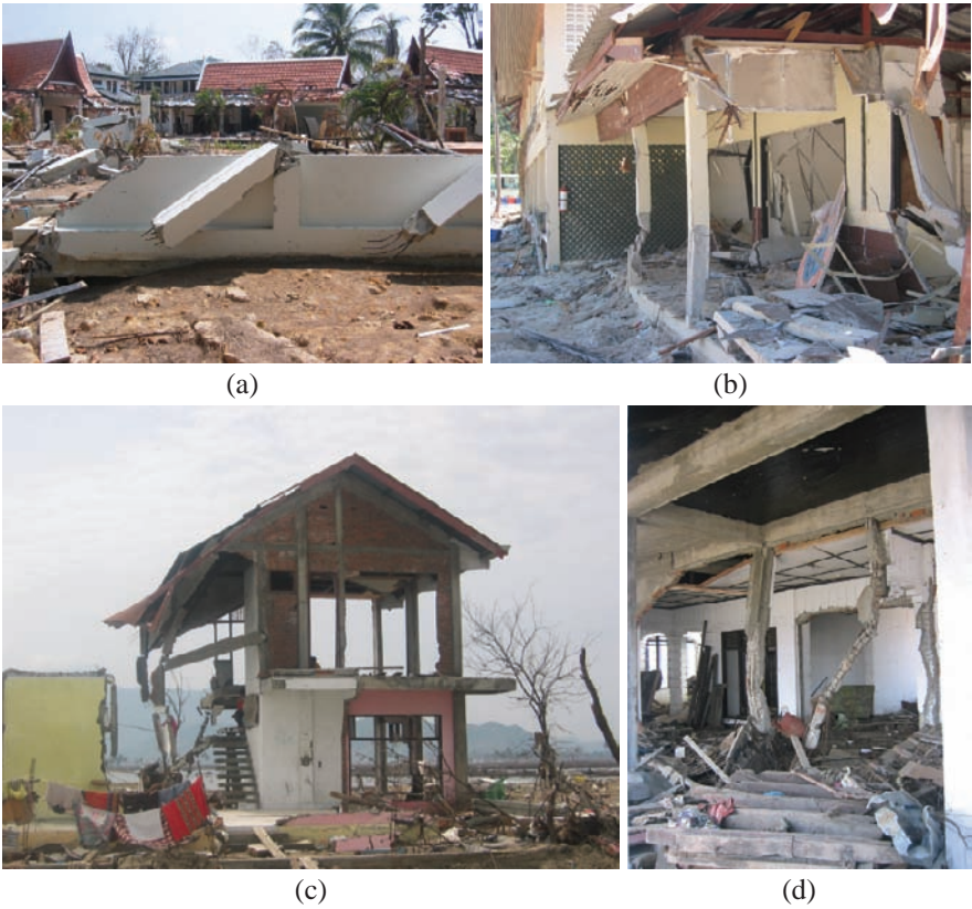
Fig. 6 Damage to non-engineered reinforced concrete; (a) Phuket, Thailand (b) Phi-Phi Island, Thailand, (c) and (d) Banda Aceh, Indonesia
