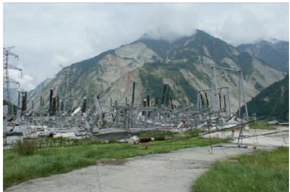
Fig. 31 A power substation was damaged in Yingxiu town, Wenchuan county
