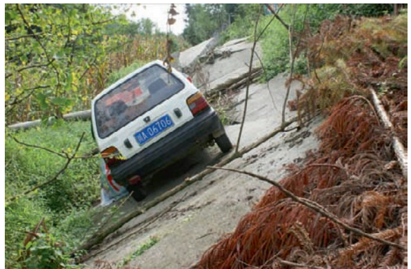
Fig. 35 Uplifted of a county road in Hongkou, Dujiangyan city
