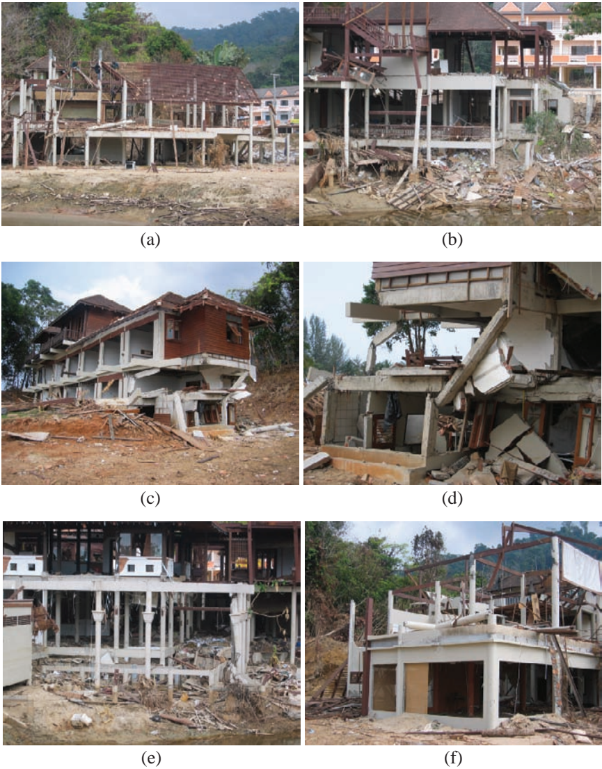
Fig. 2 Damage to reinforced concrete frame buildings in Nai Thon Beach, Thailand (See also Color Plate 15 on page 214)
