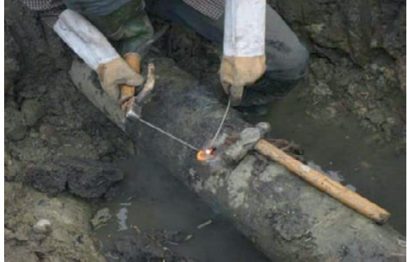
Fig. 32 A water supply pipe was broken after the earthquake (From Yuan Yifan, 2008)
