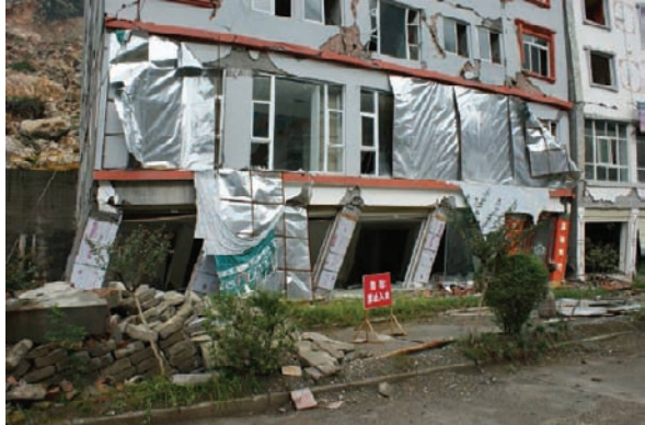
Fig. 19 A building in Beichuan county, which the first floor was destroyed and the upper floors were heavily damaged
