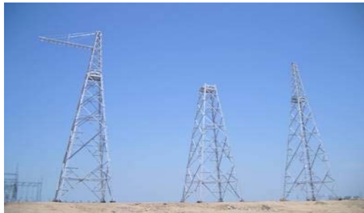
Exhibit No.28: Angle Tower consisting of one structure per phase
