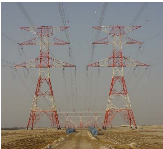
Exhibit No. 20: Two 400 kV lines installed with common access road
