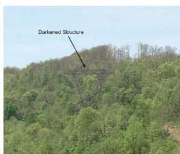
Figure 17: Darkened steel structure.
