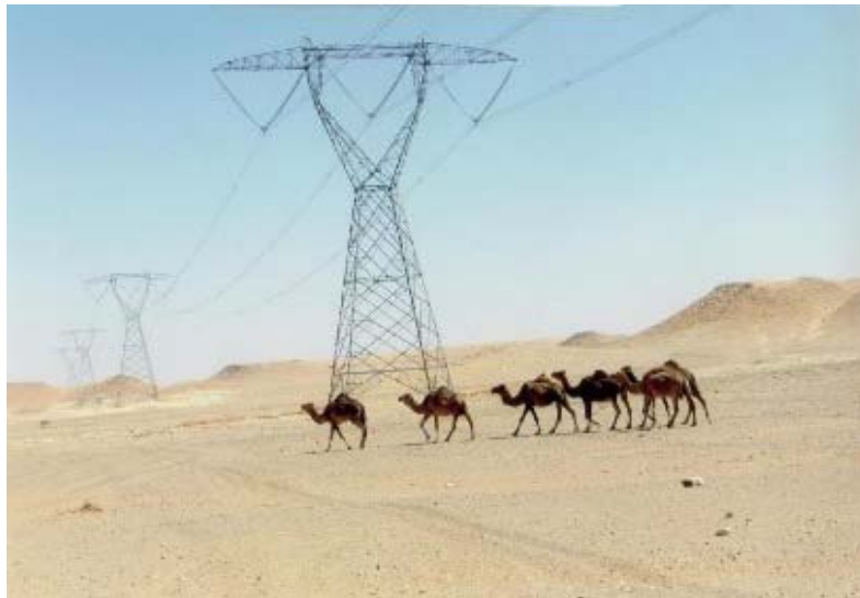
Exhibit No.31: 400 kV S/C transmission line in Sahara Desert
