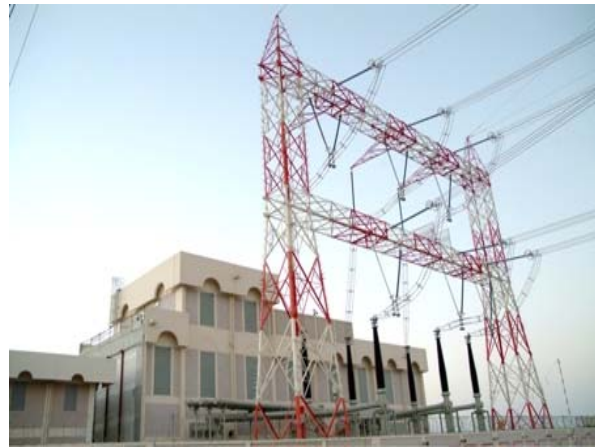
Exhibit No. 18: Double-deck gantry near GIS substation
