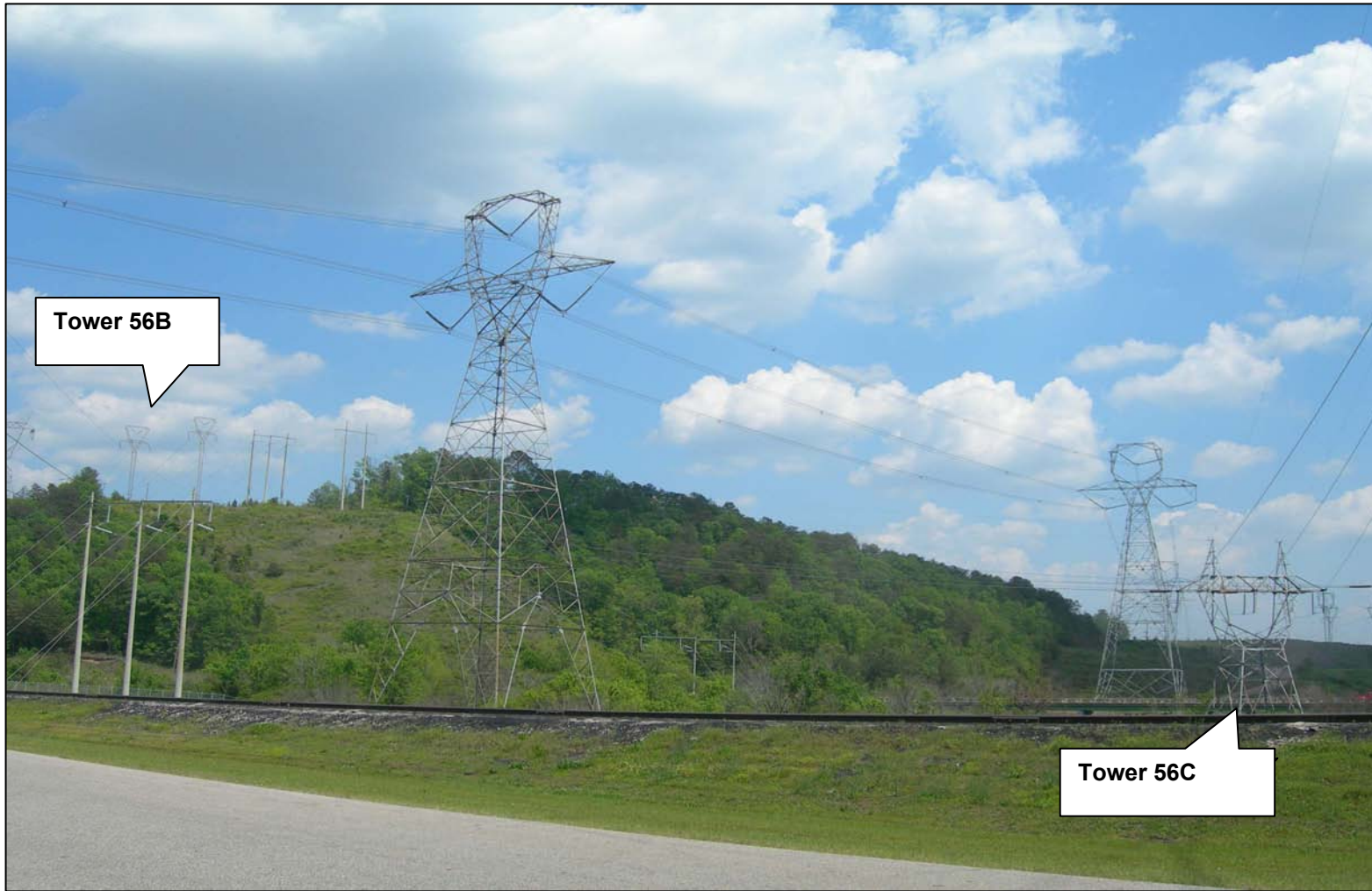
Figure 3: Conductor in Span C crossing 230 kV and 500 kV transmission lines
