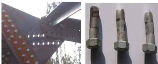
Failure at Connection B
