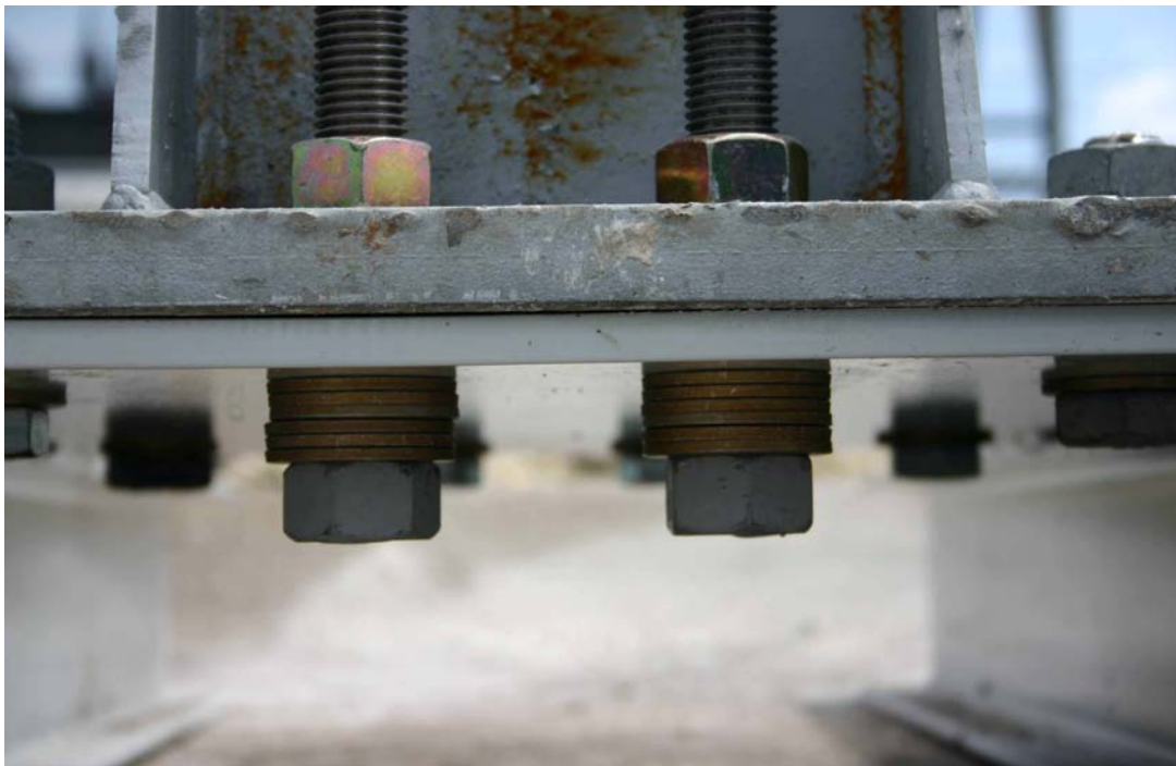
Figure 4b Dead-End Tower Bolted to Steel Base
