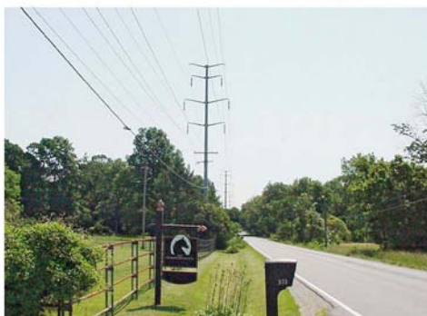
Figure 21: Double circuit 138kV with distribution underbuild attached.
