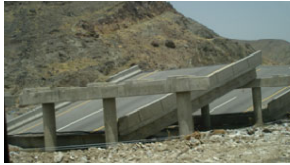
Exhibit No. 9: Damaged Bridge
