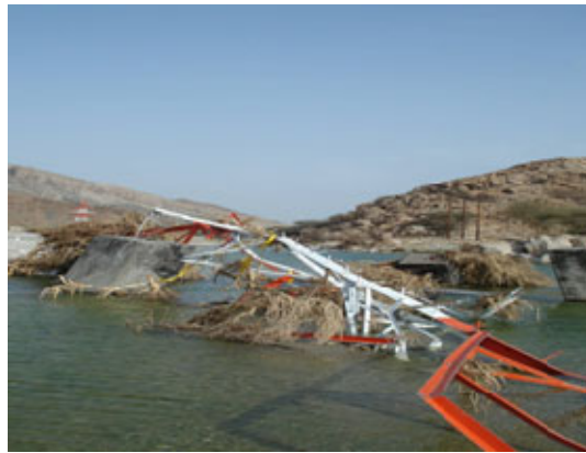
Exhibit No. 6: Damaged tower
