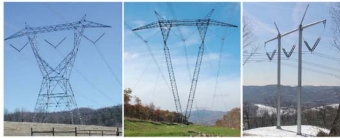
Figure 10: AEP 765kV transmission structures: self-supporting lattice; guyed-v lattice; and tubular pole. Structure type is chosen based on topography, land use, land cover, and construction access.
