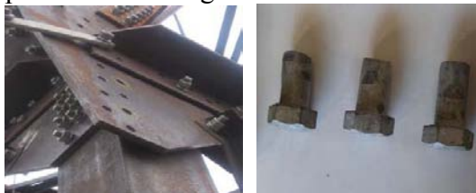
Failure at Tower Waist – Connection A
