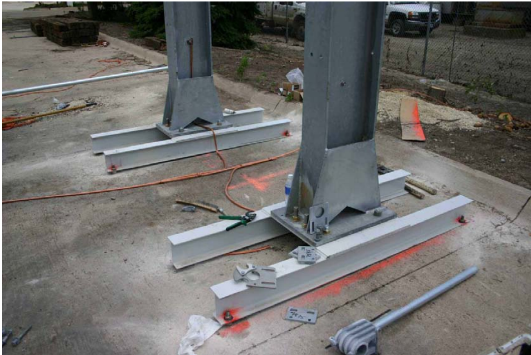
Figure – 4a Dead-End Tower Base
