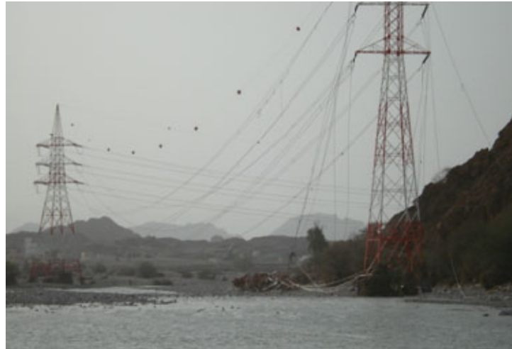
Exhibit No. 4: Conductors are grounded
