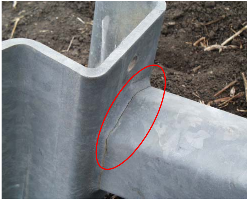
Figure 1 – Cracked Davit Arm
