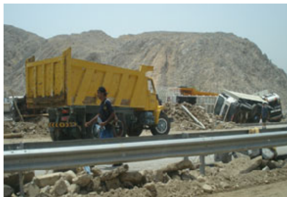
Exhibit No. 8: Damaged Highway
