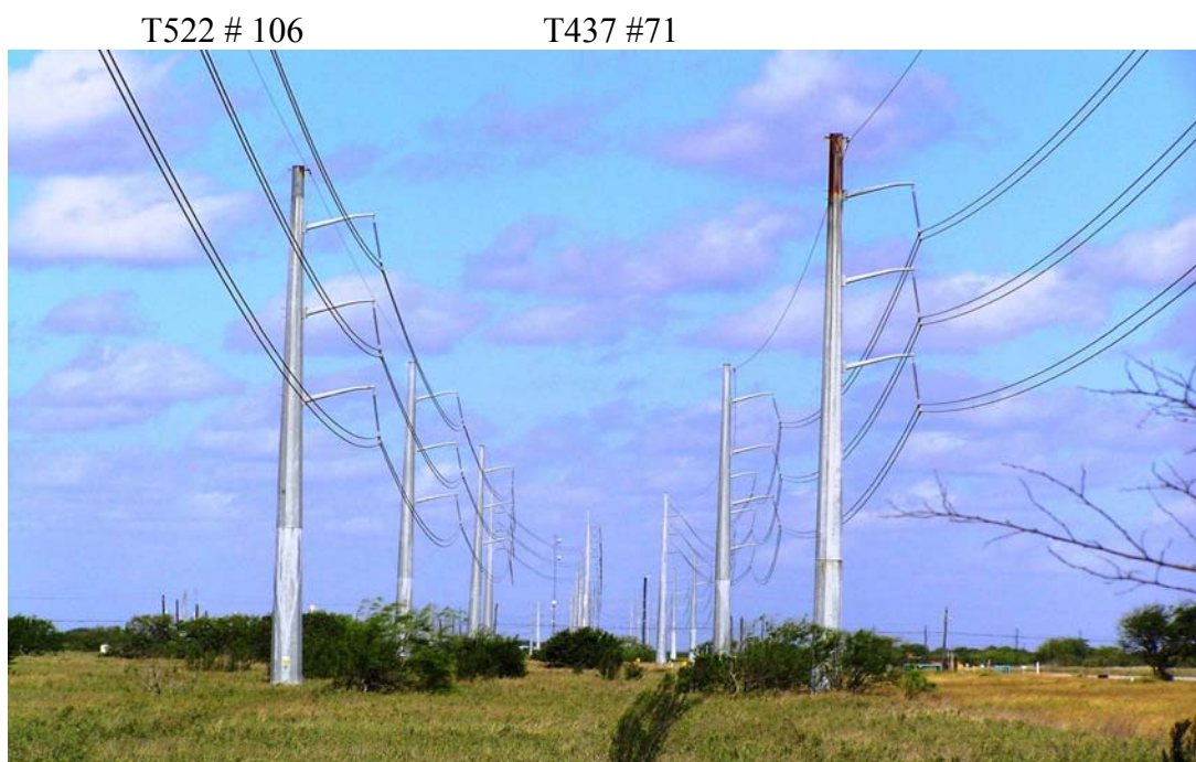
Visible Corrosion on Two Steel Poles
