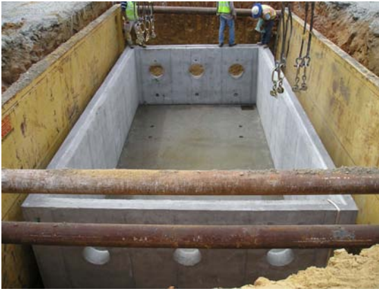
Figure 12. Trifurcating Manholes at Topeka
