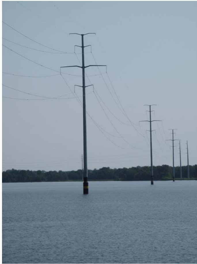
Figure 7 - Lake Fork Crossing Structures
