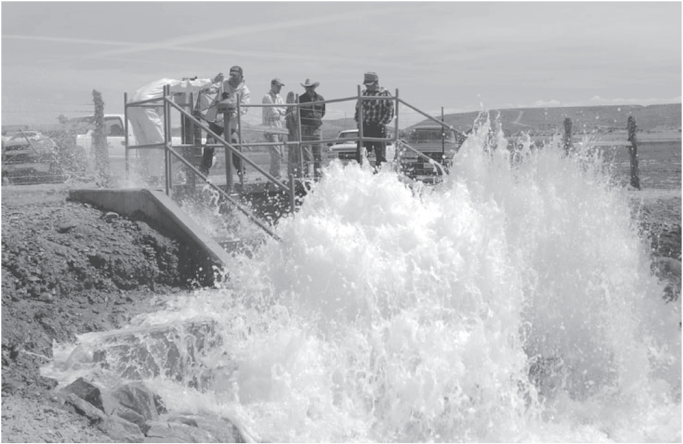
Figure 6.5 Intense splashing due to insufficient space between the conduit outlet and hanging baffle [Figure 54 in Outlet Works Energy Dissipators published by the United States Federal Emergency Management Agency (FEMA) (FEMA, 2010)].
