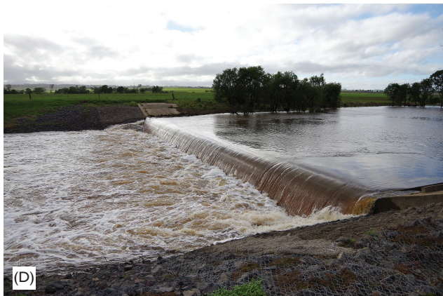
Figure 7.2 Spillway systems and operation. (A) Hinze dam spillway Stage 3 (Australia) in operation on 29 January 2013 ( Q = 200 \text{ m}^3/\text{s} ), view from upstream with a stepped chute in foreground, followed by a stilling structure, turning veins, long chute and flip bucket. (B) Intense air entrainment at Three Gorges Project (China) on 20 October 2004 ( V = 35 \text{ m/s} , shutter speed: 1/1,000 \text{ s} ). (C) Sediment deposits in Jiji weir stilling basin (Taiwan) on 11 January 2014 during cleanup. (D) Joe Sippel weir (Australia) on 5 March 2013 after a very large flood event, with a plunge pool/hydraulic jump on the stepped chute in the foreground.
