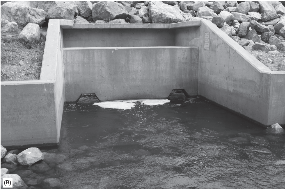
Figure 6.1 Examples of hanging baffle dissipators: (A) Julius Park Reservoir (UT, USA) (courtesy of Bret Dixon, Utah Division of Water Rights Dam Safety Program), (B) Lost Lake (UT, USA).
