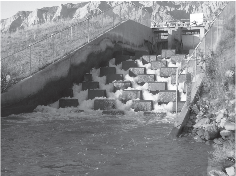
Figure 6.10 Example of a baffled chute canal drop structure near Willard, Utah, USA.
