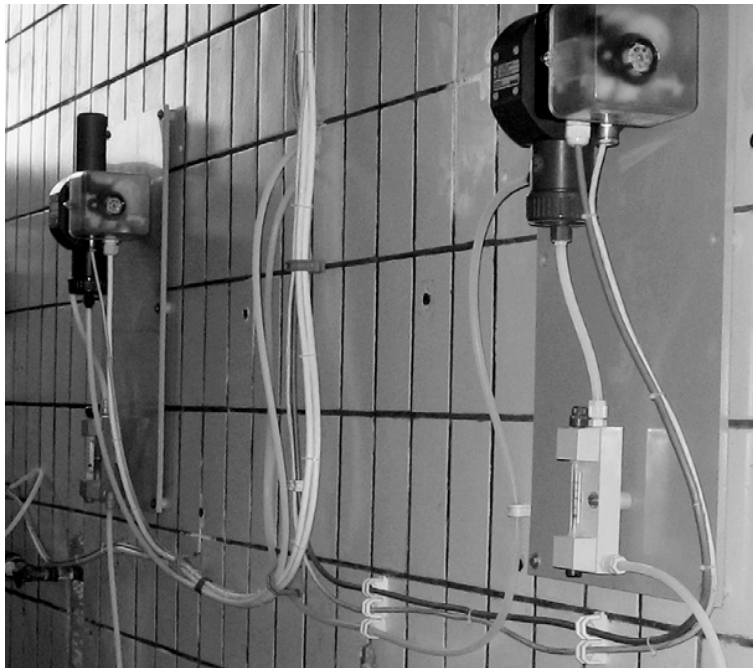
FIGURE 9-19 Automated chlorination device.
