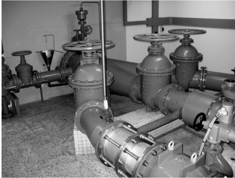
FIGURE 9-25 Large diameter pipes and valves used to divert water in different directions.
