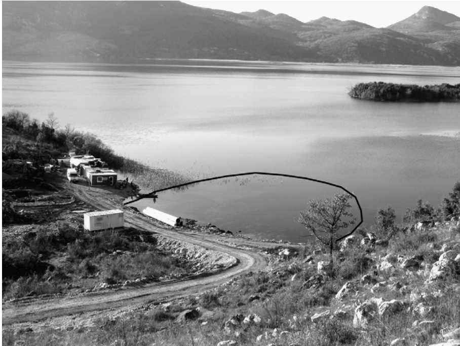
FIGURE 10.5-18 Bolje Sestre tapping structure under construction in December 2008. The curved line approximates the position of the future coffer dam.
