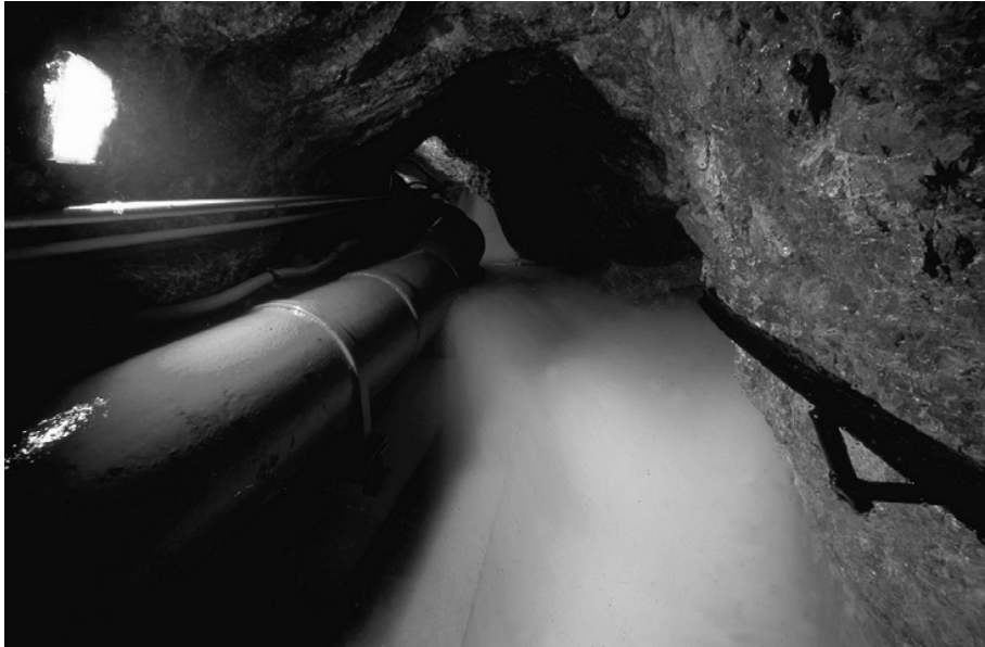
FIGURE 10.2-13 Large Kläffer (background) drains directly into the gallery. Photo taken during high water condition.
