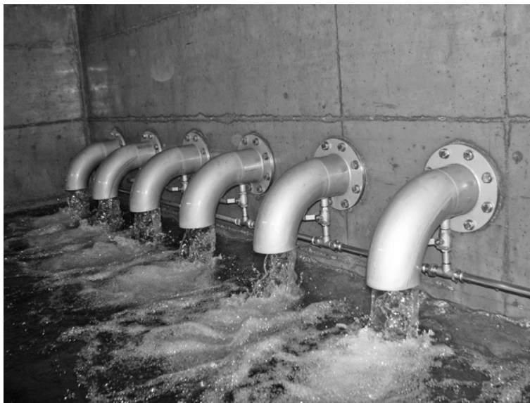
FIGURE 5-22 The Cossaux spring used for water supply of the city of Yverdon-les-Bains in western Switzerland. A detailed description of the spring is given by Pronk et al., 2005 . (Photograph courtesy of Nico Goldscheider.)
