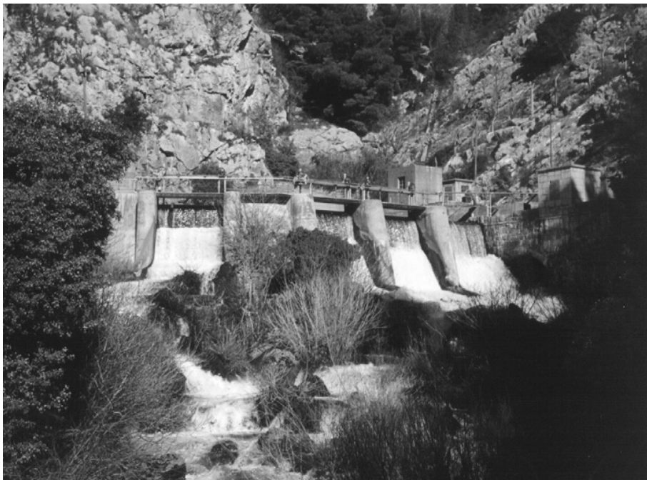
FIGURE 1–14 The Jadro Spring, initially tapped by Roman emperor Diocletian in 3rd century AD, is still used for water supply of the Croatian port city of Split. (Photograph courtesy of Ivana Gabric).
