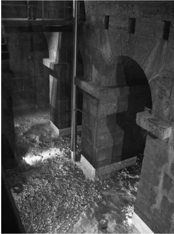
FIGURE 9-4 Detail from Kaiserbrunn spring (Rax Mt. near Vienna), a masterpiece of spring capture design and quality from the 19th century.
