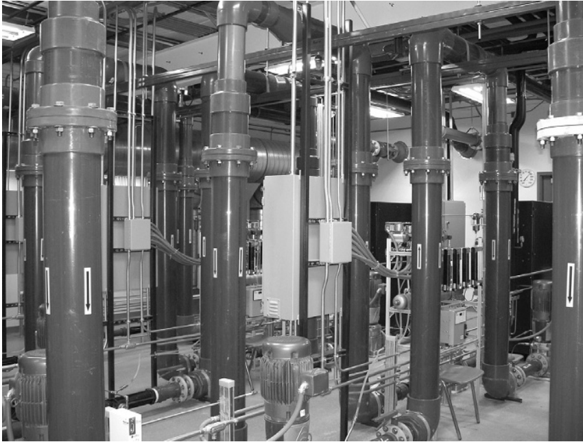
FIGURE 7-12 Full-scale advanced oxidation and ozone treatment system for flow rate of 1300 gpm. Design and engineering Farsad Fotouhi, Pall Corporation.
