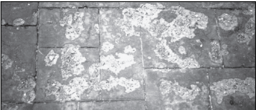
Figure 11: Damage of the concrete pavement surface by the effect of frost and of defrosting salts causing dilatation.
