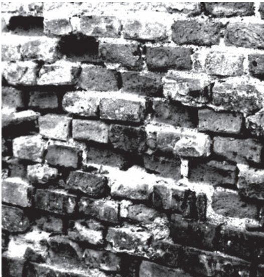
Figure 2: Brick masonry damaged by frost.
