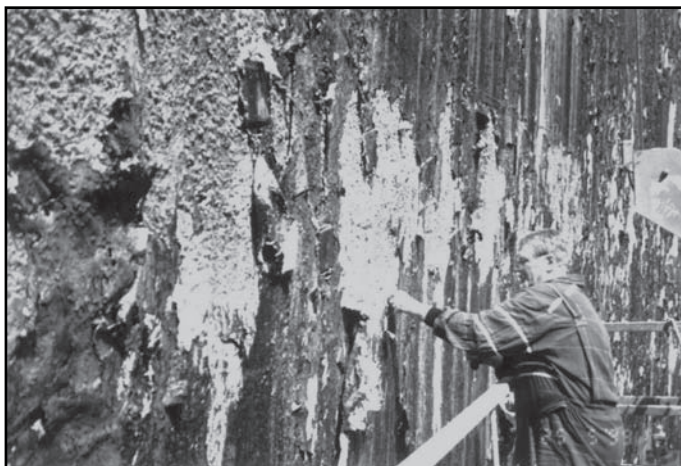
Figure 23: Completely damaged and non-functional paint of the interior part of the tower (Photo: R. Kepák).
