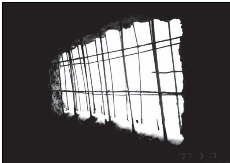
Figure 21: View of a cooling tower wall where, owing to the marked effects of carbonation, humidity and less compactness, the concrete crumbled and the so-called ‘windows’ originated.
