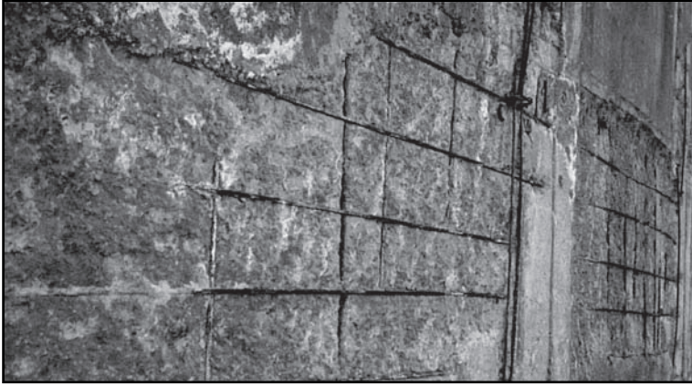
Figure 5: View of reinforced concrete wall considerably damaged by the joint effect of carbonation and sulphation. The building is in an industrial centre with high content of \text{SO}_2 in the air. (Photos without quoted names of photographer are taken from the authors' archives.)
