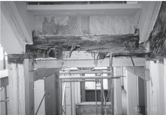
Figure 9: Damage to leaky condominium in Vancouver, Canada, due to rotting wood. (Photograph courtesy of Levelton Engineering Ltd., Richmond, BC.)
