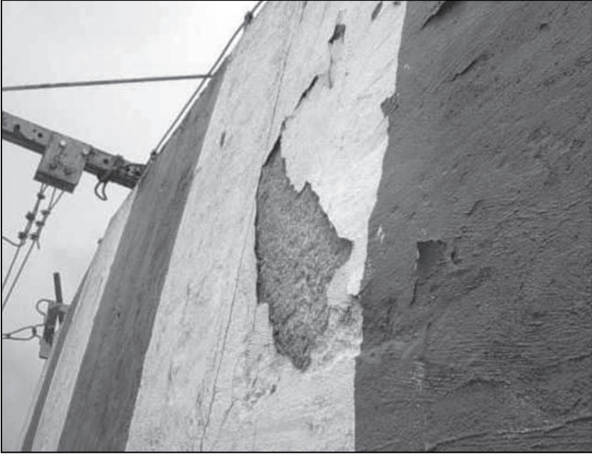
Figure 42: Detailed view of the gallery of the top part of a cooling tower exhibiting damaged red and white painted stripes based on epoxy resins. When this kind of paint is used, overall spalling occurs due to the damage of the concrete under the paint caused by the freezing-thawing action. A role is also played by the deterioration of the polymer material by UV radiation.
