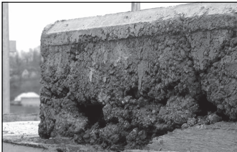
Figure 27: Extreme case of the effect of extracting rainwater. Concrete wall damaged by water flowing out for a long time from a broken pipe discharging precipitation water; poor compaction also had an effect.
