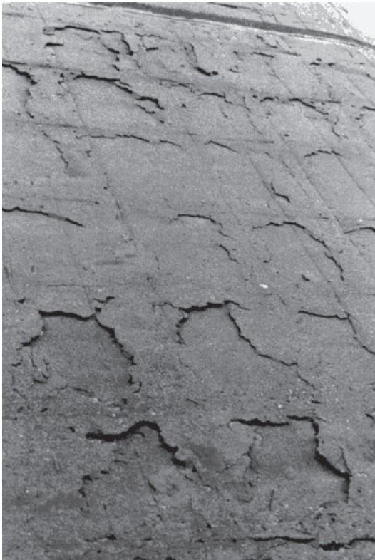
Figure 8: Crack pattern due to corrosion induced by carbonation.
