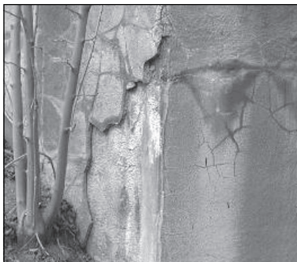
Figure 34: View of the bridge pillar corner. The damage was caused by precipitation and re-crystallisation of the calcium constituents of concrete. The high content of chlorides in water leakage into the concrete also contributed to the extract.
