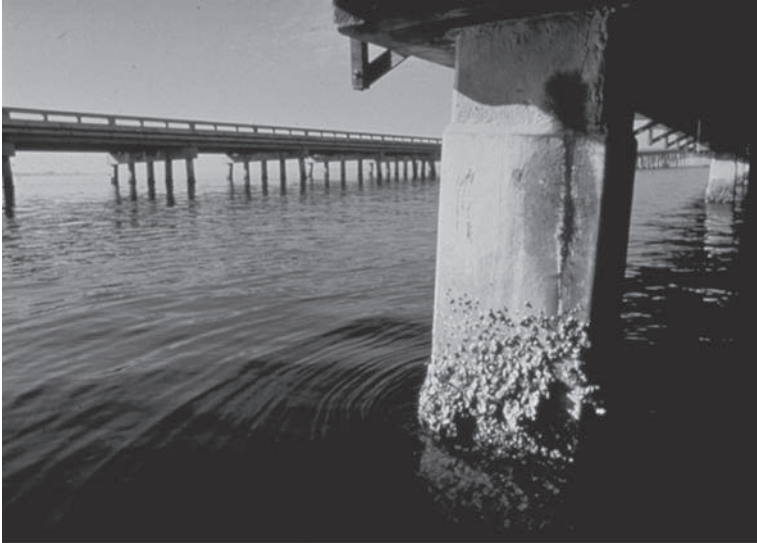
Figure 9: Concrete pier showing signs of reinforcement corrosion (Courtesy: N. Berke).
