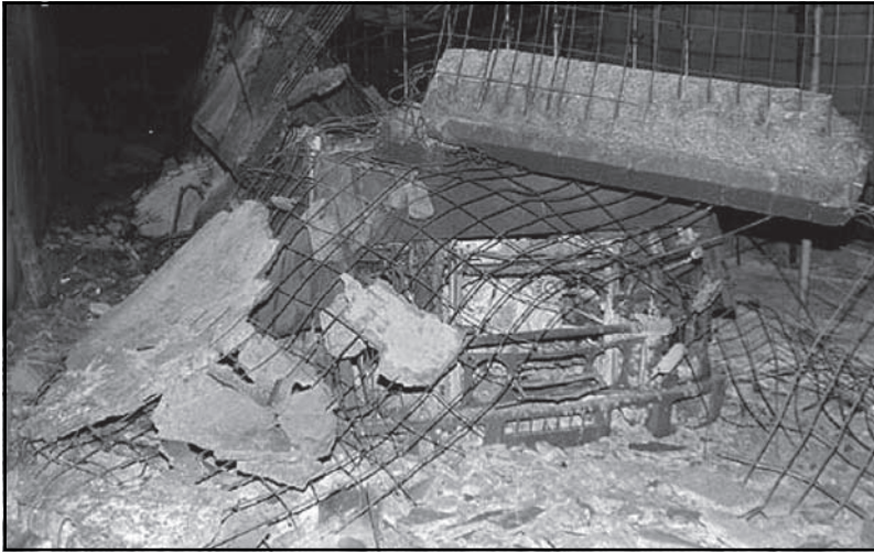
Figure 35: During a fire in a tunnel, the tunnel is completely disintegrated owing to high temperatures that may reach a maximum of 1400°C. The picture shows a warped reinforced vault made of shotcrete (Photo: J. Horvath).
