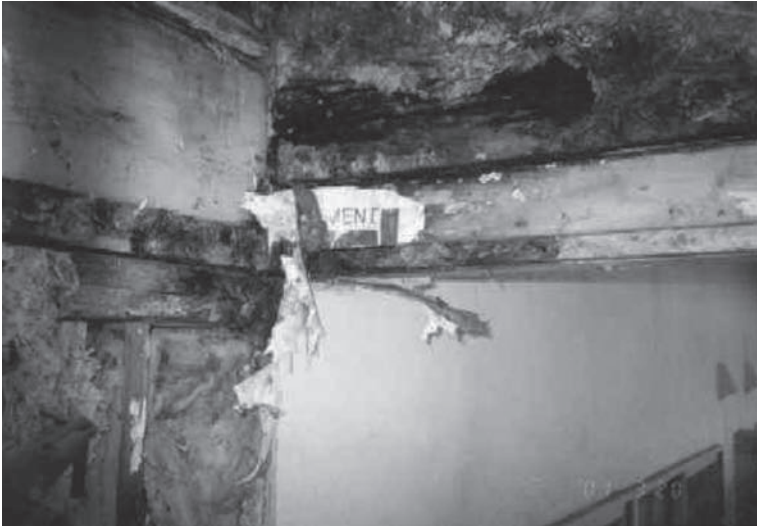
Figure 10: Rot observed in wall during recladding of structure. (Photograph courtesy of Levelton Engineering Ltd., Richmond, BC.)
