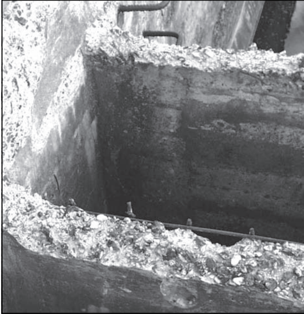
Figure 26: Concrete deterioration of the catch basin in a chemical plant.
