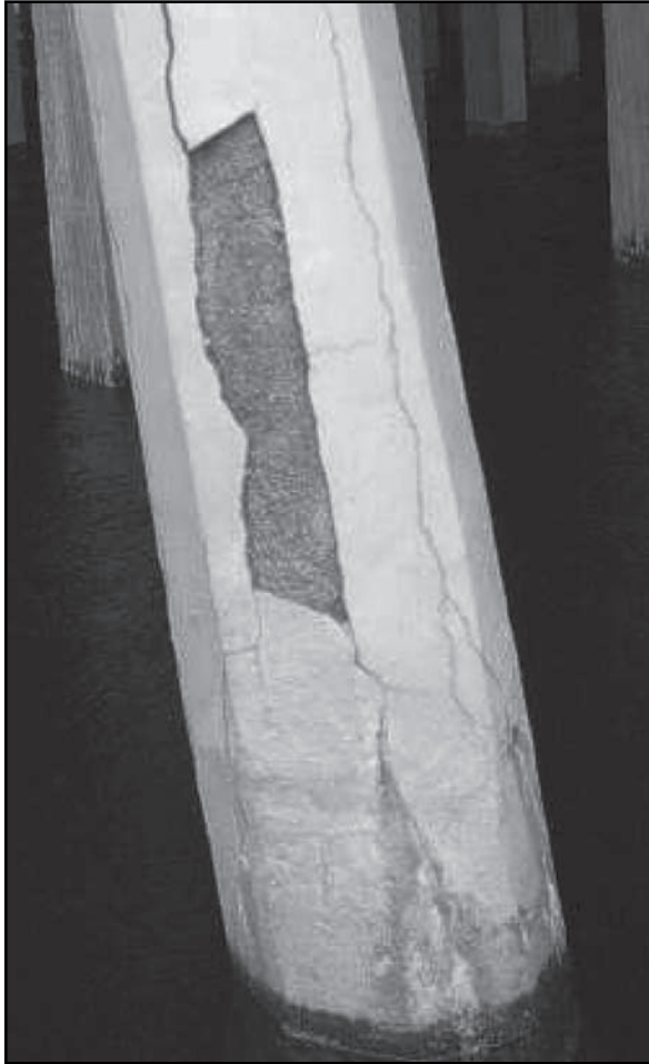
Figure 22: Frost damage of the concrete cover of stanchions (columns) supporting the whole structure of a cooling tower. The stanchions are fixed-ended in a foundation plate flooded with water.
