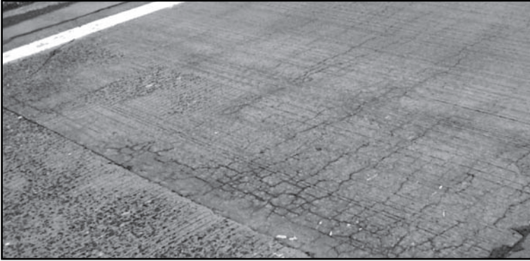
Figure 29: View of a road where concrete failure by alkali expansion was detected.
