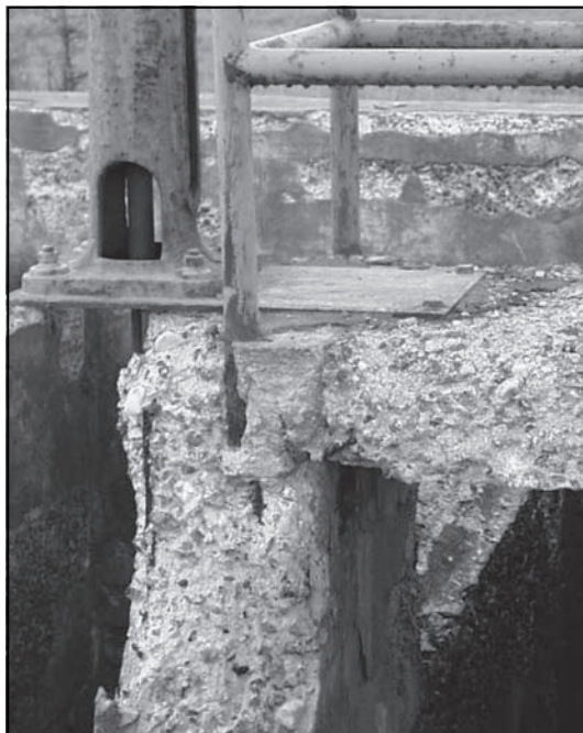
Figure 25: View of a completely damaged wall of one of the pits in a wastewater treatment plant (Photo: J. Hromádsko).
