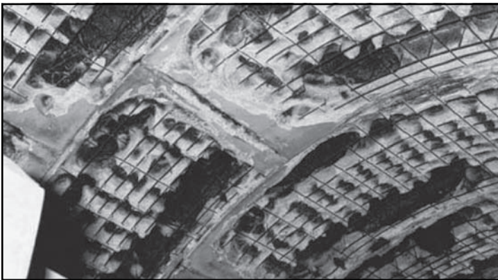
Figure 37: General view of a tunnel vault without concrete surface layers damaged by fire (Photo: J. Horvath).
