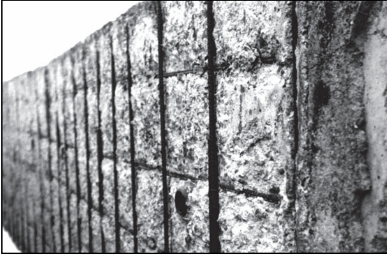
Figure 20: View of the upper part of a cooling tower wall that deteriorated owing to the effects of carbonation, humidity and insufficient compactness.
