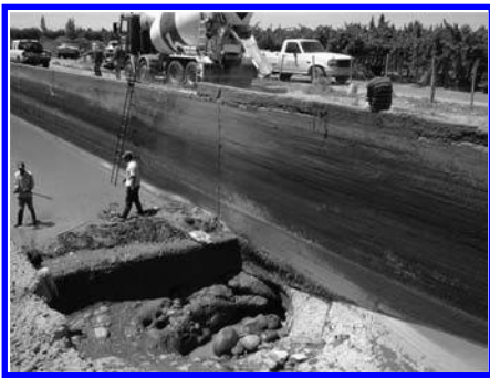
Figure 6. Hole aside the bottom step.
