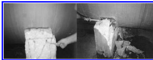
Figure 3. Damage in some supports (Almeida & Ramos, 2009).
