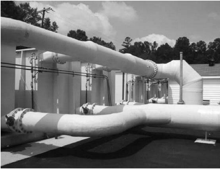
Fig. 15.3. BIOREM multiple biofilter treatment system. (Photograph courtesy of Biorem Technologies, Inc., Guelph, Ontario, Canada)
