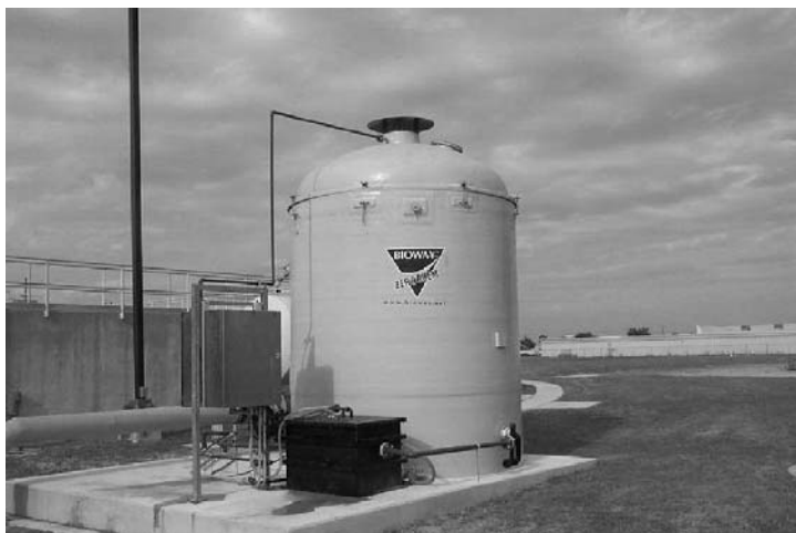
Fig. 15.8. Bioway intermittent trickling filter odor control system. (Photograph courtesy of Bioway America, Inc., Marlton, NJ)
