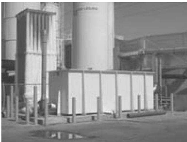
Fig. 1.1. A biofilter treating 2000-acfm air containing industrial odor emissions at Detroit, Michigan. (Courtesy of BIOREM Tech., ON, Canada)
