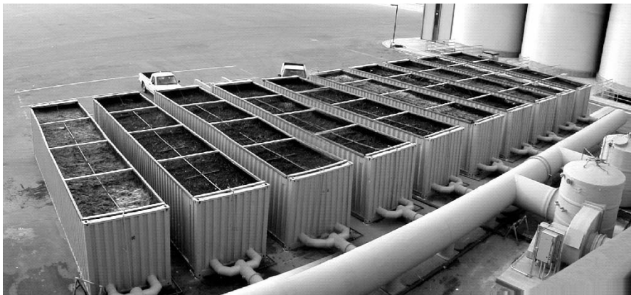
Fig. 15.7. Los Angeles County Sanitation District multiple biofilter arrangement to treat off-gases from a biosolids handling facility. (Photograph courtesy of the Los Angeles County Sanitation Districts, Los Angeles, CA)
