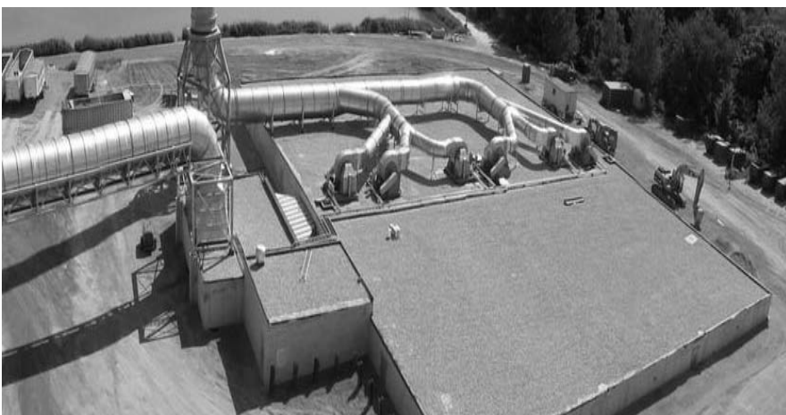
Fig. 10.2. A 250,000-cfm synthetic media biofilter system treating air emissions from a rendering plant. (Courtesy of BIOREM Technologies, ON, Canada)
