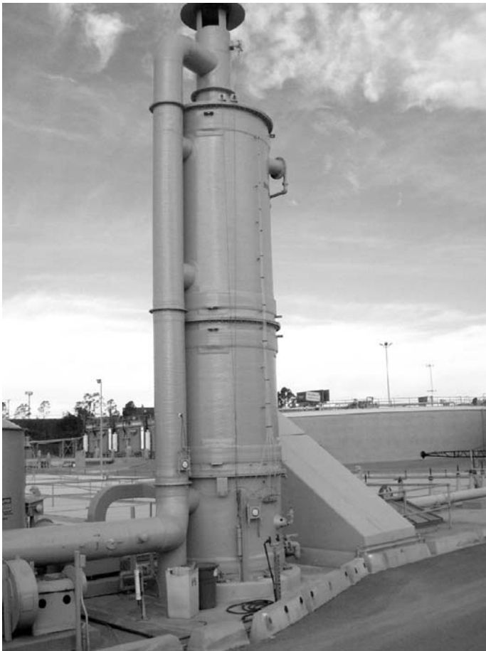
Fig. 15.9. Los Angeles County Sanitation District biotrickling filter reactor for odor removal. (Photograph courtesy of the Los Angeles County Sanitation Districts, Los Angeles, CA)
