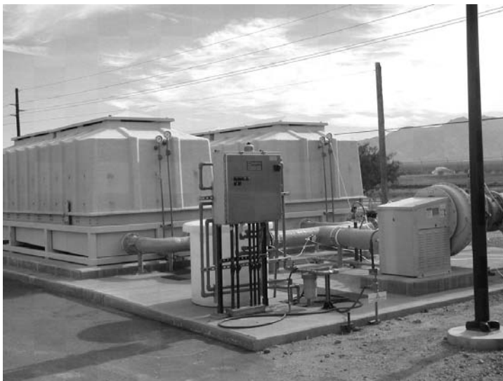
Fig. 15.2. Shaw Environmental dual P-600 biofilter assembly treating headworks off-gases. (Photograph courtesy of Shaw Environmental, Inc., Baton Rouge, LA)
