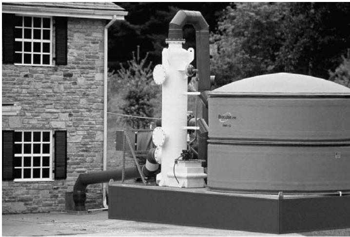
Fig. 15.6. Biocube biofilter system treating low flow waste gases. (Photograph courtesy of Biocube, Inc., Victor, NY)
