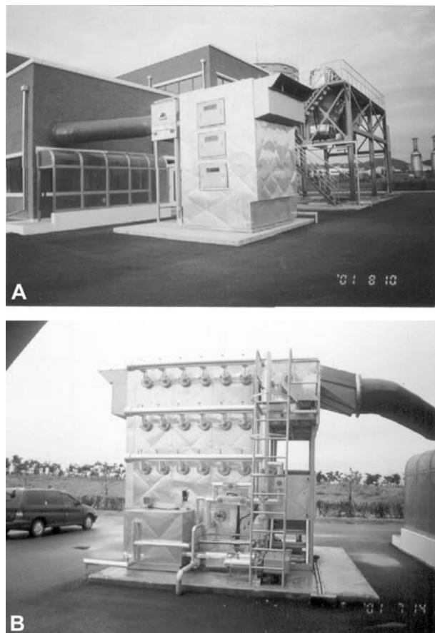
Fig. 14.2. Trickling bioreactors manufactured by Han-Ki Industrial Ltd., RK. Model BioCat-50/250-I 12,000 m 3 h -1 installed at water treatment plant in the town of Pusan. Recommended EBRT 2.0–3.0 s. A Front view; B rear view
