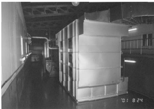
Fig. 14.3. Trickling bioreactors manufactured by Han-Ki Industrial Ltd., RK. Model BioCat-100/500-II 30,000 \text{ m}^3 \text{ h}^{-1} at the Kayang sewage treatment plant, Seoul. Recommended EBRT 2.0–3.0 s
