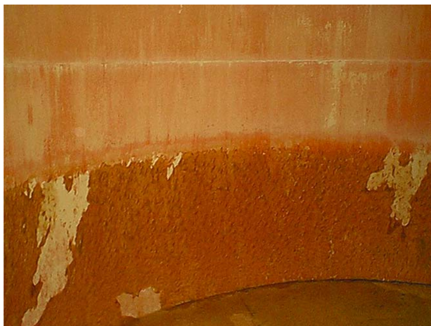
Figure 4 Bacterial biofilm inside a water storage tank.
