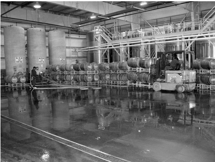
FIGURE 2.6. Work floor, tanks, and catwalks.
