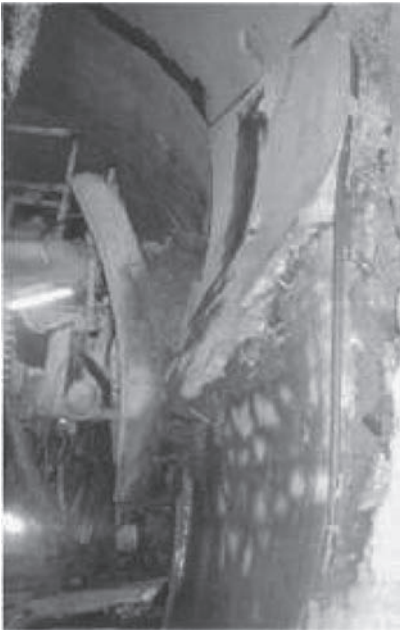
Figure 5. Failure in the Aicha Tunnel, breakage of the left-hand shotcrete lining.
