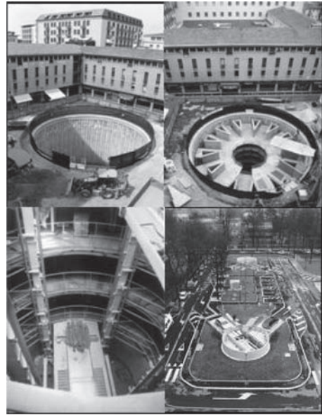
Figure 1. TreviPark construction sequence: secant piles retaining wall and excavation, placing of prefabricated internal structures, installation of car lift and final urban facilities.
