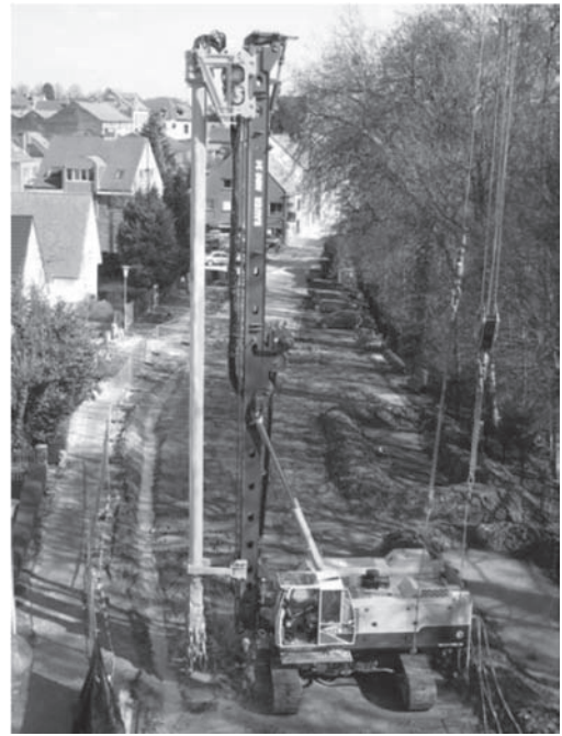
Figure 8. MBG 24 with Kelly guided SCM mixing head, executing a retaining wall, Meise, Belgium.
