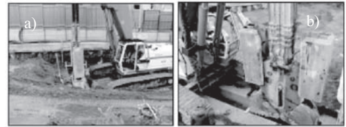
Figure 7. Pictures from the site in Napoli: different positions of the operating machine during panel excavation: a) on the long side; b) on the short side.
