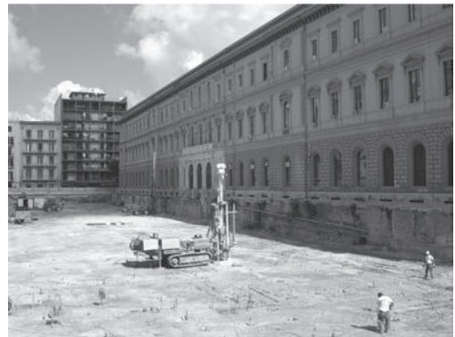
Figure 12. Drilling and grouting of the boreholes under the entire area to create a bottom plug.
