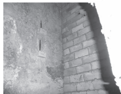
(c) WSN in Barcelona metro tunnel
