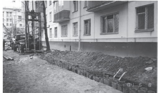
Figure 5. Erection of a cut-off diaphragm wall, made of bore steel pipes between the service tunnel and the existing building 61/67, Pochtovaya Str. in Moscow.
