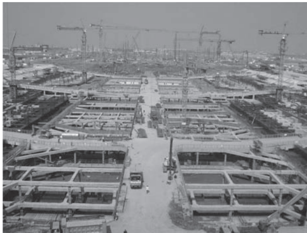
Figure 10. A photo of the construction site when the soil was cut to the final elevation.
