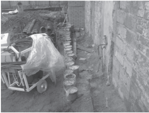
Figure 2. Geotechnical diaphragm wall for protecting the office building of the Vakhtangov Theater.
