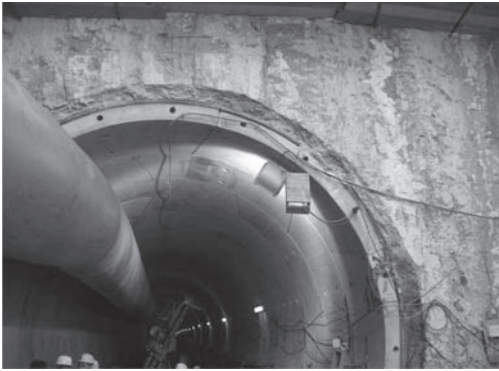
Figure 12. Photographs of the hardened back-filling at the contact between the station diaphragm walls and the tunnel.
