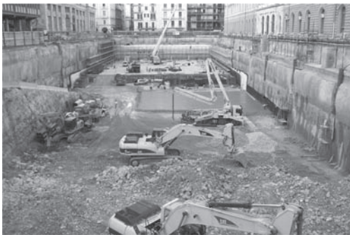
Figure 18. Excavation works, after the grouting treatment performed to consolidate and waterproof the foundation rock.
