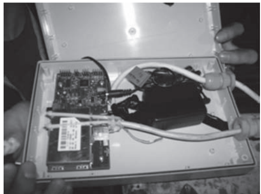
Figure 17. Wireless sensor network gateway connected with central point via Ethernet cable.
