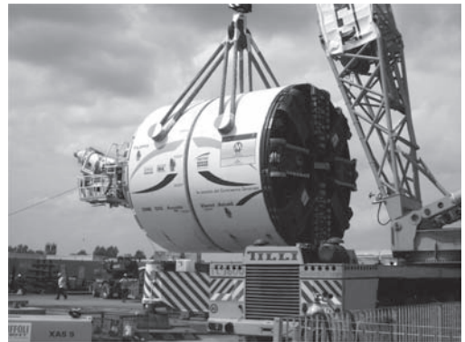
Figure 7. Photographs of the second EPB machine used for the excavation of the tunnels.
