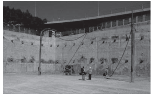
Figure 17. Situation after pumps activation.
