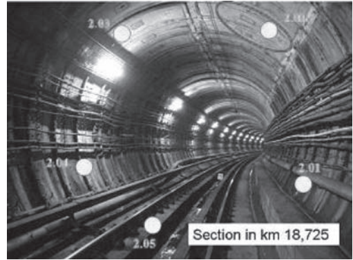
Figure 2. View of the test section 1, direction Vltavská station (tilt plates and convergence bolts are presented by yellow circles and cracked lining segment by red ellipse where crackmeters, geophones and inclinometers are installed).
