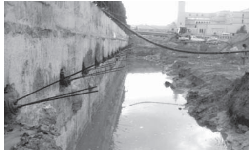
Figure 16. Situation before pumps activation.
