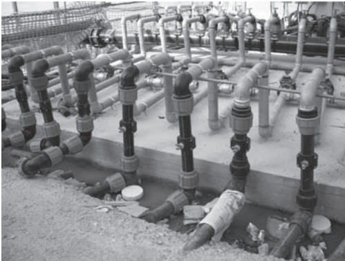
Figure 6. Picture of pumping system of the Mirti Station: flow meter and pipes.
