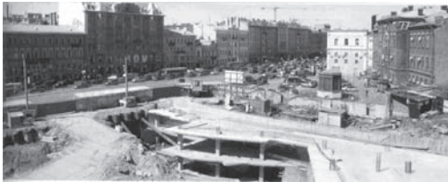
Figure 12. The construction of the underground part of the Trade Center at Ligovskii prospect.
