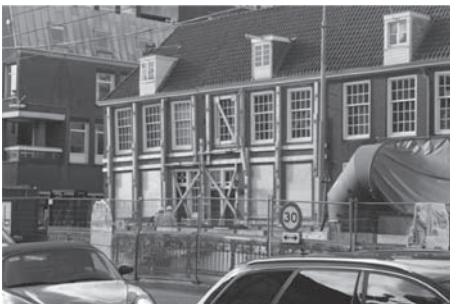
Figure 2. A timber framework was installed to stabilise the historical buildings after severe settlements.
