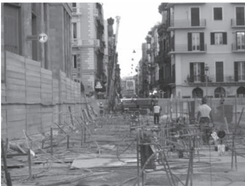
Figure 11. Grouting on the perimeter, to create an impervious grout curtain and to consolidate the walls of the designed excavation.
