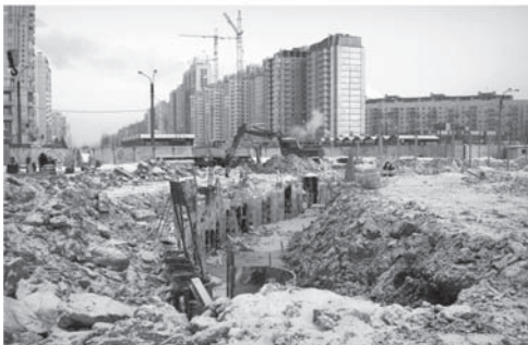
Figure 2. Initial trench made by “Wall in ground” method (a) and sheet pile immersion (b).
