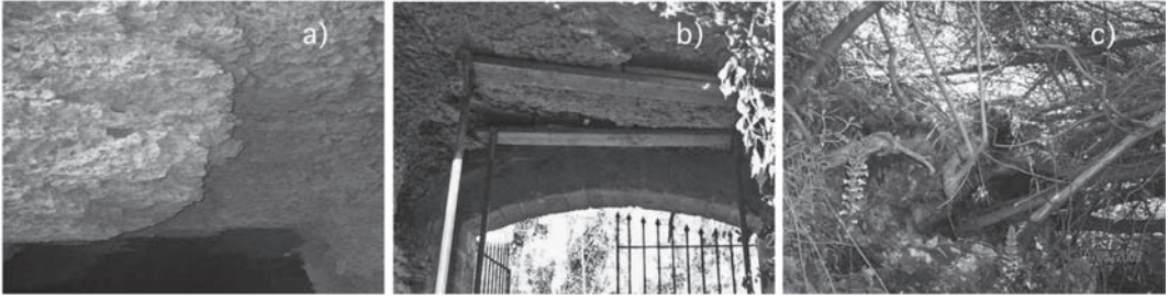
Figure 9. Rock mass decay phenomena: a) fall of slabs b) development of cracks c) fall due to the pull out of the roots.
