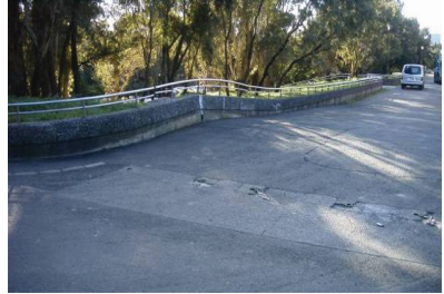
FIG.8. Distortion of road pavement on embedded pipe due to subsidence.
