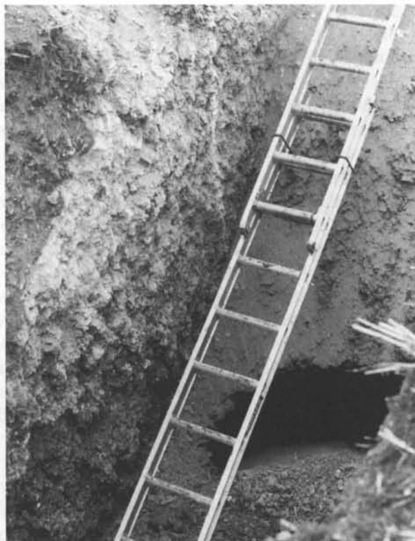
Fig. 3.2 Section through a void in granular soil exposed in the side of a trial trench at Littleheath Road, West Sussex, UK, after Matthews et al. (2000b)
