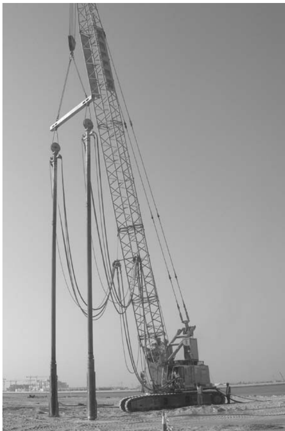
Figure 3.38 Vibro compaction equipment set up for S700 twin vibrator operation (by courtesy of Keller Group plc)
