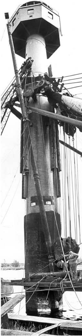
Figure 2.7 Lighthouse Tegeler Plate being set up to be vibrated into the seabed
