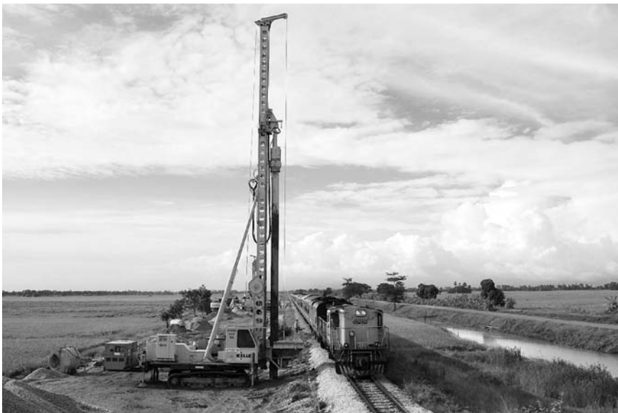
Figure 4.38 Vibrocat in operation next to existing railway track (by courtesy of Keller Group plc)
