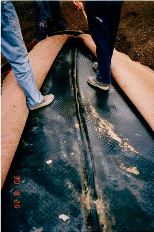
Fig. 9.7. Steep wave pushed together during backfilling. Excessive deformations may arise in the range of such waves. Courtesy Schicketanz Consulting Engineers, Aachen
