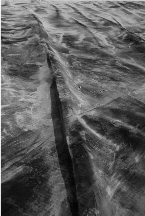
Fig. 9.6. Trial pitting of a composite liner after drainage layer installation showing that the geomembrane has been placed and ballasted without ensuring flatness. The waves have not been smoothed out by the load. Courtesy Schicketanz Consulting Engineers, Aachen
