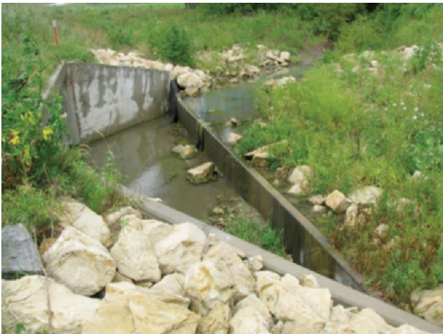
Figure 2.7 Inlet End of Reinforced Concrete Box With Soil Saver.
