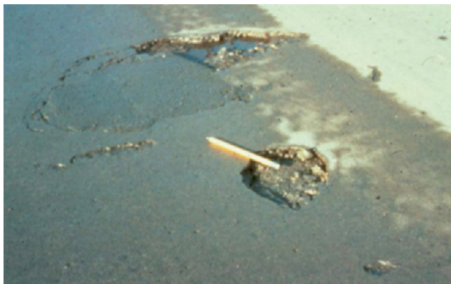
Figure 2.69 Concrete Spall. (Adapted from FHWA Bridge Inspectors Reference Manual [7]).
