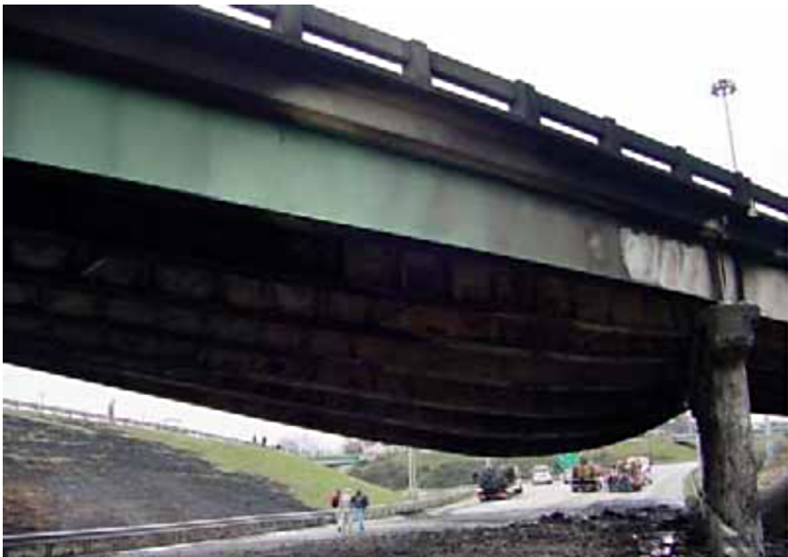
Figure 5.25 Fire Damaged Steel Girders. (Adapted from Federal Highway Administration. Bridge Inspector's Reference Manual . FHWA-NHI 12-049. Washington, DC; US Department of Transportation; 2012).
