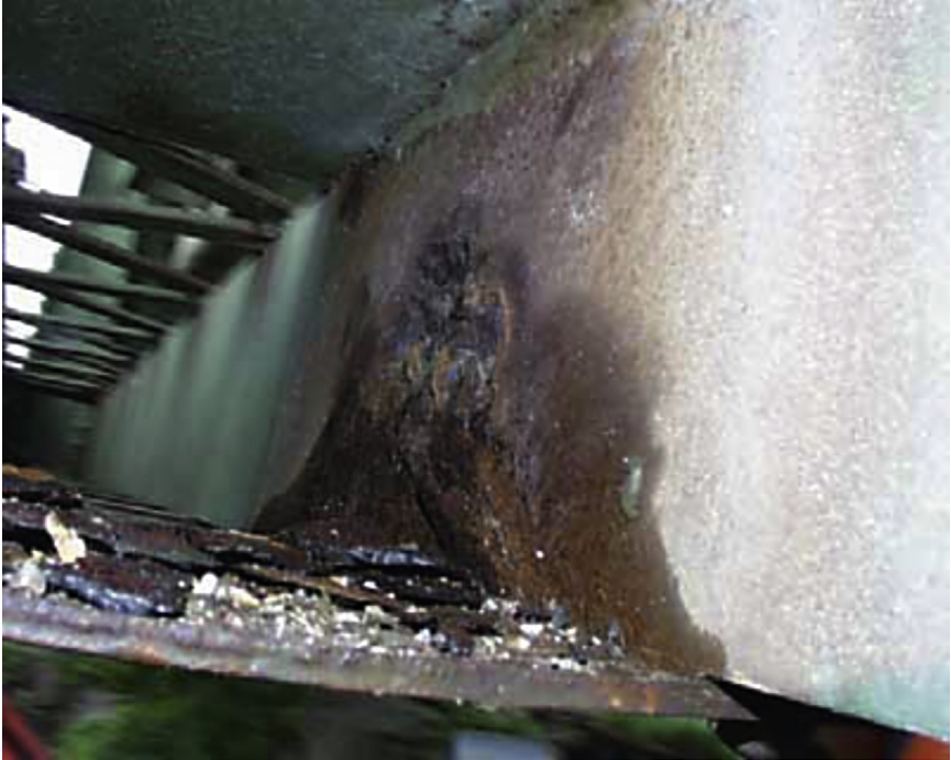
Figure 5.19 Section Loss Inside of Truss Chord.
