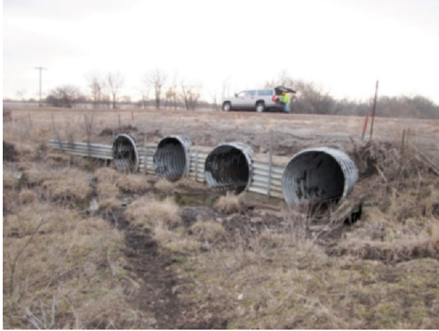
Figure 2.4 Multiple Corrugate Metal Pipes.
