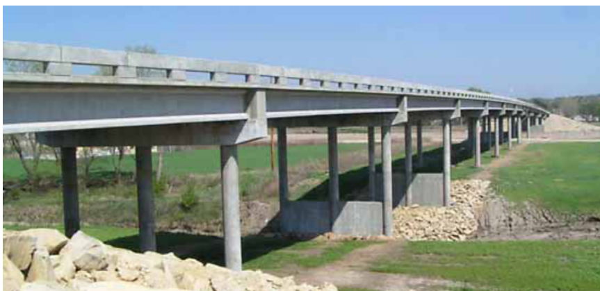
Figure 4.16 Use of Stone as Revetment at Berms and Scour Protection at Piers.
