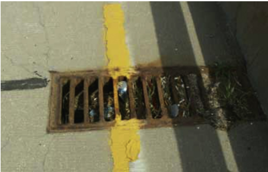
Figure 4.2 Plugged Deck Drain.
