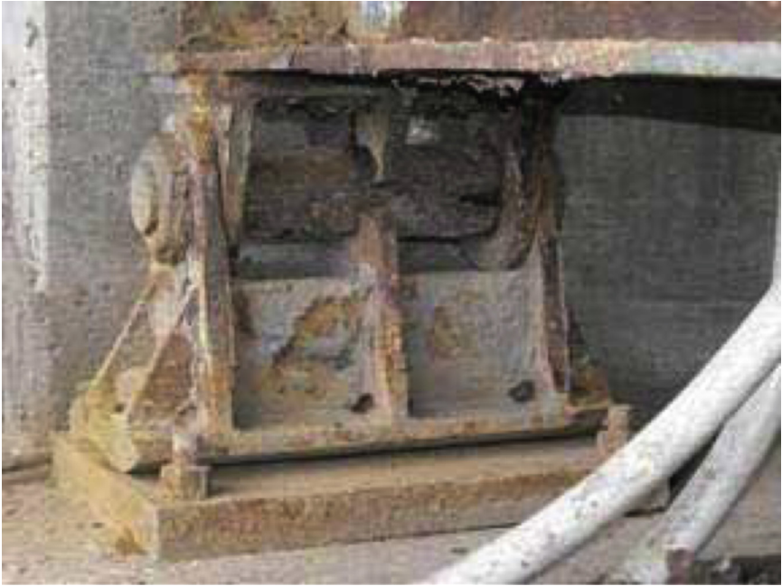
Figure 5.44 Deteriorated Steel Rocker Bearing.
