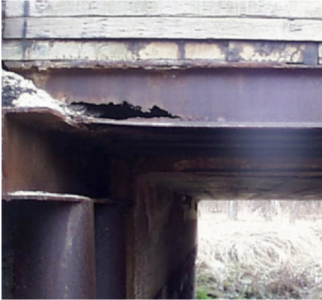
Figure 2.76 Corrosion Through Web of Steel Beam.
