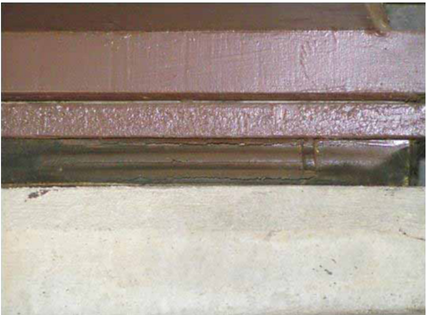
Figure 5.45 Splitting of Reinforced Elastomeric Bearing.
