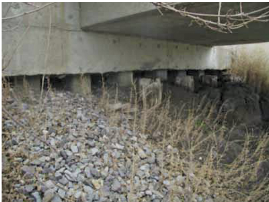
Figure 4.15 Erosion Under Abutment.
