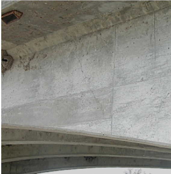
Figure 2.64 Typical 45° Shear Crack in Concrete Girder.
