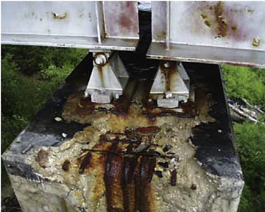
Figure 4.11 Failed Waterproofing Member and Bearing Area Deterioration.
