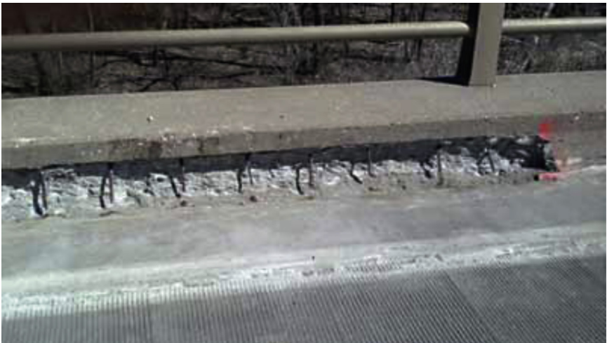
Figure 6.10 Deteriorated Reinforcing Steel in Parapet (KDOT).
