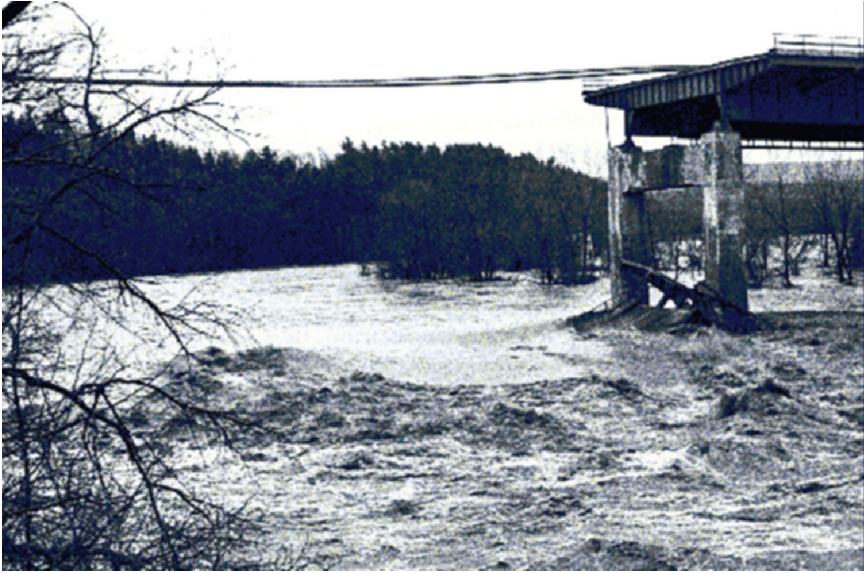
Figure 1.13 Collapse of NY State Thruway Over Schoharie. (From FHWA Underwater Inspection Manual [16]).
