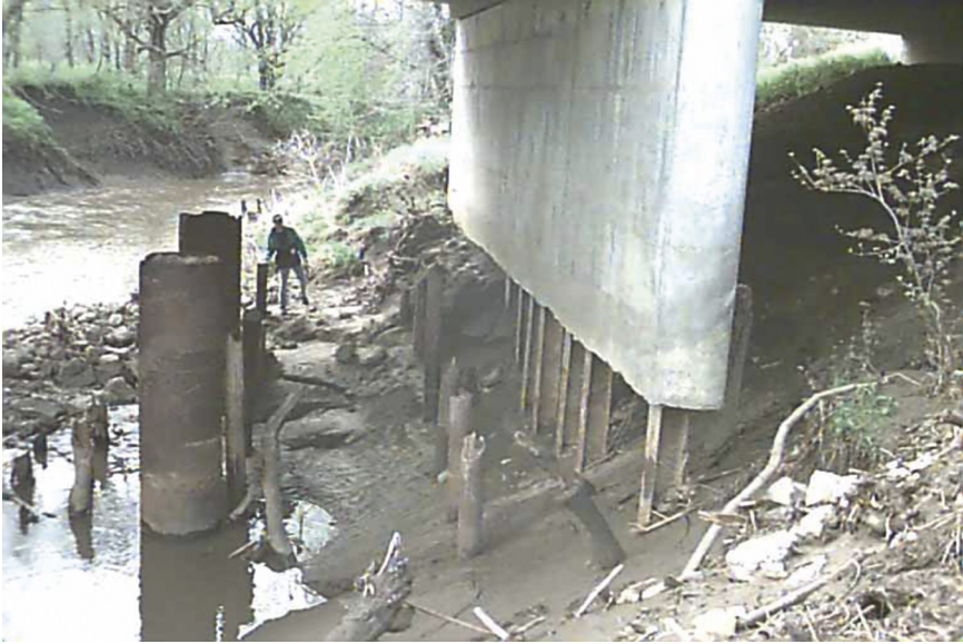
Figure 4.13 Scour at Pier Wall.
