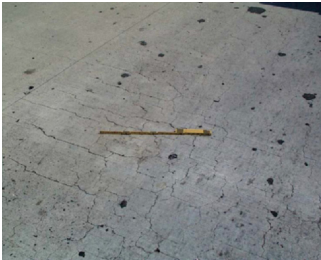
Figure 2.66 Shrinkage Cracks. (Adapted from FHWA Bridge Inspectors Reference Manual [7]).
