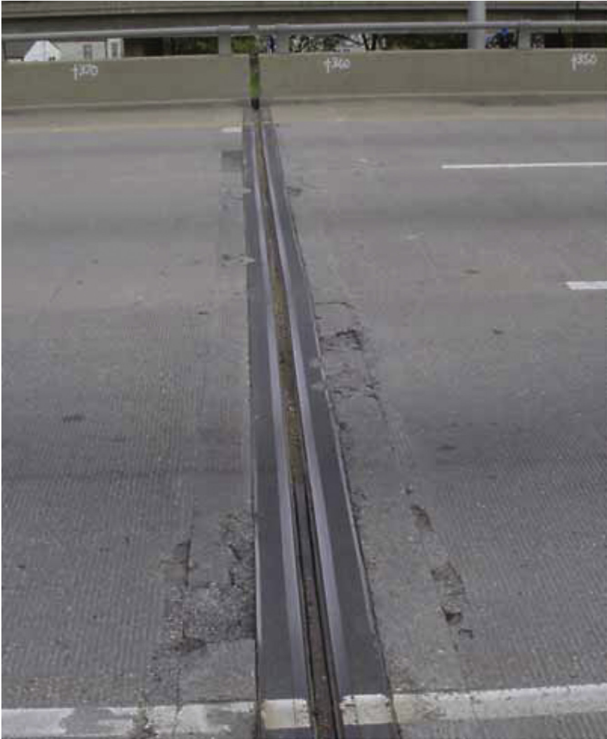
Figure 4.6 Deck Deterioration at Expansion Joint.
