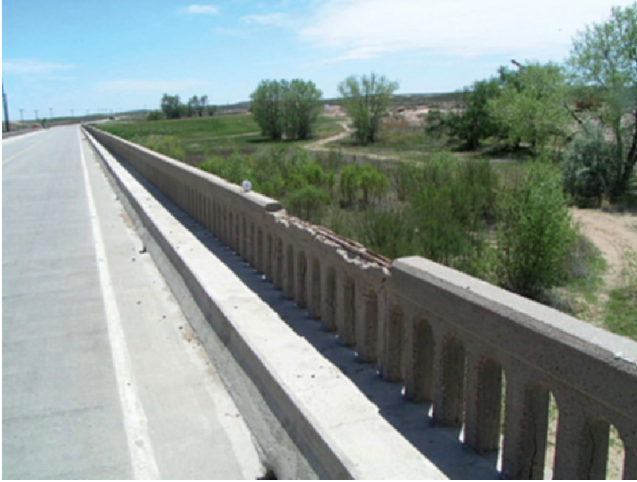
Figure 2.27 Damaged Type A Rail.
