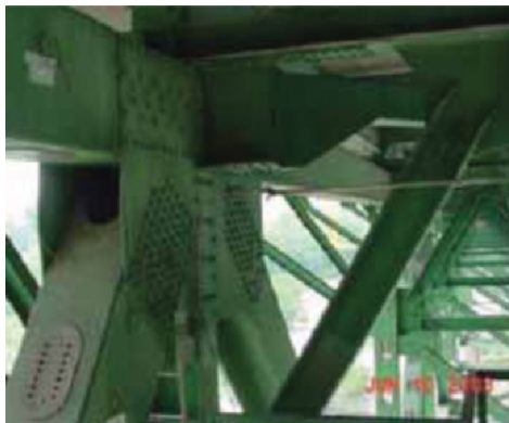
Figure 1.18 Connections at Node U10 West. (From 2008 NTSB Report [17]).
