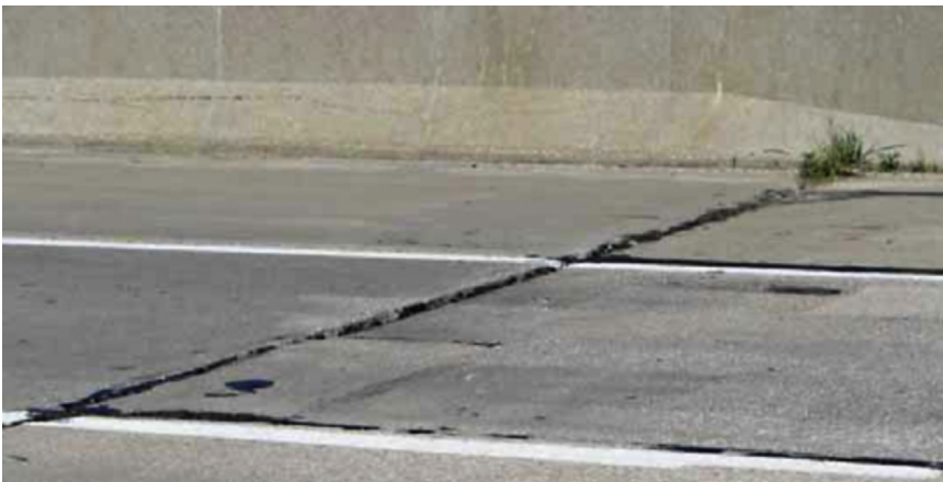
Figure 4.17 Settlement of Approach Slab.
