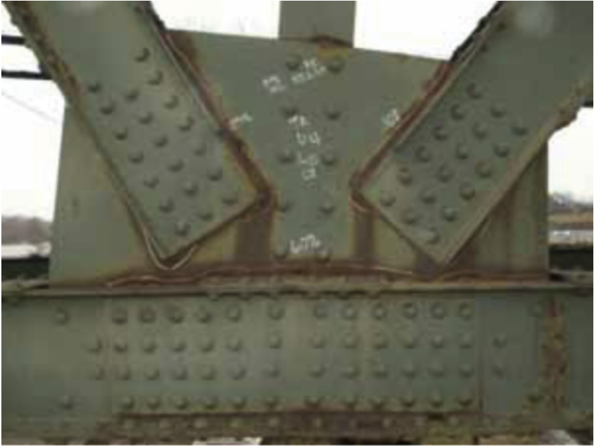
Figure 5.48 Deteriorated Gusset Plate on Steel Truss Bridge.
