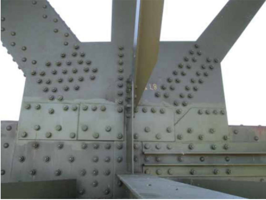
Figure 1.21 Typical Gusset Plate Repair.
